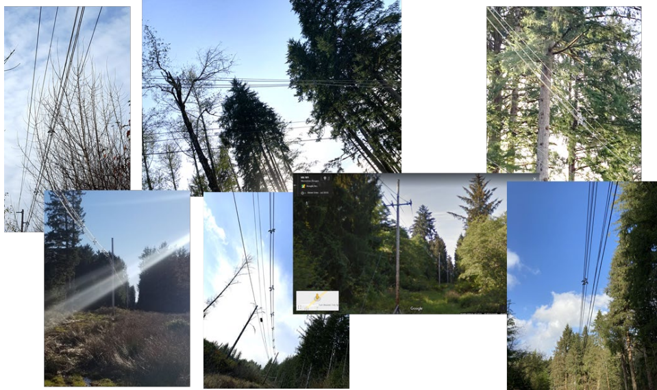
Figure 5 PacifiCorp Covered Conductor Effectiveness Examples
