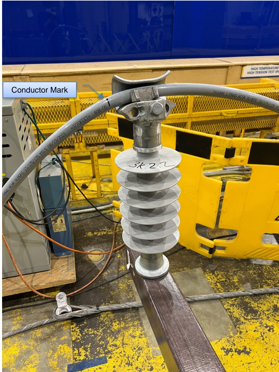
Figure 6-32: Sample 3K.2.2 – Insulator and Cross-arm Condition after Test
