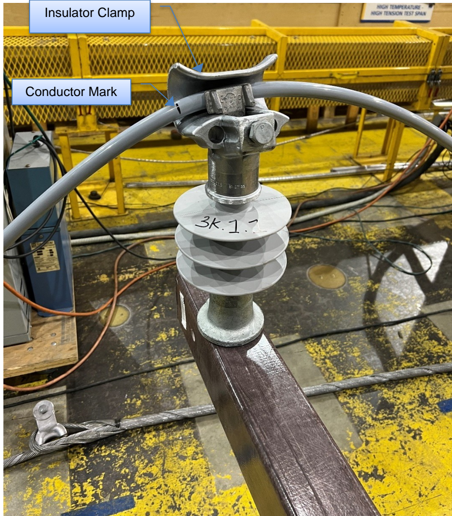
Figure 6-25: Sample 3K.1.1 – Insulator and Cross-arm Condition after Test
