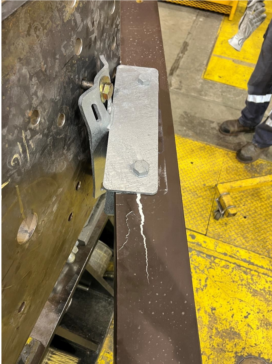
Figure 6-17: Sample 4.1 – Failure Location
