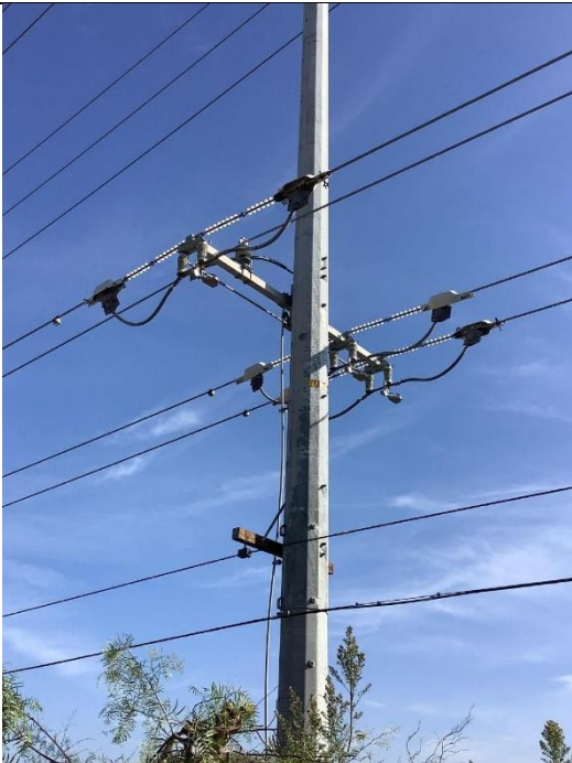
Item13IA1img1: No vibration dampers installed
