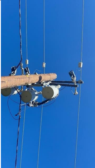
Item16IA1Img1: No vibration dampers installed
