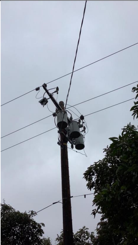
Item3IA1Img1: No vibration dampers are installed
