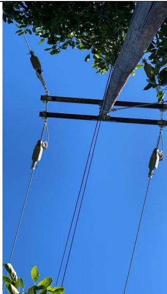
Item10IA1Img1: Vibration dampers not installed
