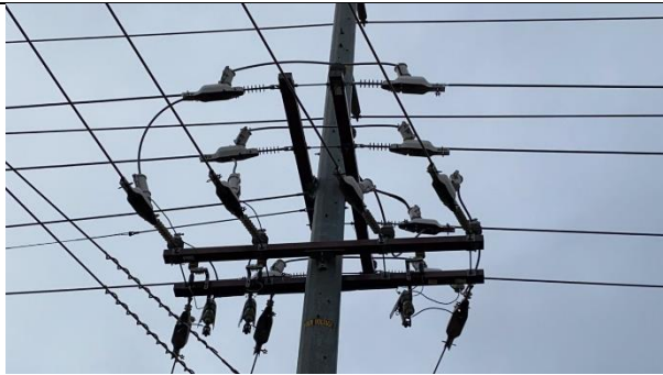
Item16IA2img1: No vibration dampers
