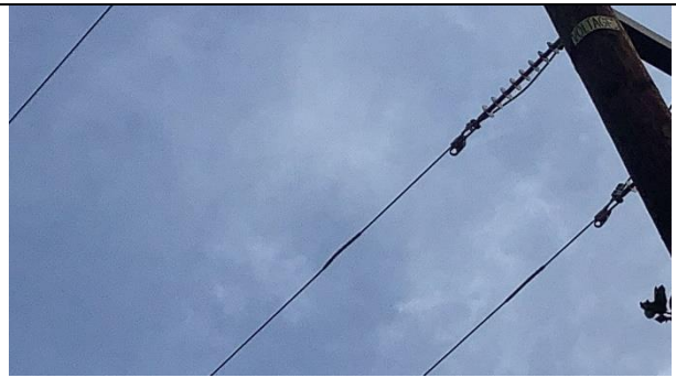
Item1IA1Img2: Close up of bare wire
