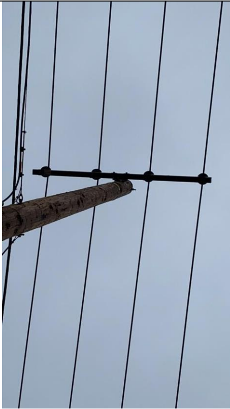
Item11IA1mg1: No vibration dampers
