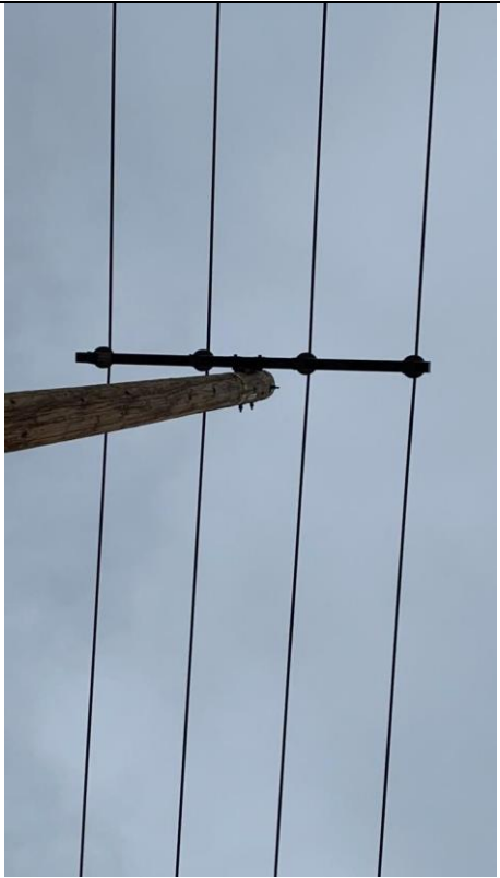
Item10IA1mg1: No vibration dampers
