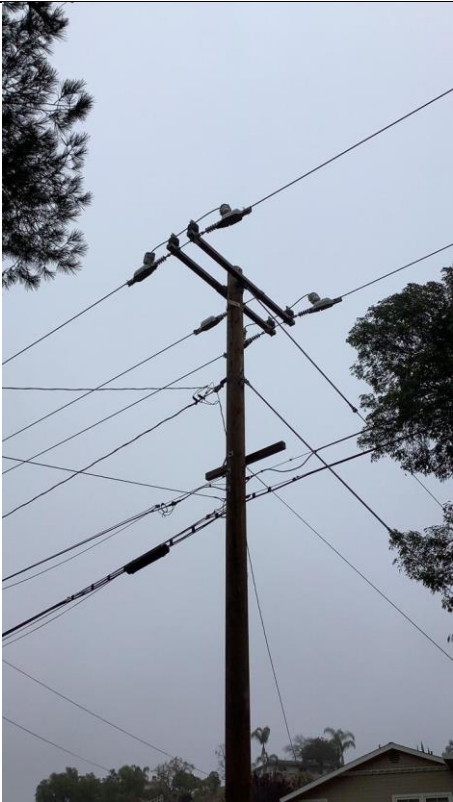
Item3IA1Img1: No vibration dampers are installed
