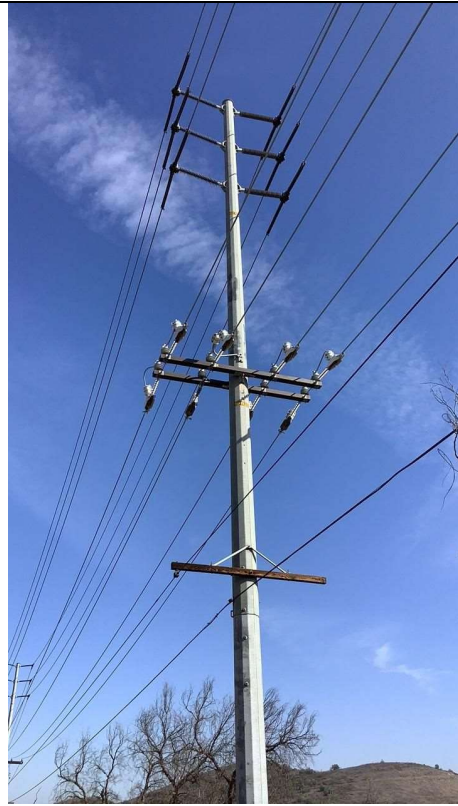
Item8GImg2: Overall view of the pole and covered conductor
