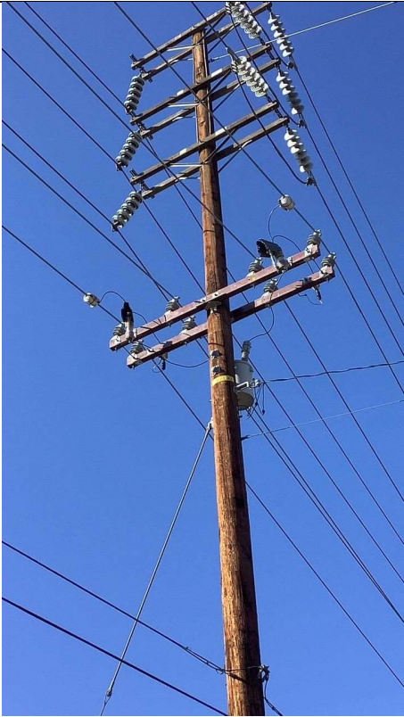
Item2IA1Img1: No vibration dampers are installed
