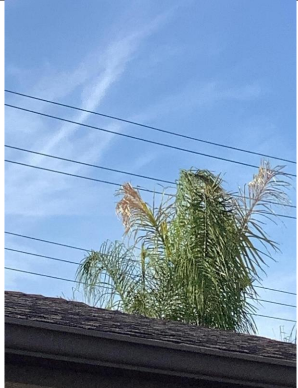
Item9IA1Img4: Palm fronds contacting conductors
