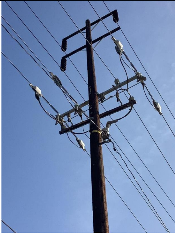
Item11IA1img1: Vibration dampers are missing
