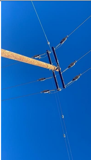
Item9IA2Img1: Three guy wires with porcelain insulators
