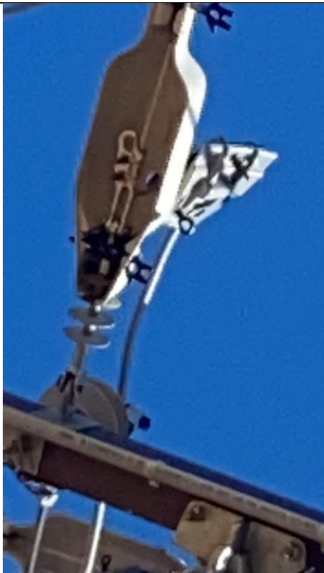
Item16IA2Img1: Loose center phase bolted wedge connector
