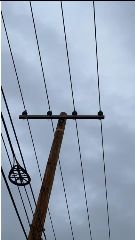
Item9IA1Img1: No vibration dampers
