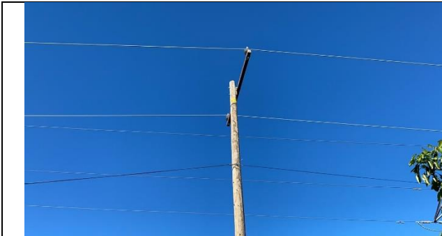
Item9IA1img1: Vibration dampers not installed
