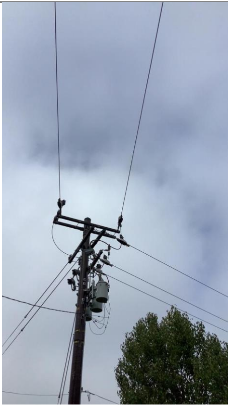
Item1IA1Img1: No vibration dampers are installed
