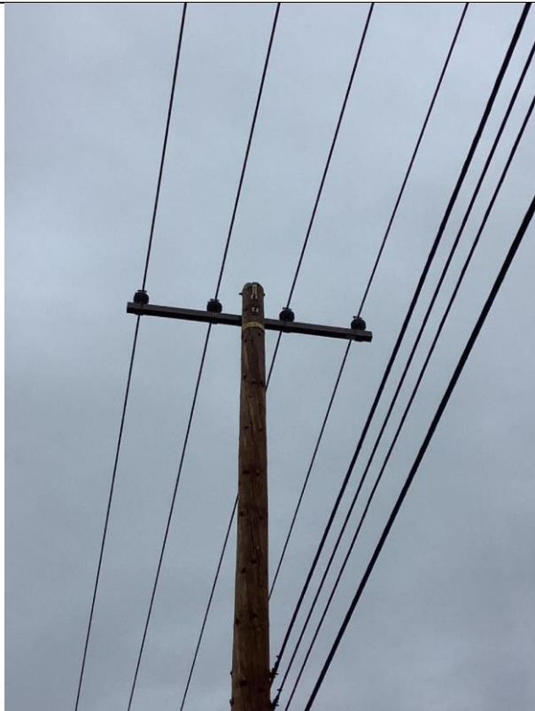
Item9IA1Img1: No vibration dampers installed
