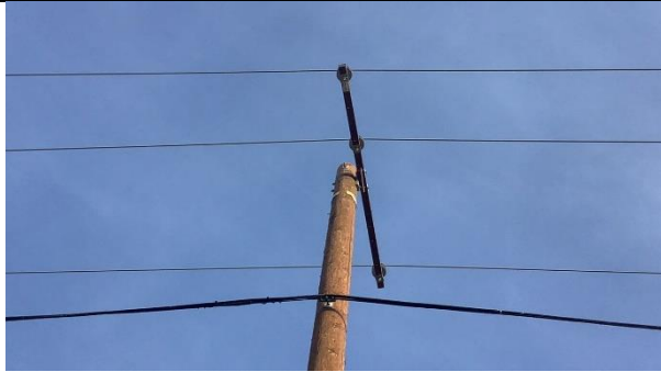
Item10IA1Img1: No vibration dampers installed
