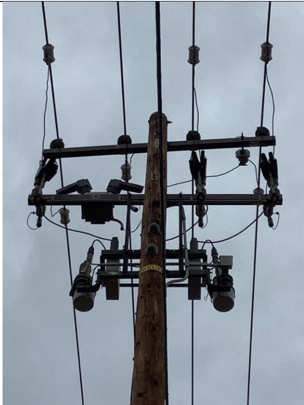
Item13IA1mg1: No vibration dampers installed
