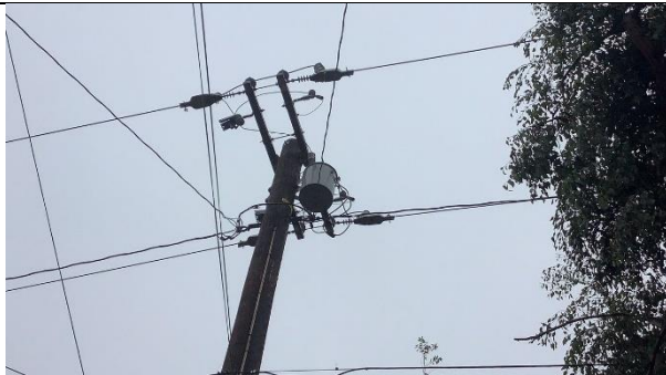
Item4IA1Img1: Vibration dampers not installed
