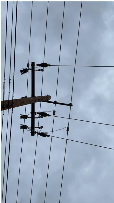
Item12IA1Img1: No vibration dampers
