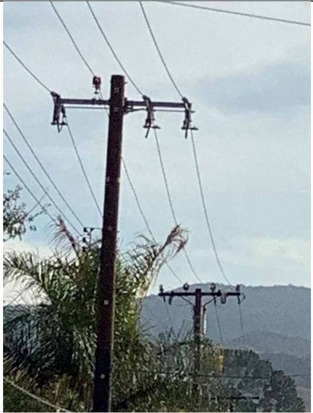
Item9IA1Img2: Palm fronds contacting the conductor.
