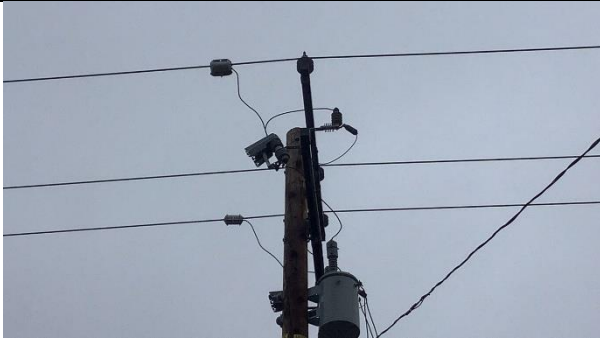
Item2IA1Img1: Vibration dampers not installed
