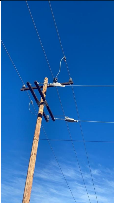
Item8IA1Img1: No vibration dampers
