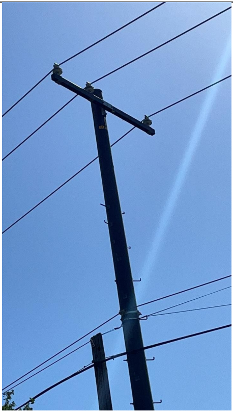
Item1IA1Img1: Missing vibration dampers
