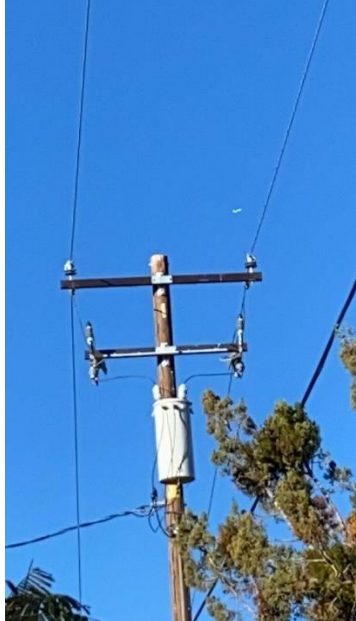
Item4IA1img1: Vibration dampers not installed
