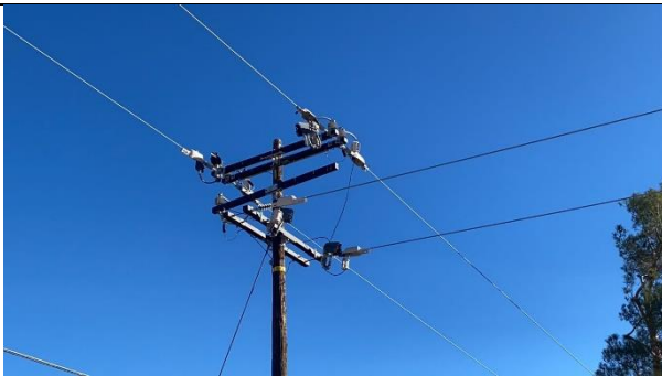
Item6IA1Img1: No vibration dampers
