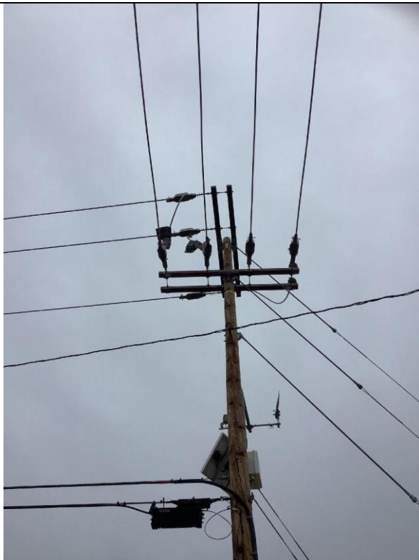
Item15IA1img1: No vibration dampers installed
