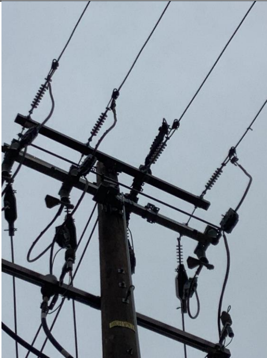
Item16IA2Img1: Bolted wedge connector cover not installed
