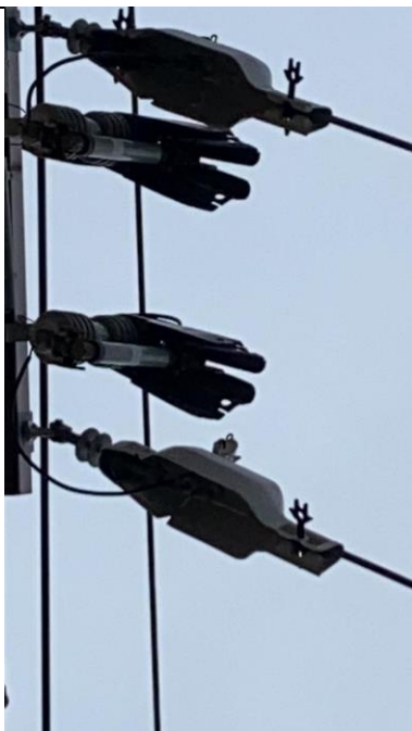
Item16IA4Img1: Loose dead-end clamp
