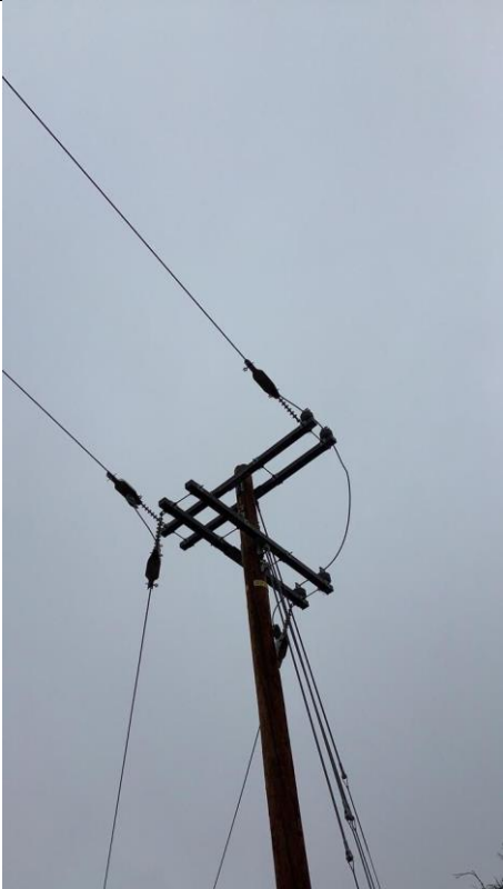
Item2IA1Img1: No vibration dampers are installed
