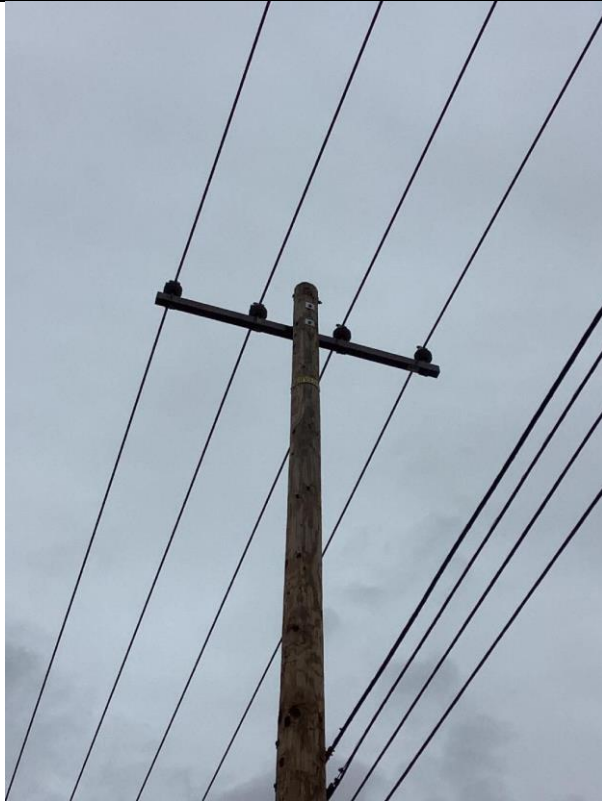
Item12IA1Img1: No vibration dampers installed
