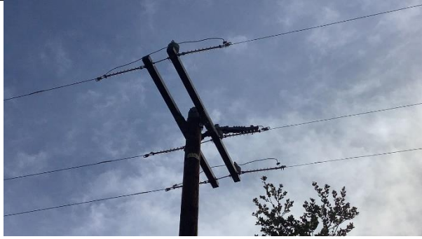
Item1IA1img1: No covered conductor
