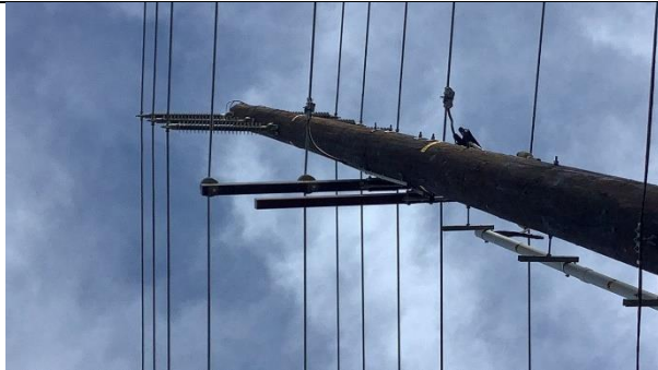
Item5IA1Img1: Vibration dampers not installed
