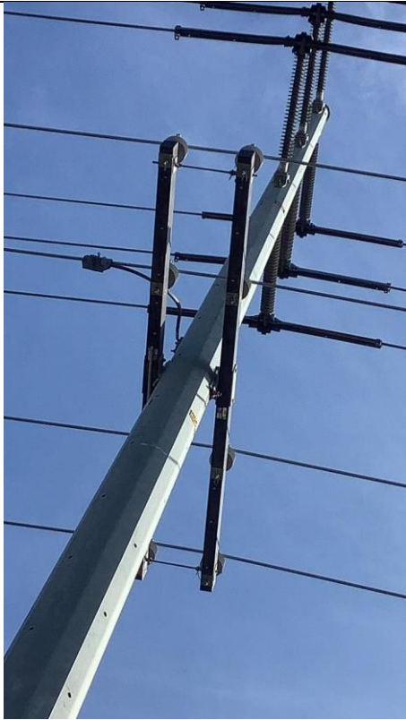
Item10IA1mg1: Vibration dampers not installed
