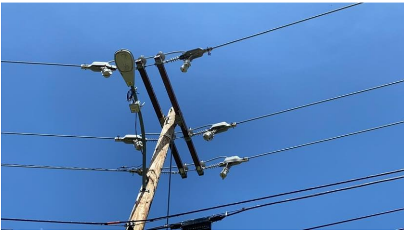
Item10IA2Img1: No vibration dampers
