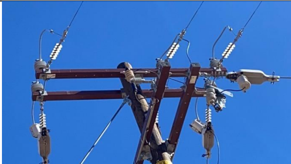
Item15IA2Img2: Bare to dead end with no bolted wedge connector covers
