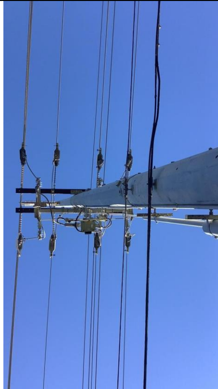
Item1IA1img2: Showing where covered conductor ends and bare conductor begins
