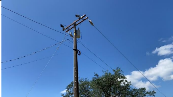
Item3IA1Img1: No vibration dampers
