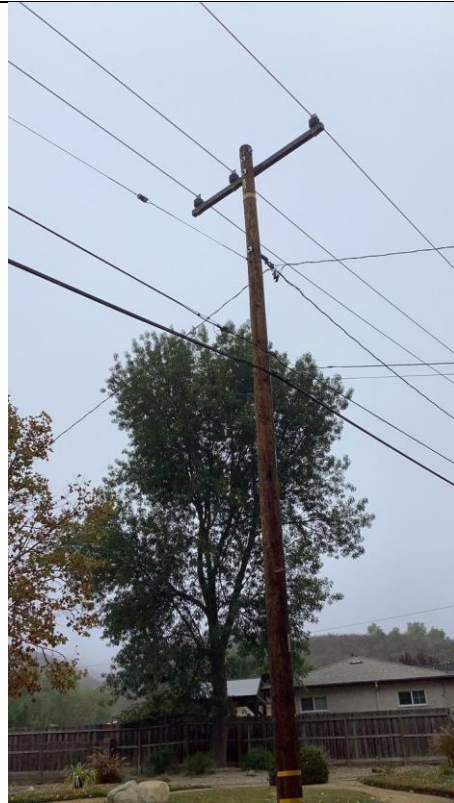
Item2Gimg2: Overall view of the pole and covered conductor
