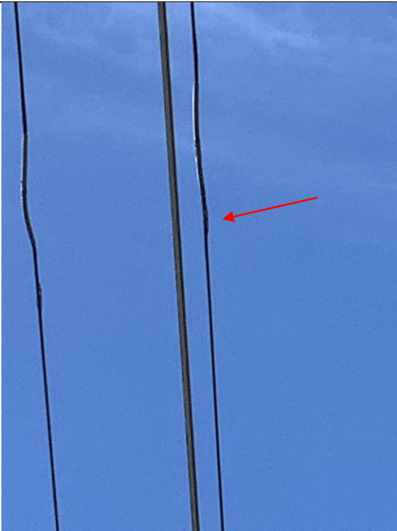
Item4CD5Img3: Bird-Caging middle conductor near pole X11580E
