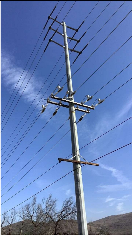
Item8IA1Img1: No vibration dampers are installed
