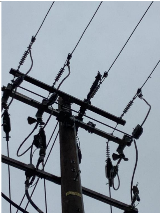
Item16IA2Img1: Bolted wedge connector cover not installed
