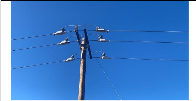
Item13IA1Img1: No vibration dampers
