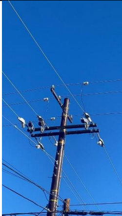
Item14IA1img1: Vibration dampers not installed
