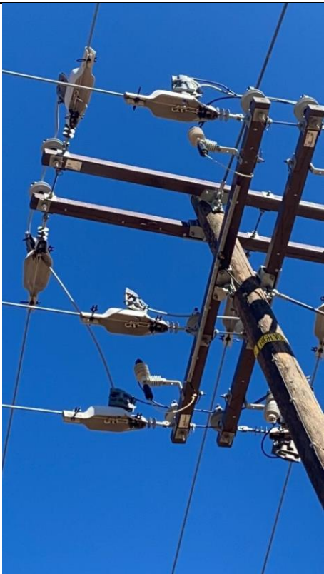
Item16IA2Img2: Overall loose center phase bolted wedge connector
