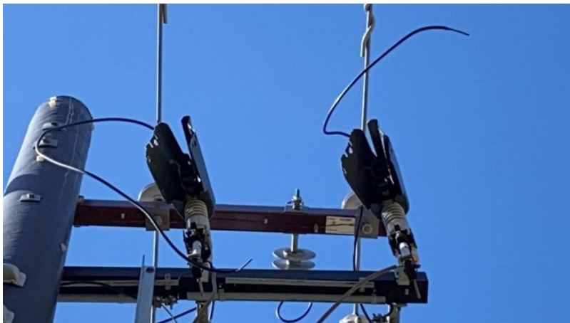
Item3IA1Img3: Observation, 3 Fuses are popped with jumpers hanging in air
