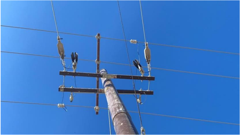
Item13IA1img1: No vibration dampers
