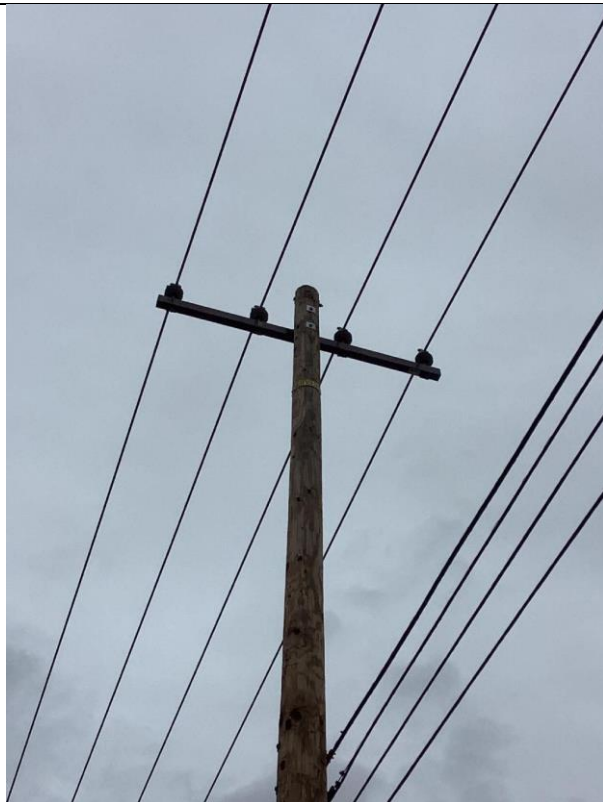
Item12IA1Img1: No vibration dampers installed
