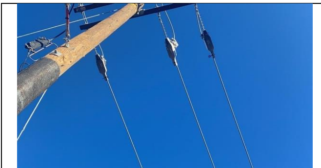
Item3IA1Img1: No vibration dampers
