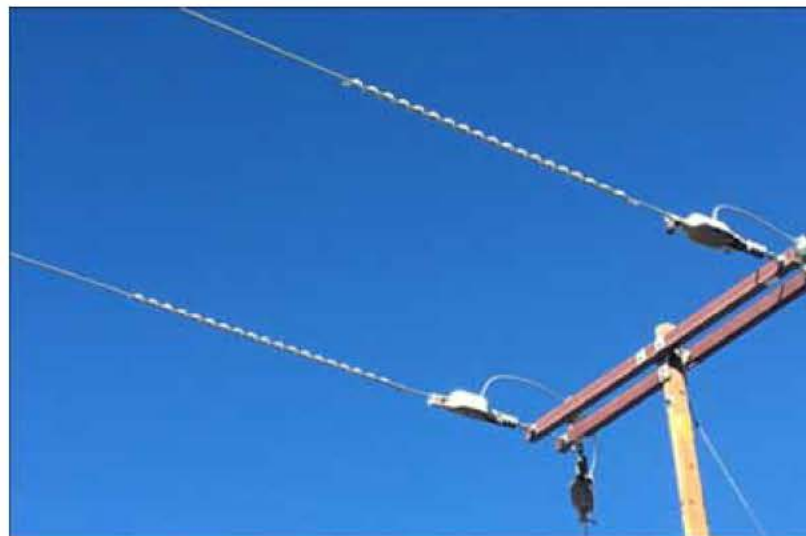
Figure CC 190–4: Installed Spiral Vibration Dampers on Covered Conductor
