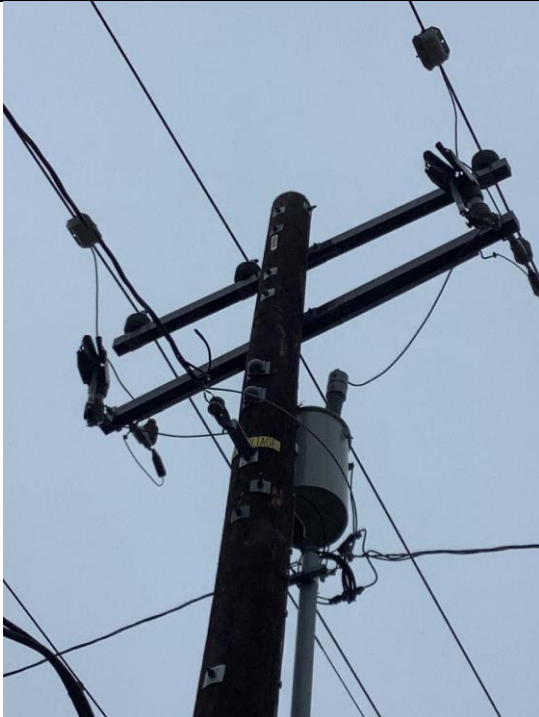
Item2IA1Img1: Vibration dampers are missing
