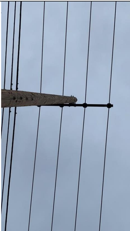
Item8IA1Img1: No vibration dampers
