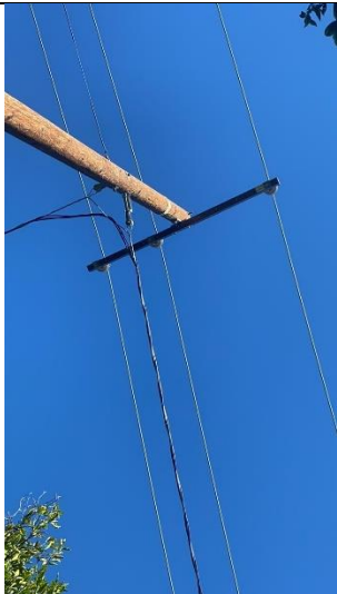
Item15IA1img1: Vibration dampers not installed
