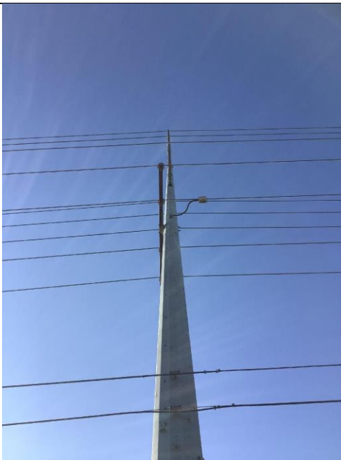
Item2IA1Img1: No vibration dampers installed
