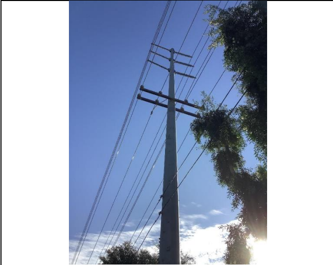
Item1IA1mg1: No vibration dampers installed
