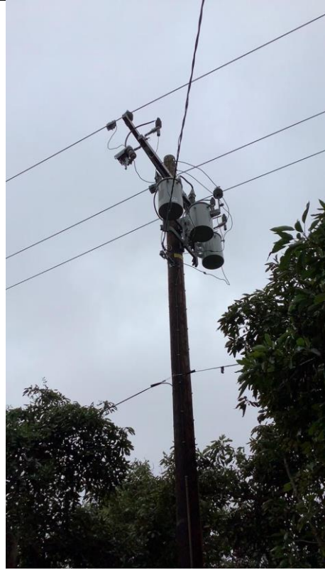
Item3GImg2: Overall view of the pole and covered conductor
