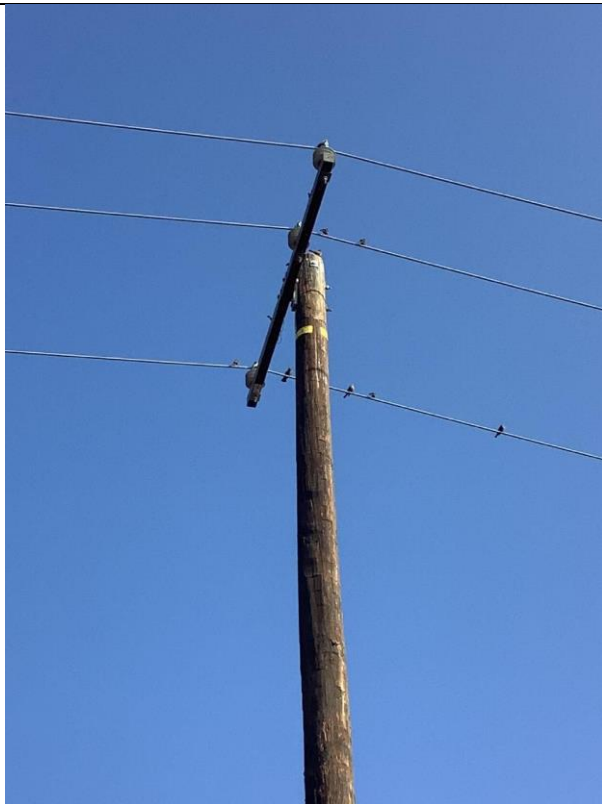
Item10IA1mg1: Vibration dampers are missing
