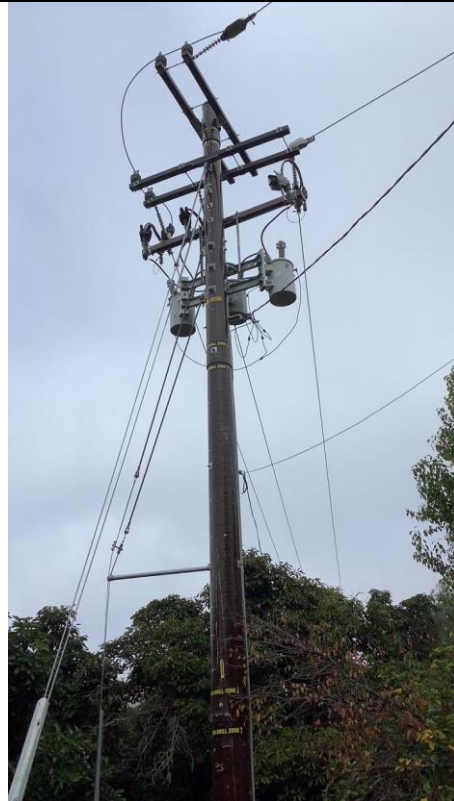
Item1GImg2: Overall view of the pole and covered conductor
