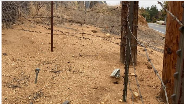
Item12IA3Img1: Abandoned guy anchor
