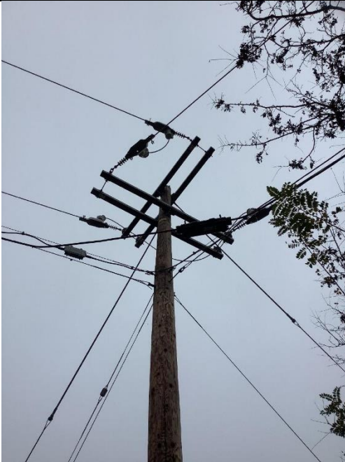
Item4IA1Img1: Vibration dampers are missing
