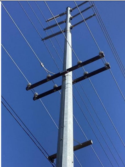
Item7IA1Img1: Vibration dampers not installed
