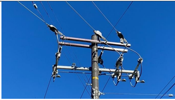
Item6IA2Img1: Vibration dampers not installed
