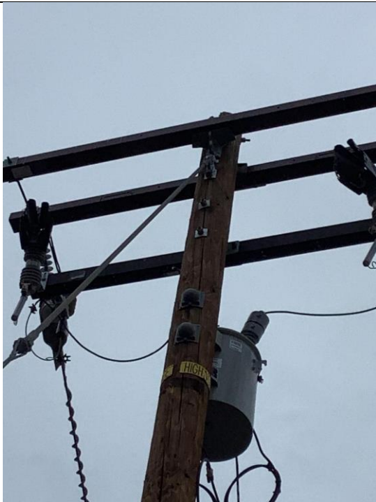
Item4IA1img1: Surge arrester clamp not covered
