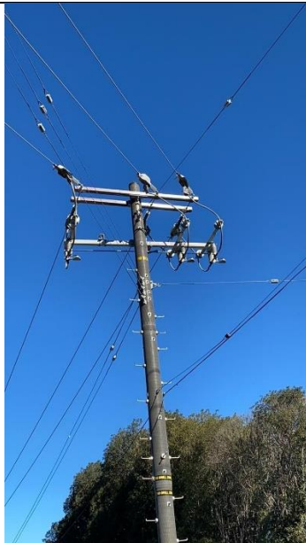
Item6IA1Img1: Overall of 6 guy spans with porcelain insulators
