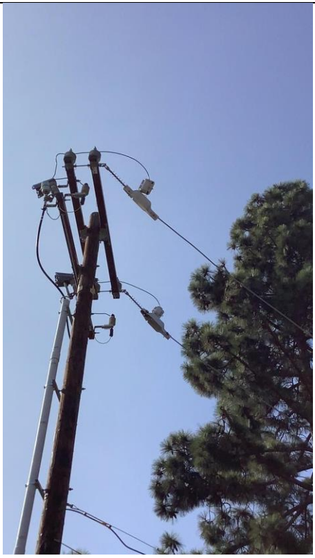
Item3IA1Img1: No vibration dampers are installed
