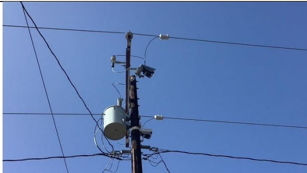
Item11IA1img1: Vibration dampers not installed
