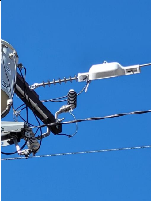
Item1IA3Img1: Missing bolted wedge connector cover
