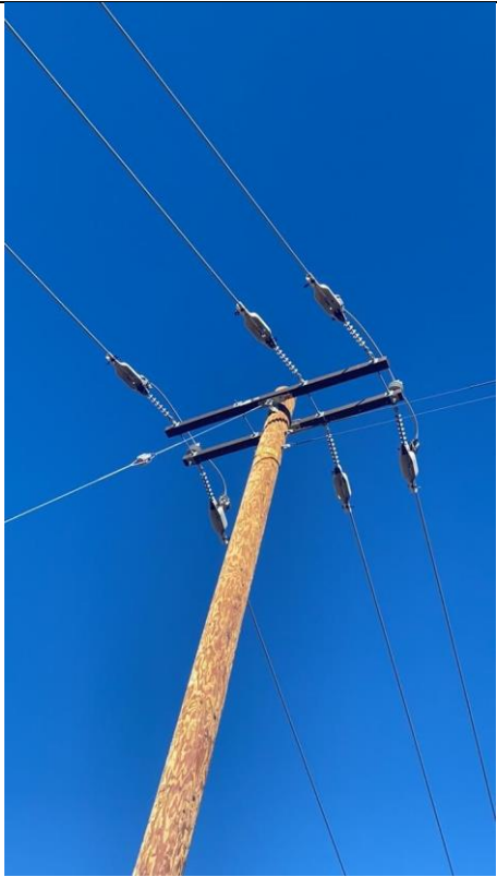
Item9IA1Img1: No vibration dampers
