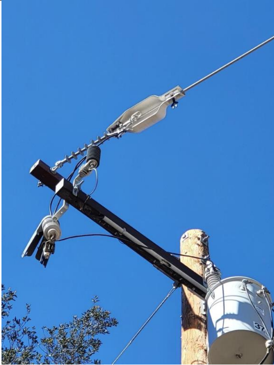
Item1IA2Img1: Missing vibration dampers
