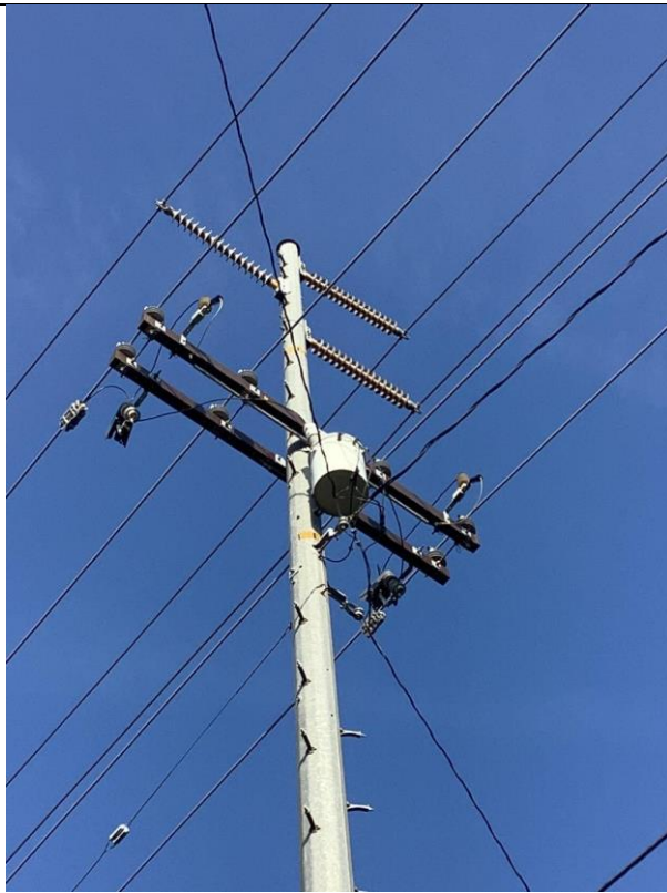
Item12IA1mg1: Vibration dampers are missing
