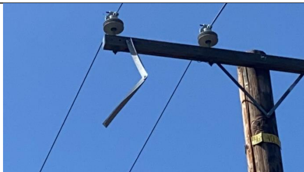
Item11CA2Img1: Wildlife Mitigation device falling off crossarm
