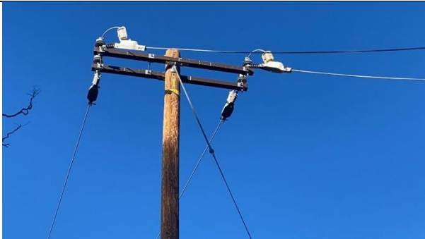
Item2IA1Img1: No vibration dampers
