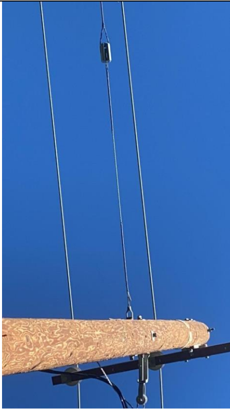
Item15IA2Img1: : Fiberglass span guy wire insulator not installed
