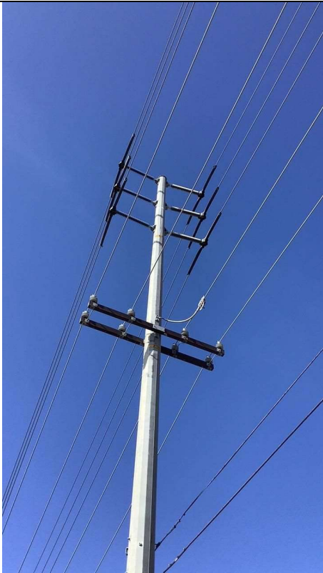
Item4IA1img1: Steel pole observed in the field and no vibration dampers installed
