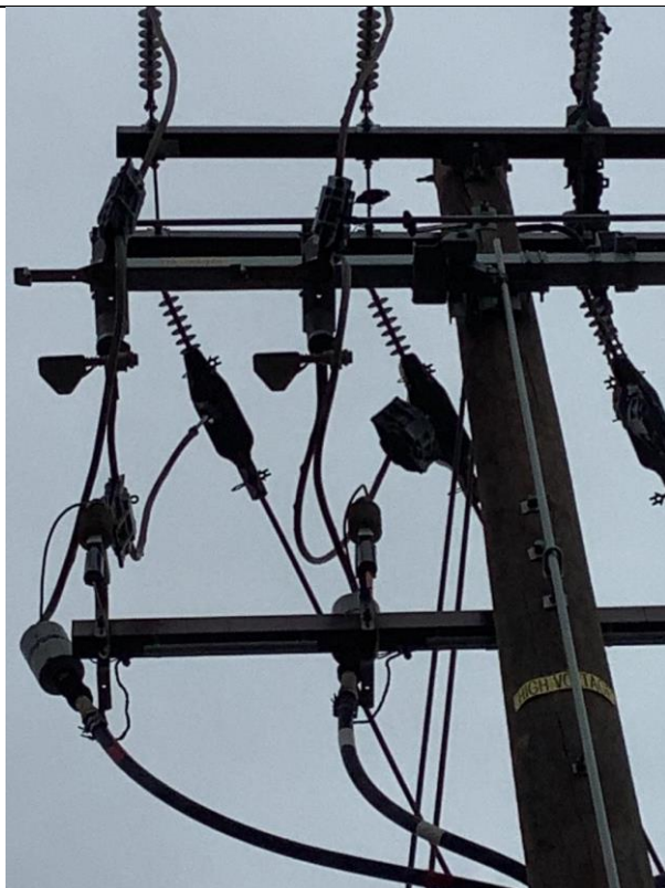
Item16IA3Img1: No cover on jumper wire
