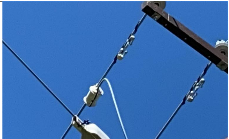
Item4IA1Img2: Observation: Close up showing vibration dampers on upper pole phase level between jumper and crossarms
