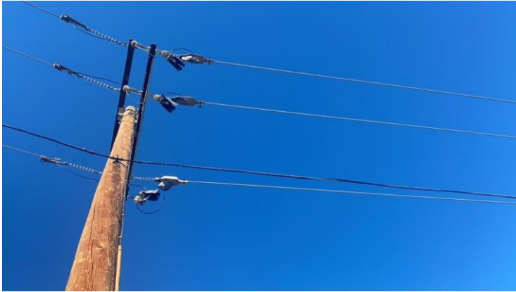
Item2IA1Img1: No vibration dampers
