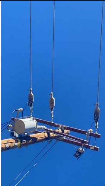
Item14IA1img1: No vibration dampers
