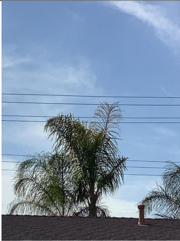
Item9IA1Img1: Palm fronds contacting the conductor.
