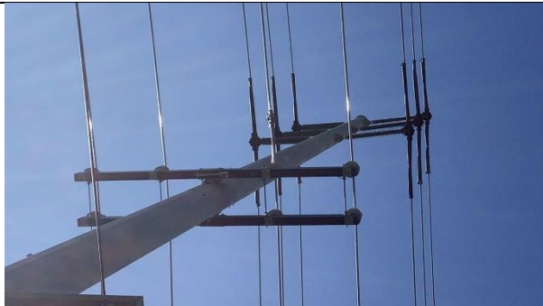
Item4IA1Img1: No vibration dampers installed
