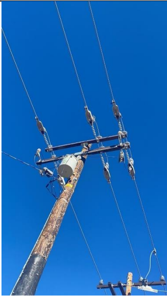
Item7IA1Img1: No vibration dampers
