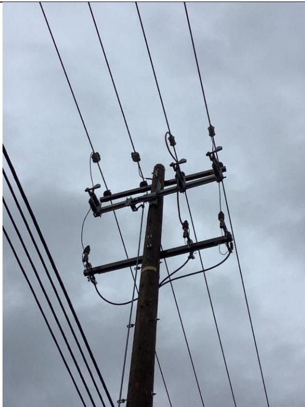
Item11IA1mg1: No vibration dampers installed
