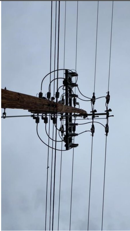
Item13IA1Img1: No vibration dampers
