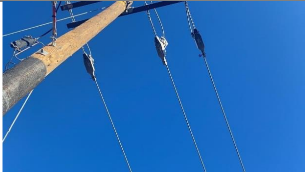
Item3IA1Img1: No vibration dampers
