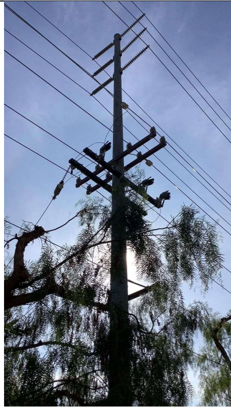
Item9GImg2: Overall view of the pole and covered conductor
