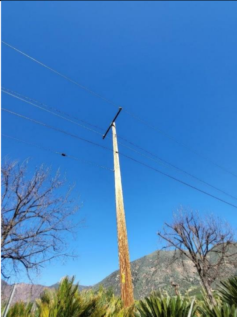
Item2IA1img1: Missing vibration dampers
