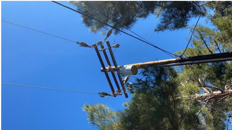
Item17IA1img1: No vibration dampers
