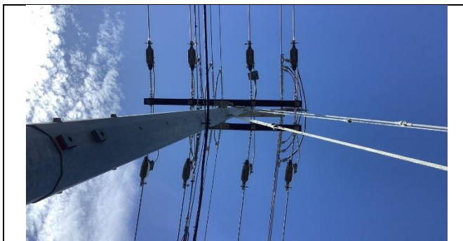
Item2IA1Img1: No vibration dampers installed
