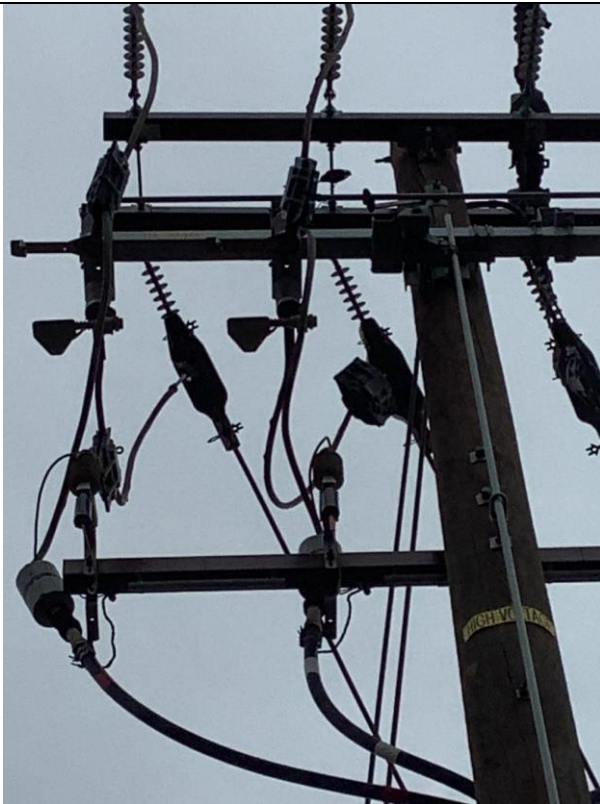
Item16IA3Img1: No cover on jumper wire
