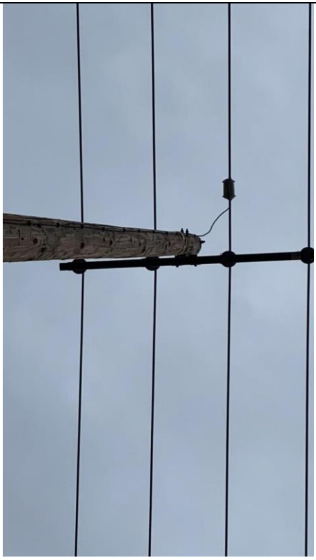
Item6IA1Img1: No vibration dampers
