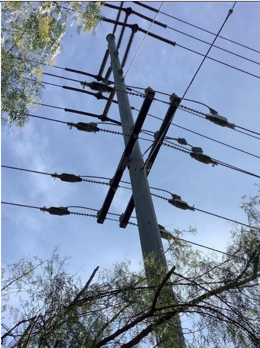
Item16IA1Img1: No vibration dampers installed
