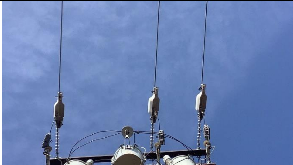
Item13IA1img1: Vibration dampers not installed
