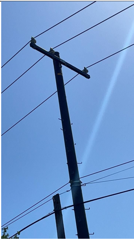
Item1IA1Img1: Missing vibration dampers
