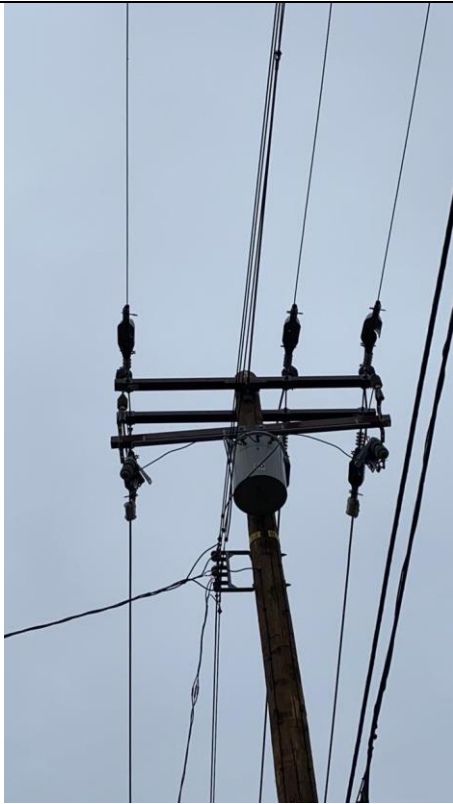
Item14IA1mg1: No vibration dampers
