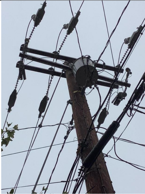
Item1IA1Img1: Vibration dampers are missing
