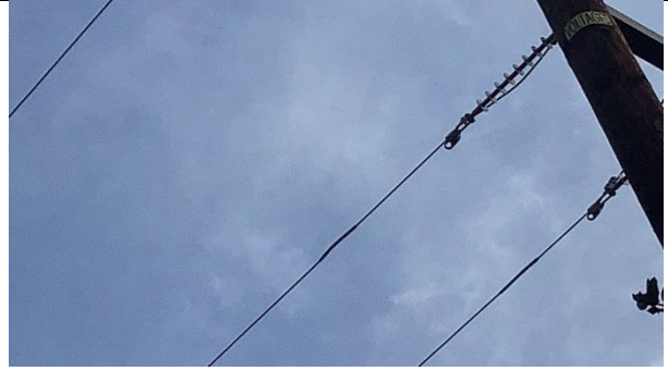
Item1IA1img2: Close up of bare wire
