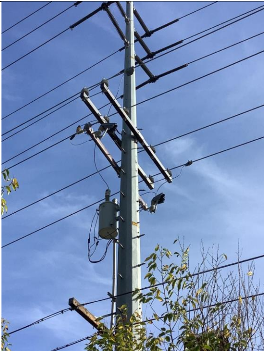
Item15IA1Img1: No vibration dampers installed
