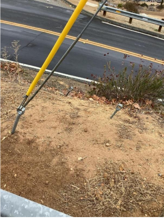
Item16IA4Img1: Guy anchors left in in the ground
