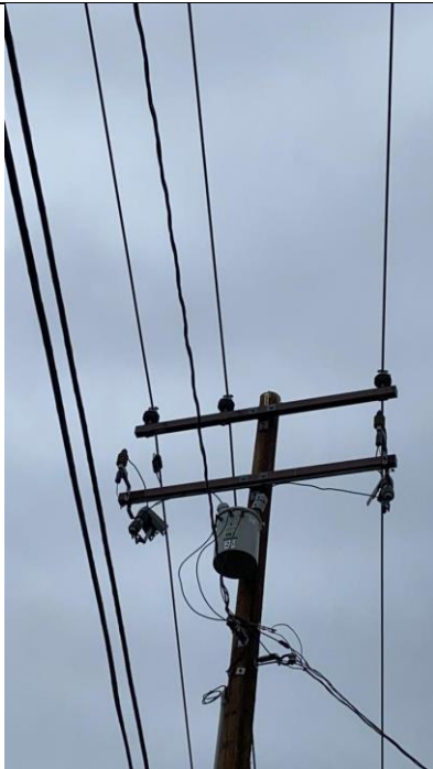
Item15IA1Img1: No vibration dampers
