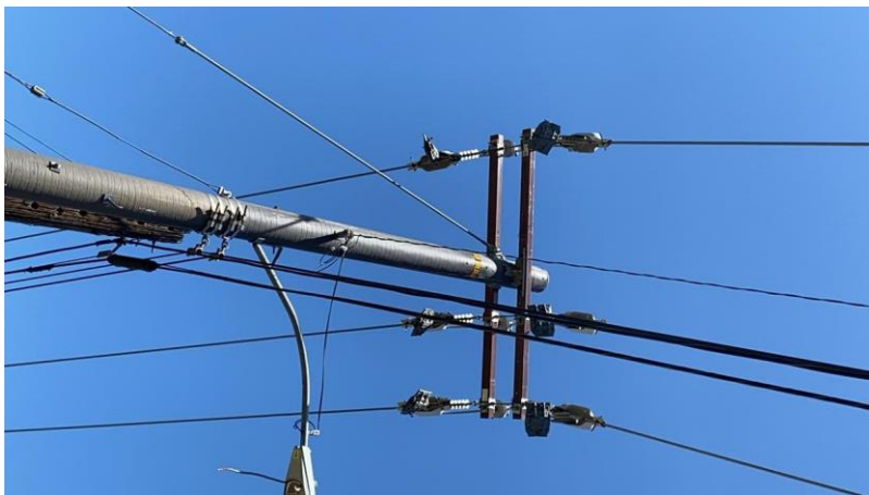
Item8IA1Img1: No vibration dampers
