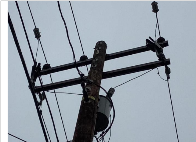
Item3IA1Img1: Vibration dampers are missing
