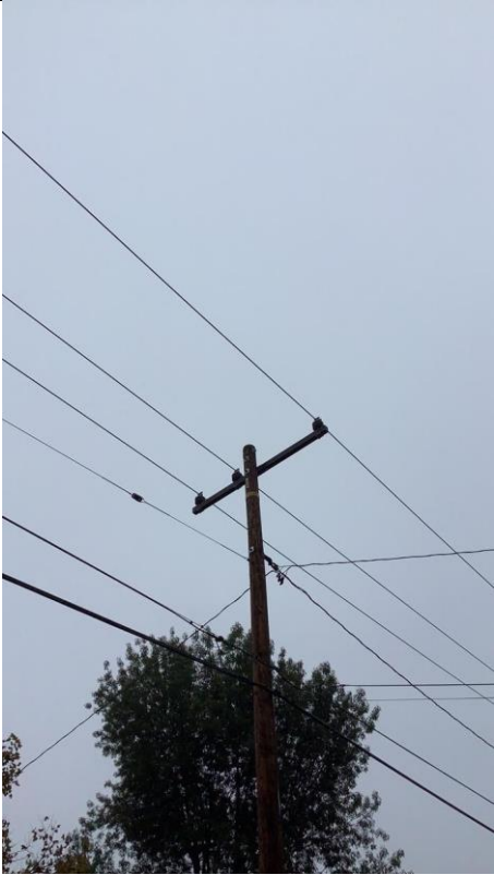
Item2IA1Img1: No vibration dampers are installed
