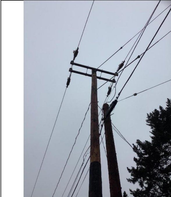
Item5IA1img1: Vibration dampers are missing
