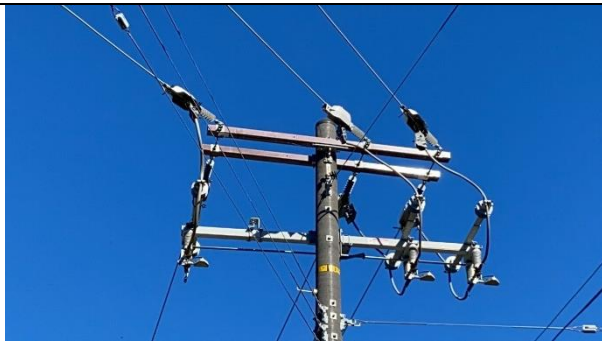
Item6IA2Img1: Vibration dampers not installed
