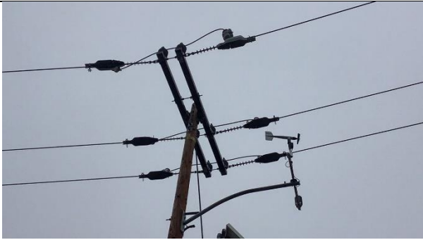
Item3IA2Img1: Vibration dampers not installed
