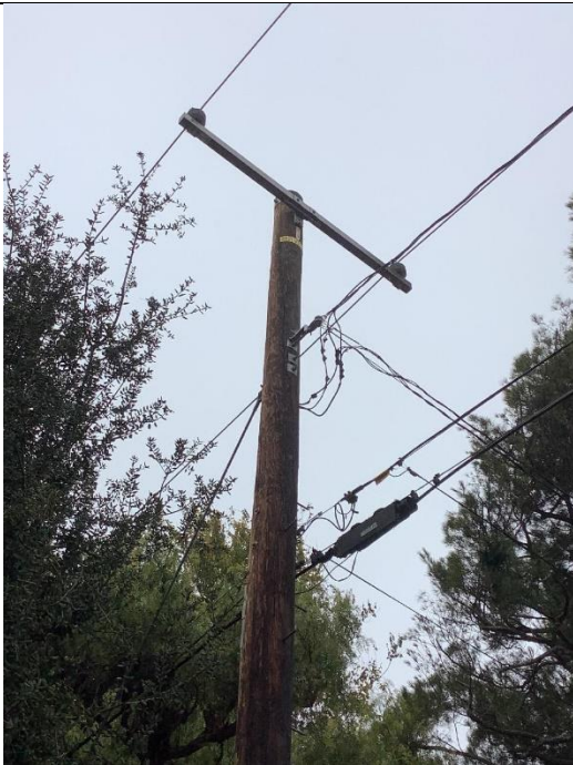
Item6IA1img1: Vibration dampers are missing
