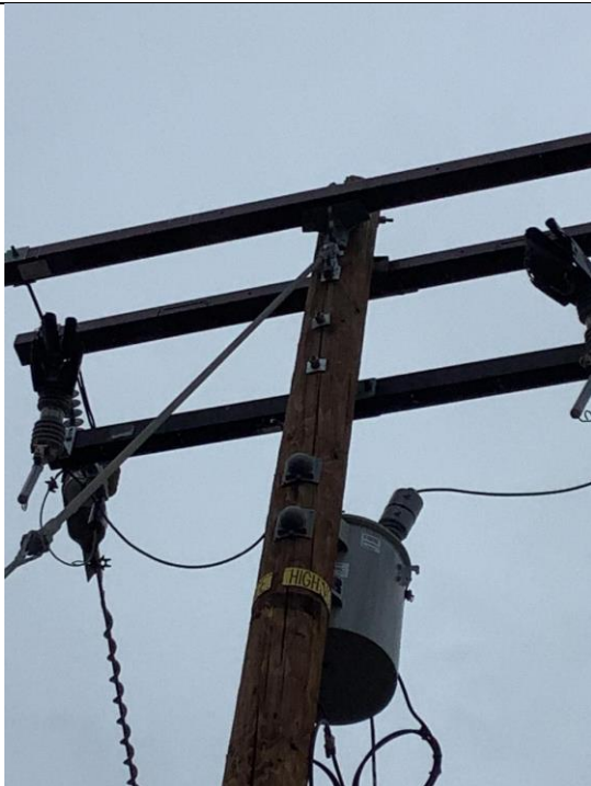
Item4IA1Img1: Surge arrester clamp not covered
