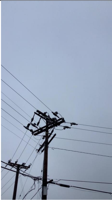
Item1IA1Img1: No vibration dampers are installed
