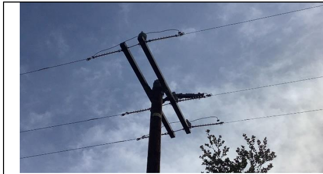
Item1IA1Img1: No covered conductor
