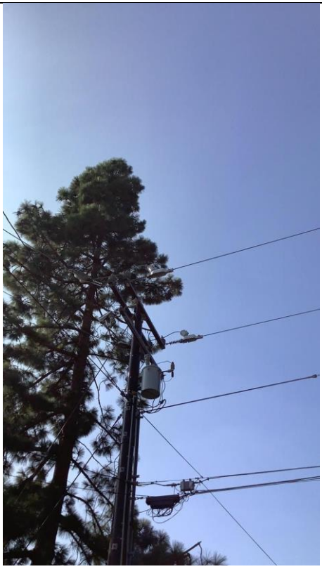
Item2IA1Img1: No vibration dampers are installed
