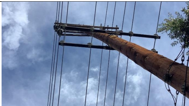
Item9IA1Img1: Vibration dampers not installed
