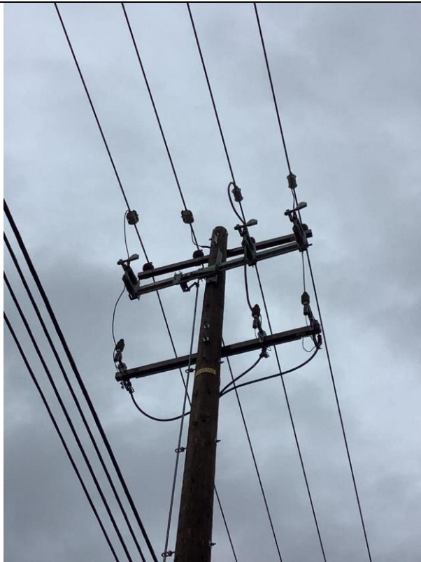
Item11IA1Img1: No vibration dampers installed
