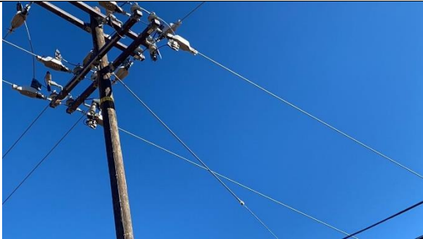
Item16IA1Img1: No vibration dampers
