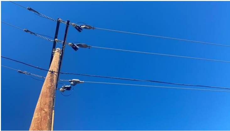
Item2IA1img1: No vibration dampers
