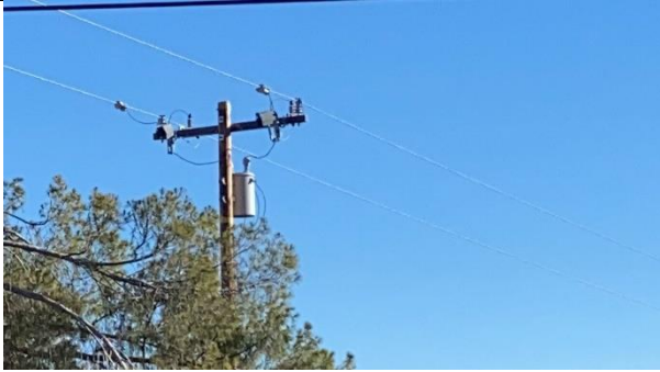
Item5IA1img1: No vibration dampers
