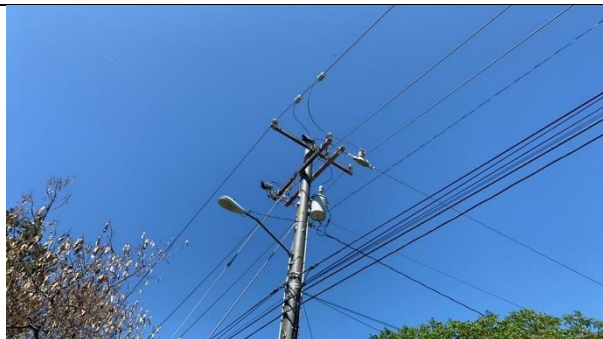
Item6IA1Img1: No vibration dampers
