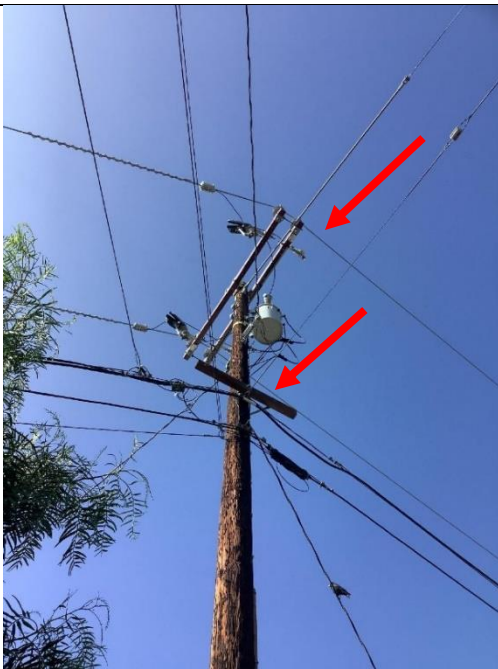
Item8IA1Img1: One side vibration dampers installed
