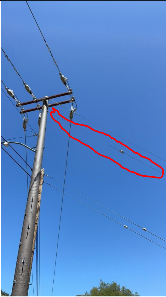
Item6IA1Img1: One of the down guy insulators incorrect type
