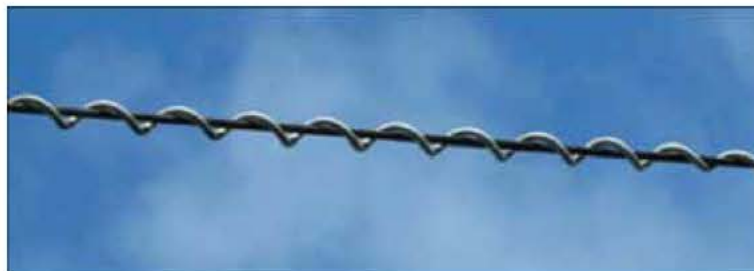
Figure CC 190-1: Spiral Vibration Damper
