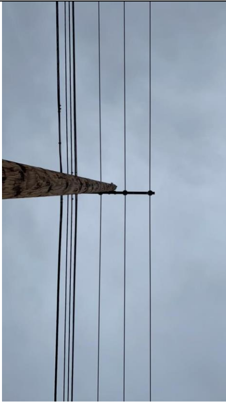
Item7IA1Img1: No vibration dampers
