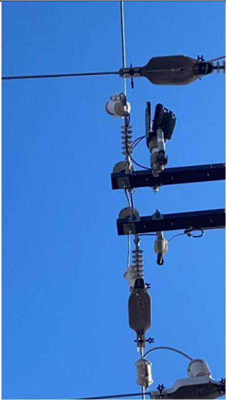
Item9IA2Img1: No bolted wedge connector cover at double dead end
