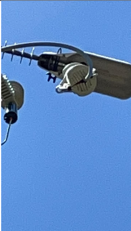
Item2IA2Img1: Missing anti-rotational device at outer notch under dead uncover
