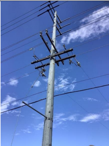
Item6IA1Img1: No vibration damper installed
