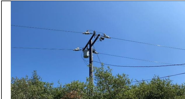
Item2IA1Img1: No vibration dampers on span
