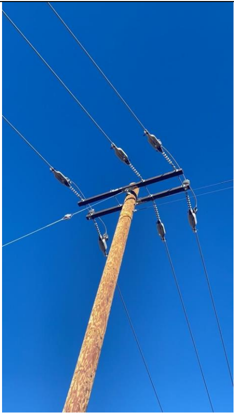
Item9IA1img1: No vibration dampers
