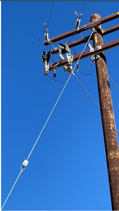
Item13IA2Img1 : Fiberglass down guy wire insulator not installed
