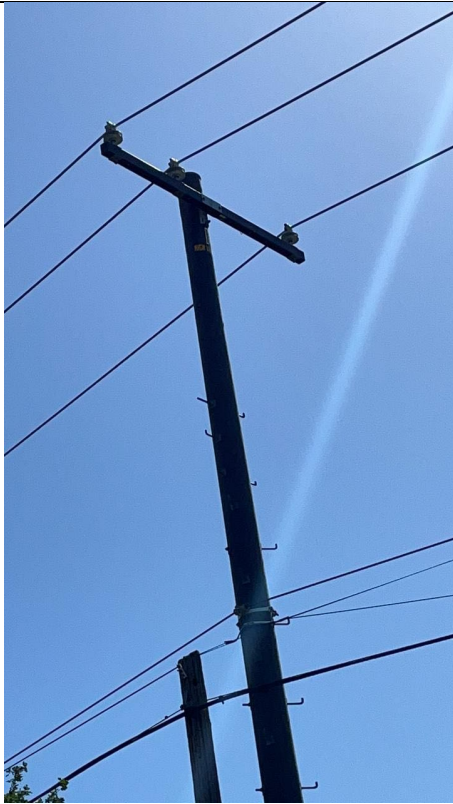
Item1IA1Img1: Missing vibration dampers
