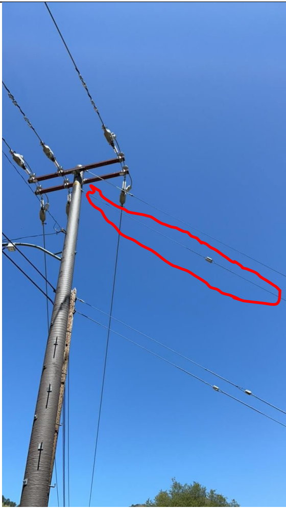
Item6IA1Img1: One of the down guy insulators incorrect type
