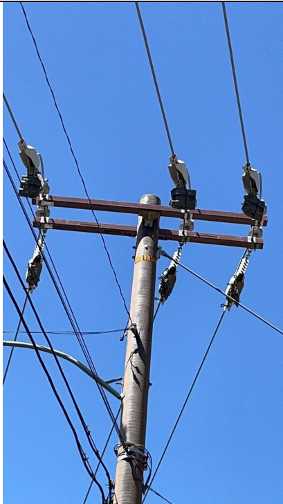
Item4IA1Img1: Missing vibration dampers
