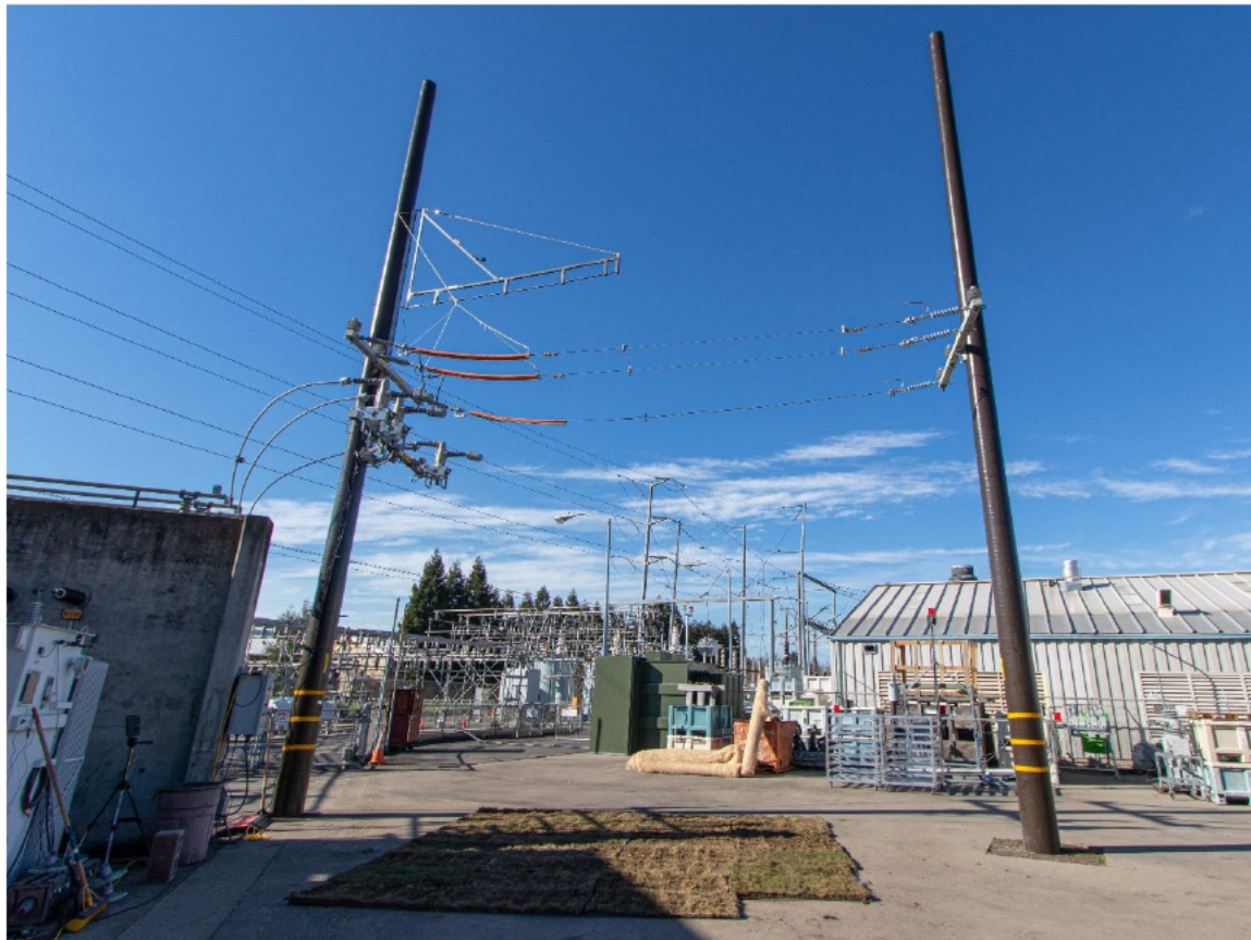
Figure 3: Line-to-line test apparatus
