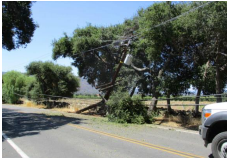
FIGURE PG&E-REMEDY-21-09-10: COVERED CONDUCTOR CONTACT WITH VEGETATION AFTER CAR HIT POLE OJAI, CALIFORNIA – JULY 24, 2020
