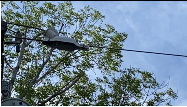
Item1IA1Img1: Covered conductor installed at this pole
