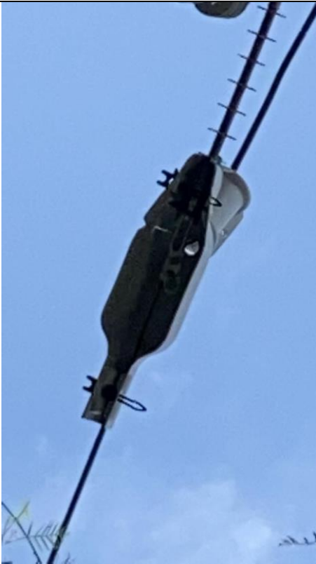
Item1IA2Img1: No anti-rotational clip installed on dead-end cover
