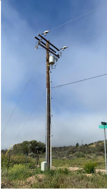
Item4Gimg1: Overall pole
