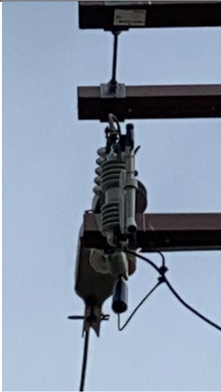
Item4IA1Img1: Missing fuse cover
