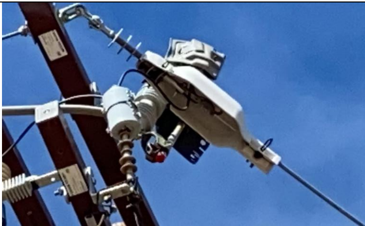
Jumper is not oriented in the direction that the conductor is intended to be routed
