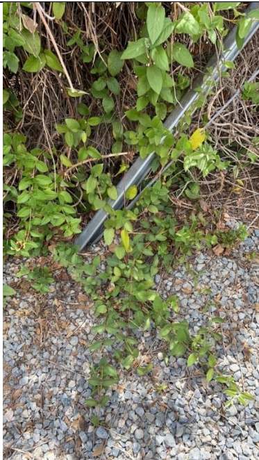
Item8GW1Img1: Buried guy anchor
