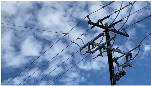
Item6GW1Img1: Close up Loose span guy
