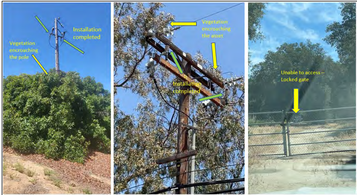
Image 21: Issues on lightning arrestor inspections.
