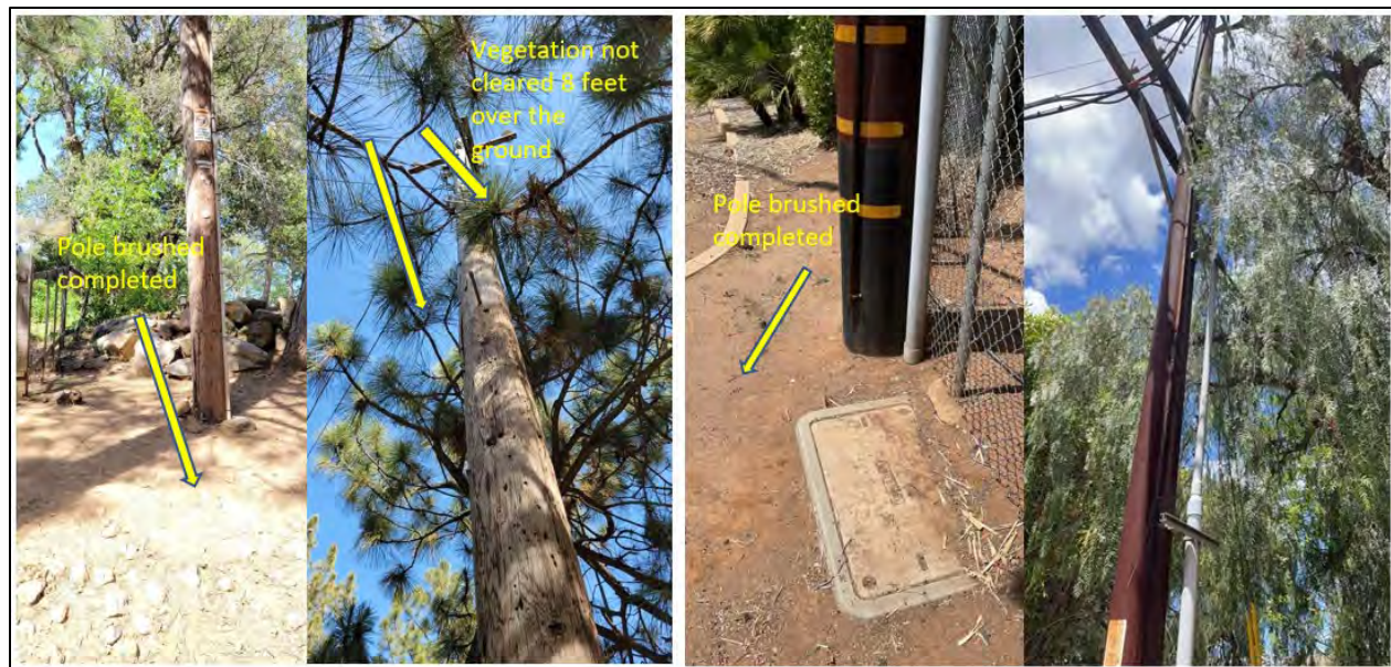
Image 33: Vegetation encroaching on the pole.
