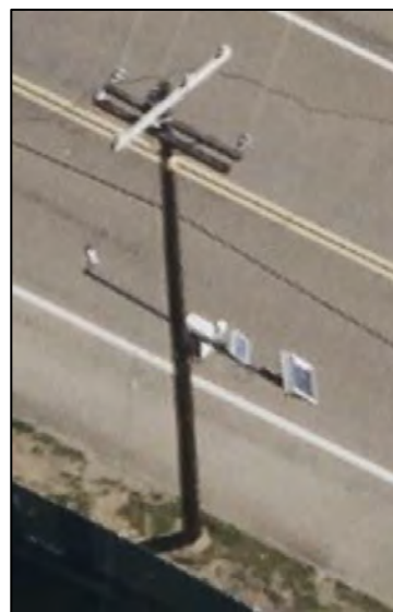
8.1.4. RBV weather station – east
