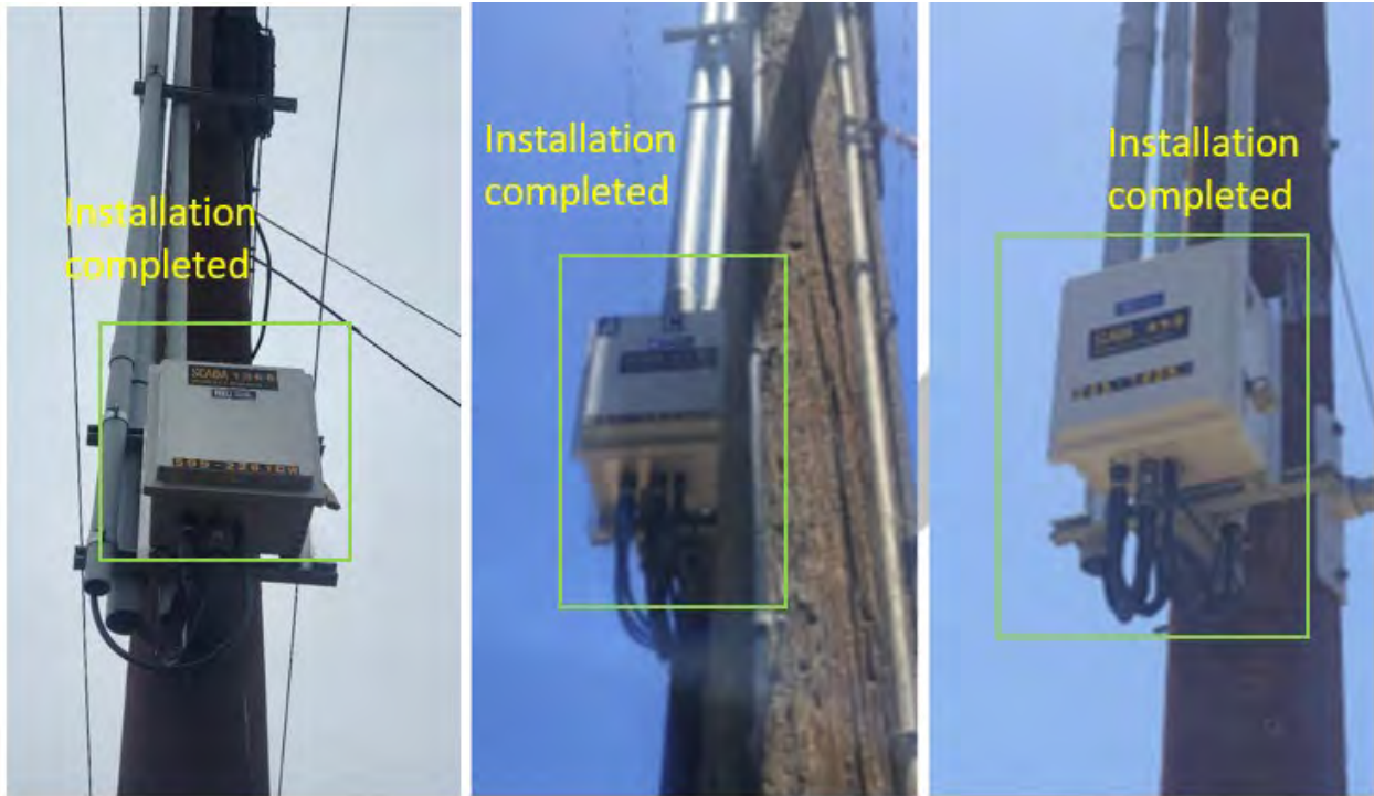
Image 42: SCADA capacitor inspected with no issues.
