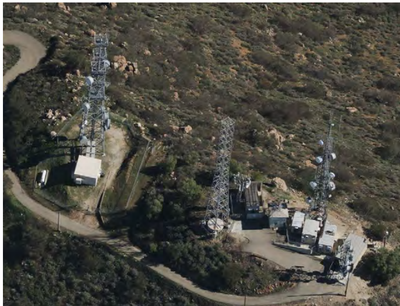
Image 3. DCRI – 000006 Multiple towers with multiple antennas
