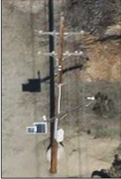
7.1.3. ELM Weather station – north
