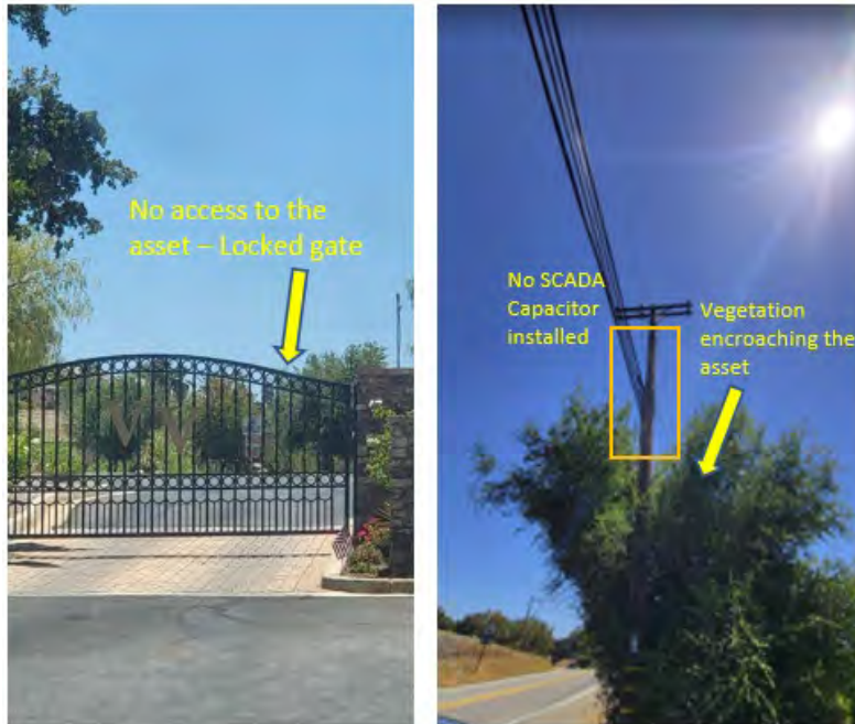
Image 43: No SCADA capacitor installed on the pole.
