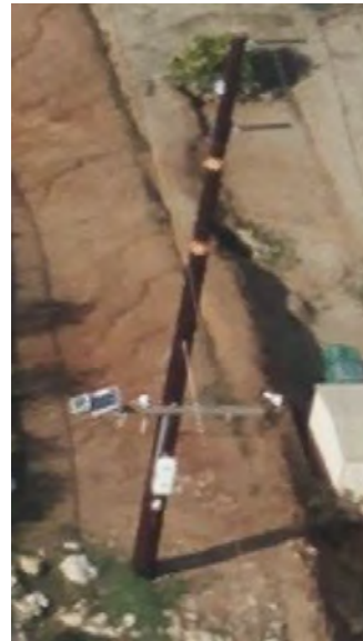
10.1.6. WAL weather station – west
