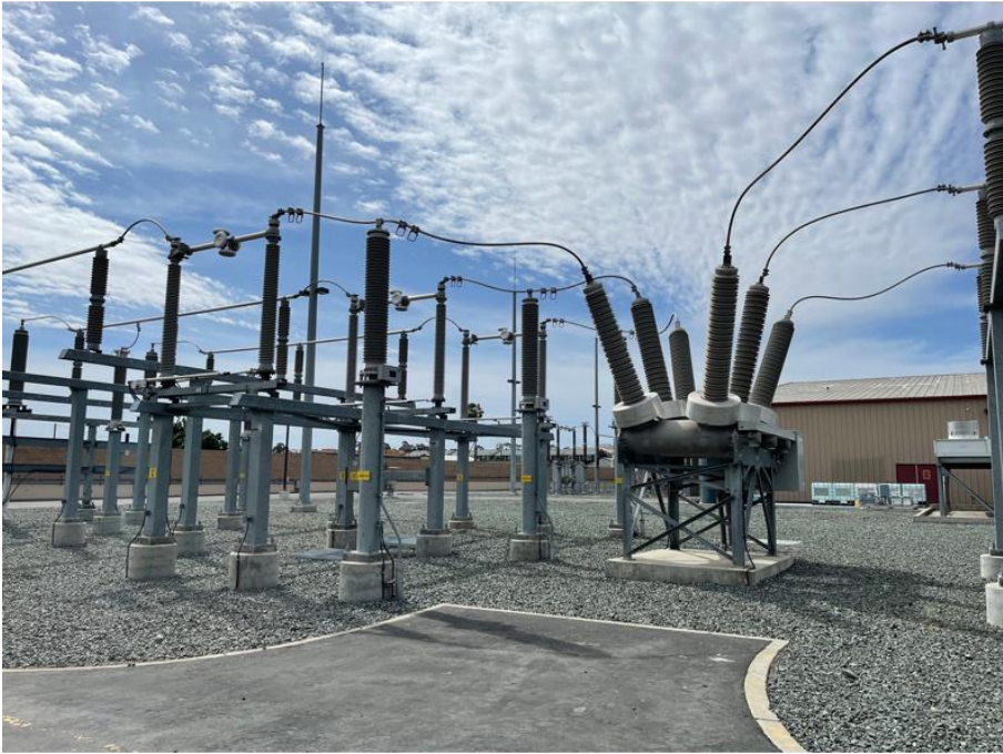
Figure 8: 230-kV Risers and Circuit Breaker
