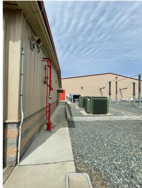
Appendix Figure 10. FD riser located at [REDACTED]
