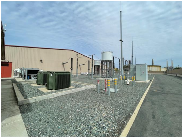
Appendix Figure 8. ±200-kV DC yard
