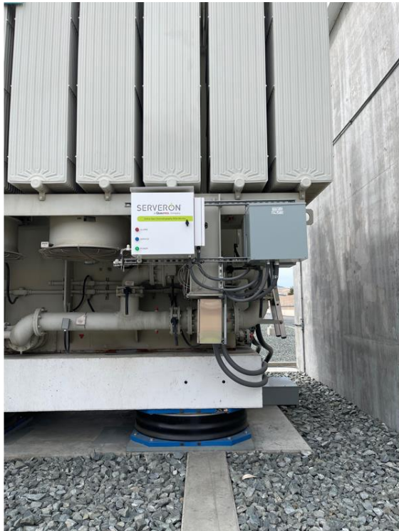
Figure 10: Serveron Monitoring System
