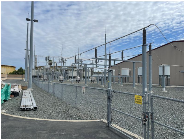
Figure 6: 180-kV AC Yard
