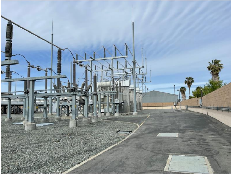
Figure 7: 230/180-kV Transformers and 230-kV AC yard
