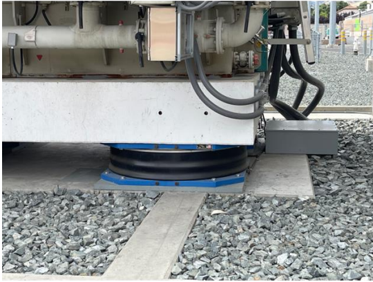
Appendix Figure 7. Seismic base isolators (close up)
