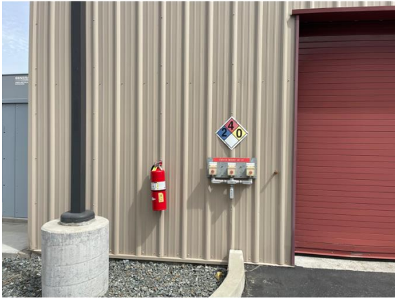
Appendix Figure 11. Generator emergency shutoff
