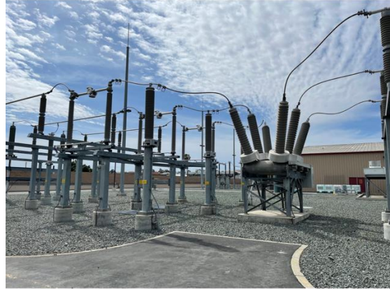
Appendix Figure 9. 230-kV risers and circuit breaker
