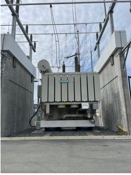
Appendix Figure 6. Seismic base isolators
