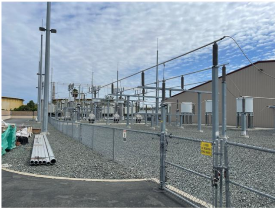
Appendix Figure 3. 180-kV AC yard
