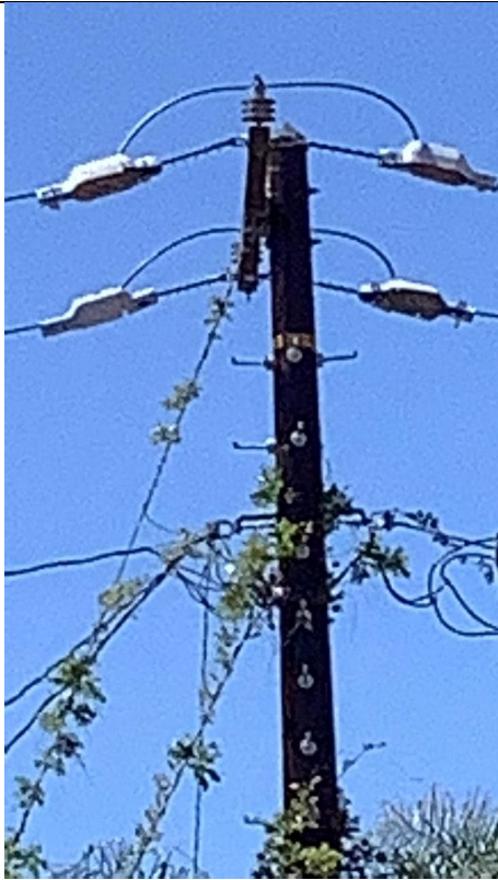
Item8GW2Img1: Vegetation above guy insulator
