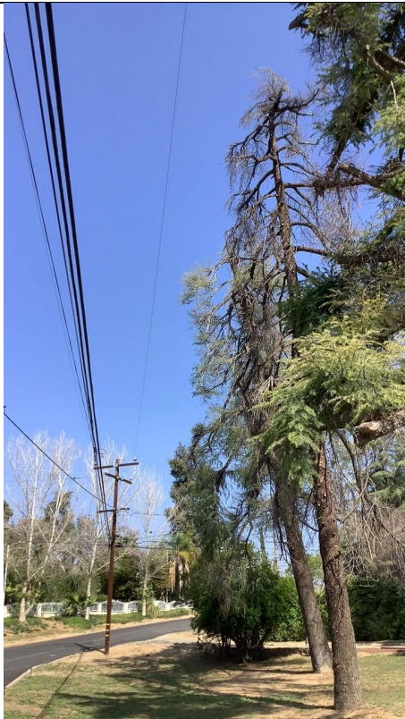
Item1VG6Img1: danger tree near conductor
