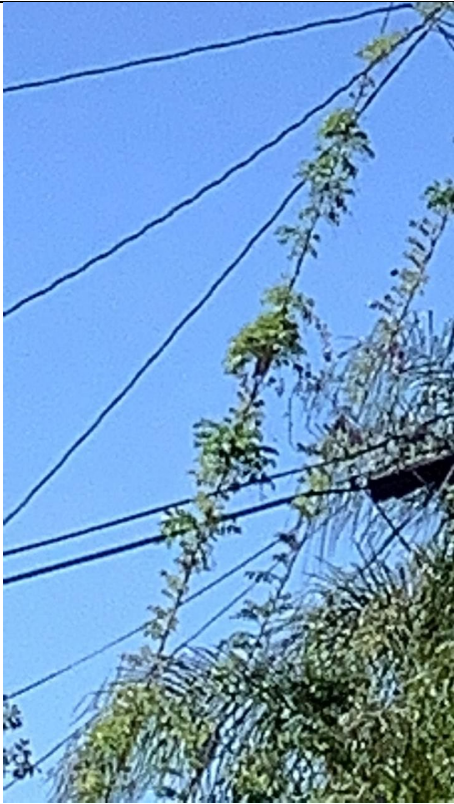
Item8GW2Img2: Vegetation above guy insulator
