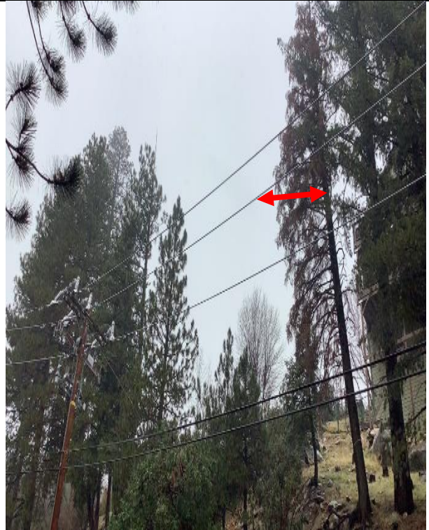
Item3VG6Img4: Proximity of tree to SCE assets
