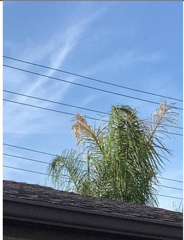
Item9IA1Img4: Palm fronds contacting conductors
