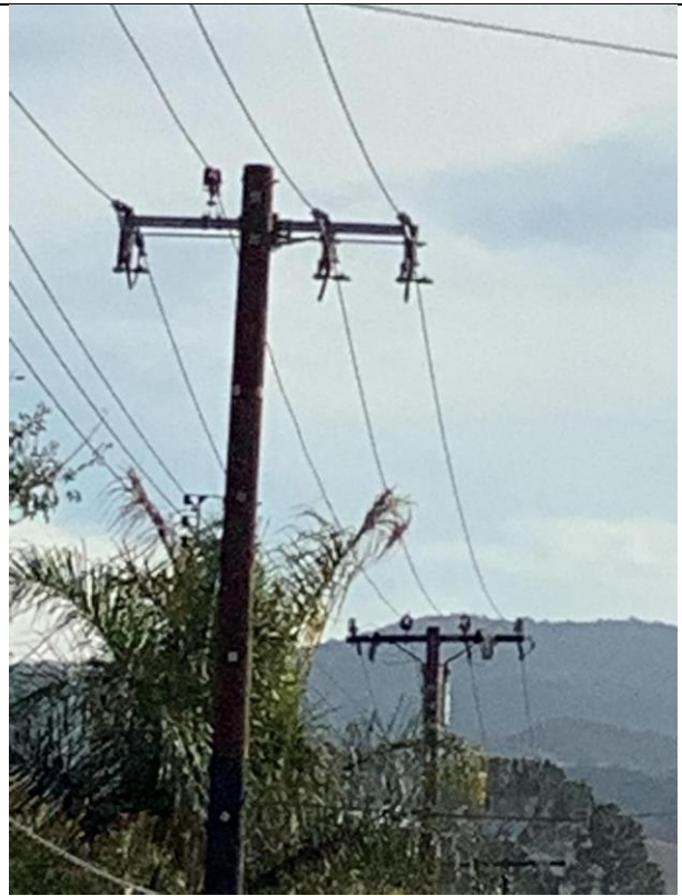
Item9IA1Img2: Palm fronds contacting the conductor.
