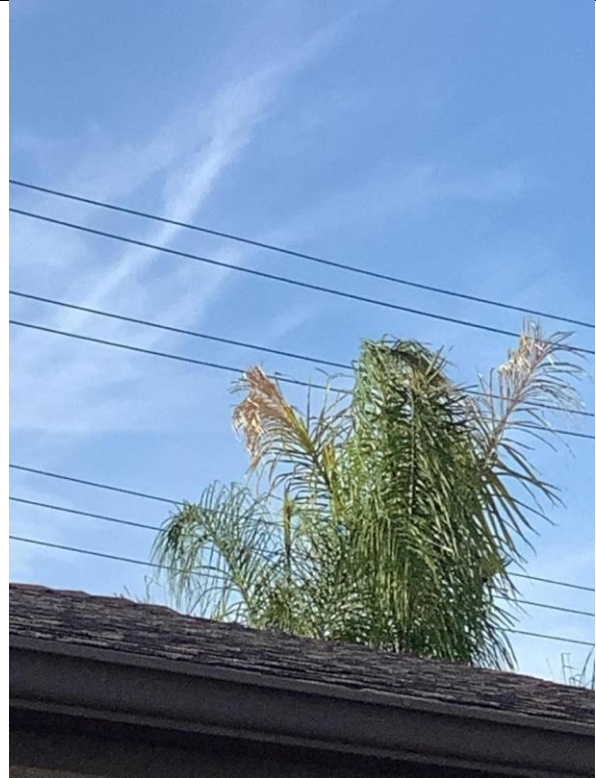
Item9IA1Img4: Palm fronds contacting conductors
