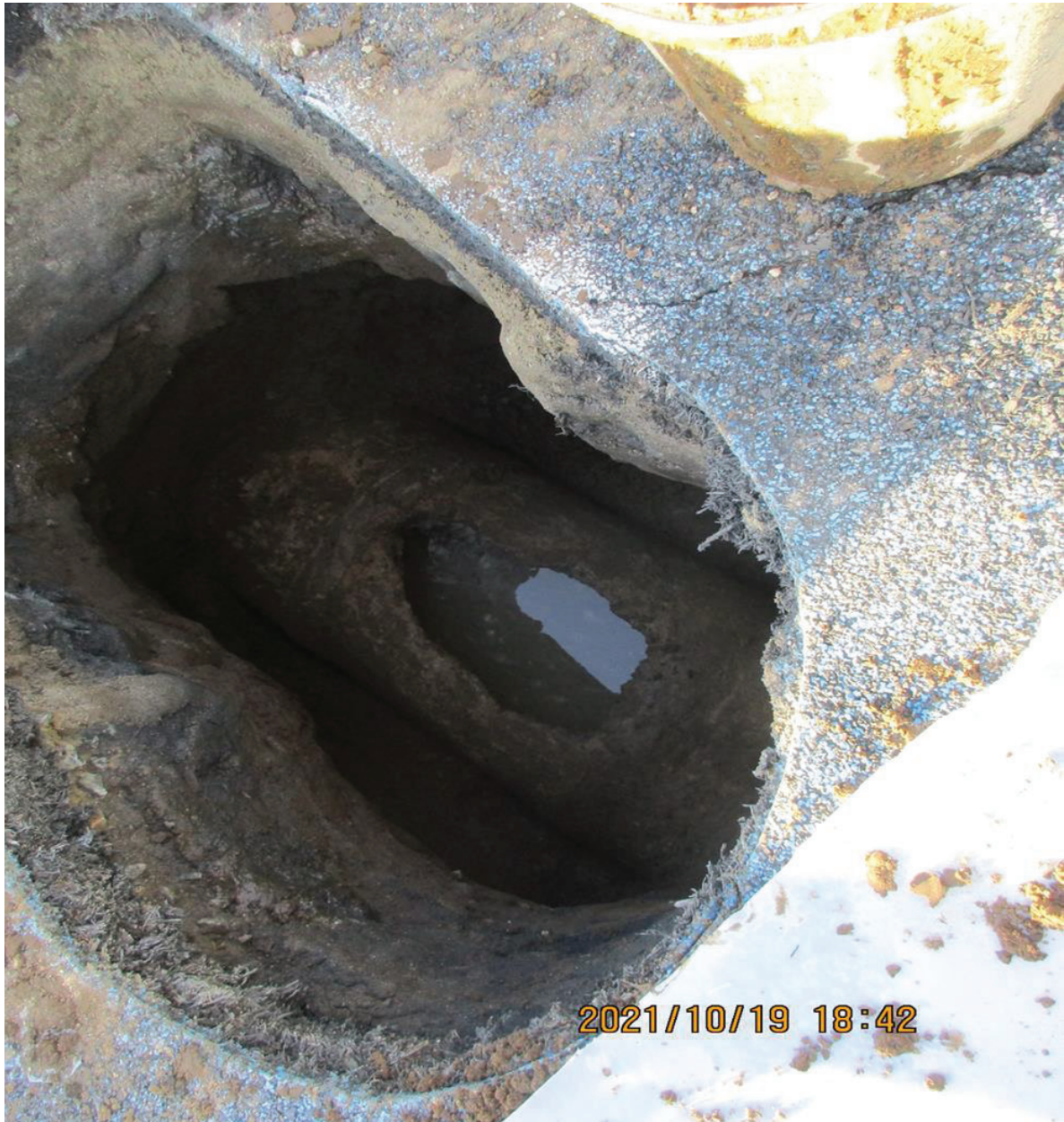
Photo 2 - Damaged Irrigation Pipeline provided by Covina Irrigation Company
