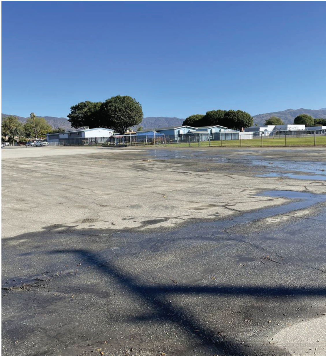
Photo 1 – Leak from damaged irrigation pipe provided by Covina Irrigation Company
