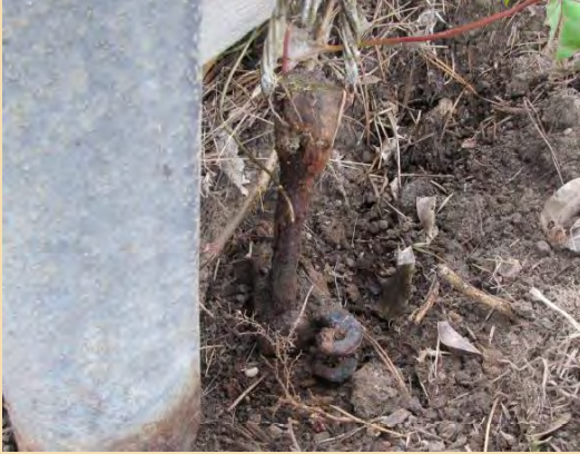
Anchor above ground
