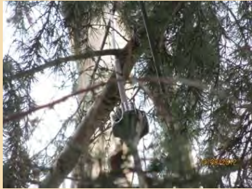
Guy grounded by vegetation
