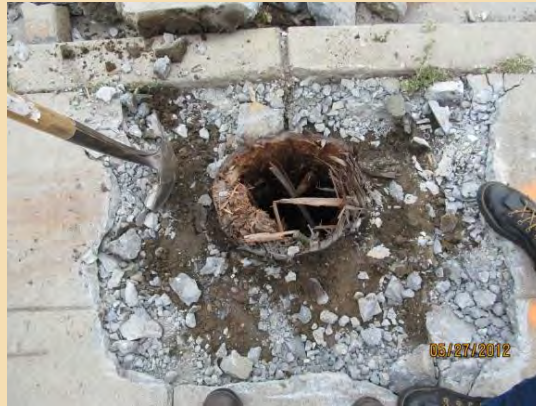
After extraction showing below ground deterioration
