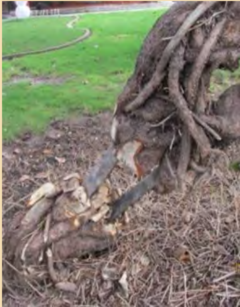
Anchor buried by roots
