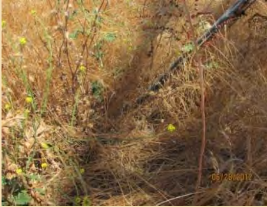
Before: Vegetation covers anchor
