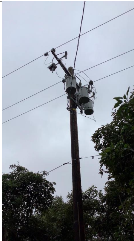
Item3GImg2: Overall view of the pole and covered conductor
