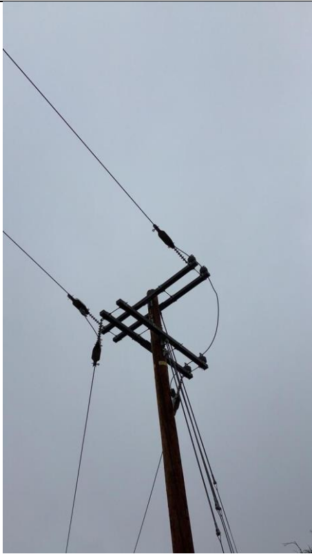
Item2IA1Img1: No vibration dampers are installed
