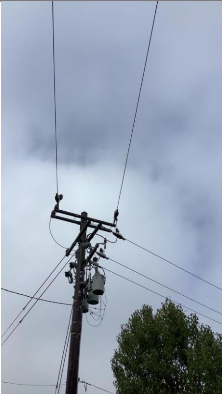
Item1IA1Img1: No vibration dampers are installed
