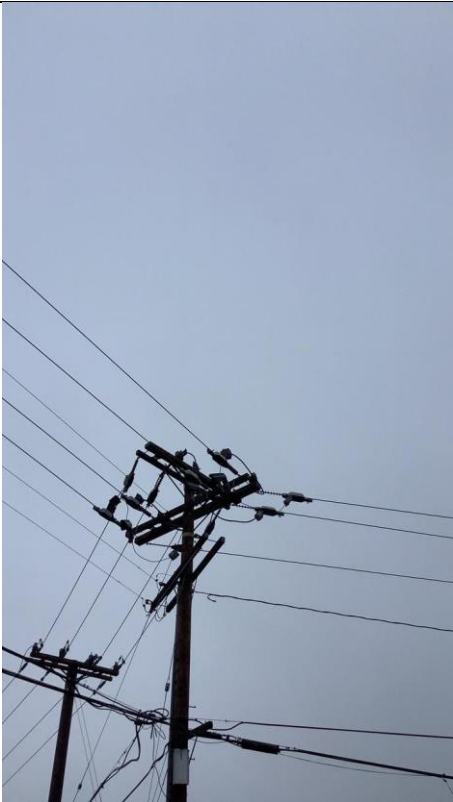
Item1IA1Img1: No vibration dampers are installed
