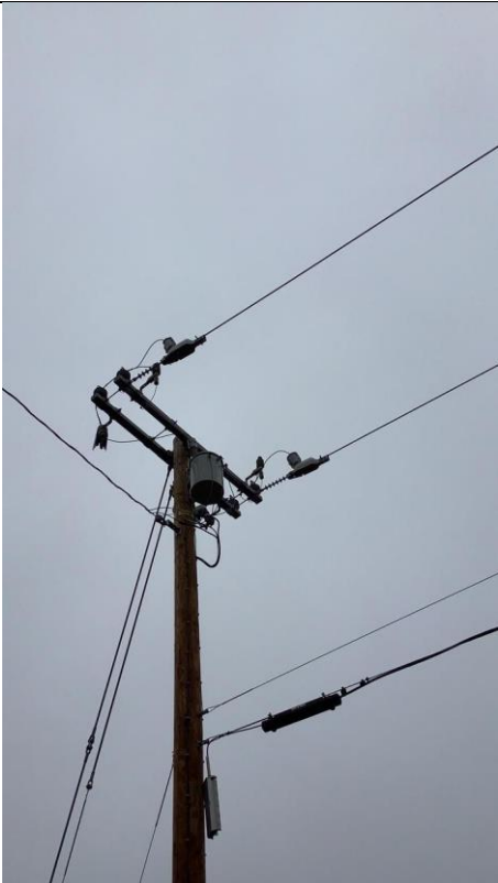
Item4IA1img1: No vibration dampers are installed
