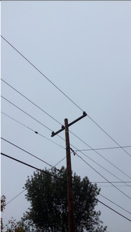
Item2IA1Img1: No vibration dampers are installed
