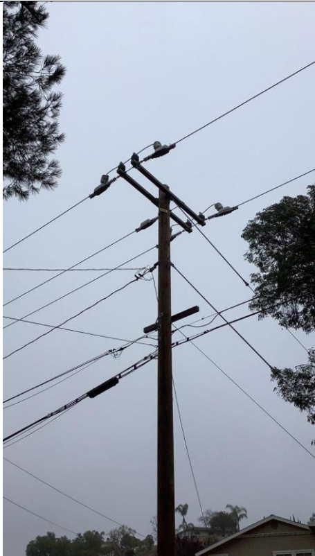
Item3IA1Img1: No vibration dampers are installed
