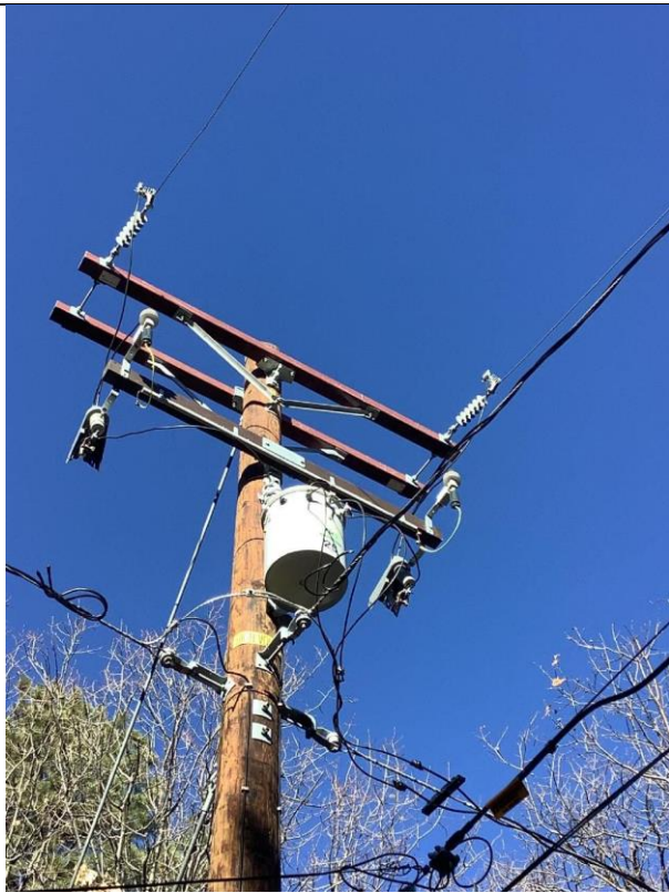
Item4IA1Img1: No covered conductor installed as reported
