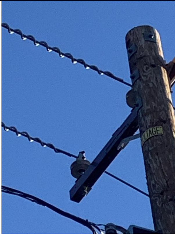
Item2IA1img1: Vibration damper within 6 inches of insulator
