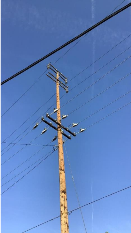
Item1IA1Img1: No vibration dampers are installed
