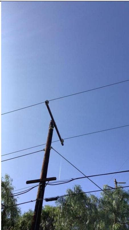
Item1IA1Img1: No vibration dampers are installed
