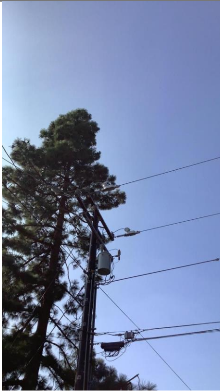
Item2IA1Img1: No vibration dampers are installed
