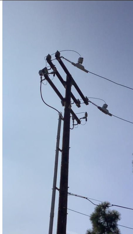
Item3GImg2: Overall view of the pole and covered conductor installed
