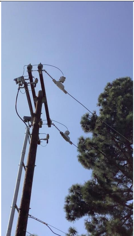
Item3IA1Img1: No vibration dampers are installed
