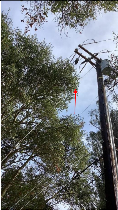
Item4GW2Img2: Vegetation contacting guy wire above insulator
