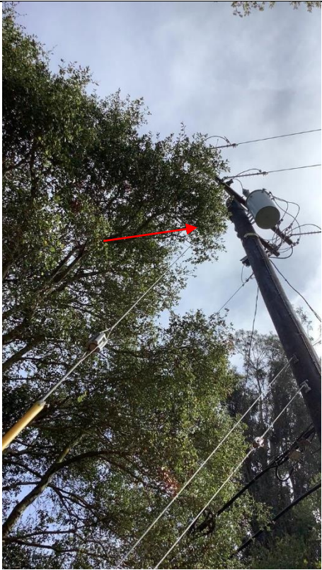
Item4GW2Img1: Vegetation contacting guy wire above insulator
