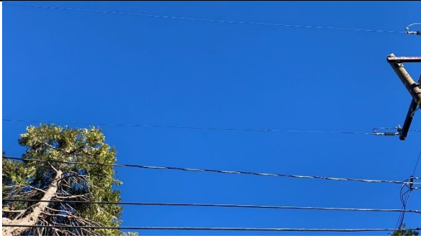
Item6CD9Img1: 3 splices on one phase
