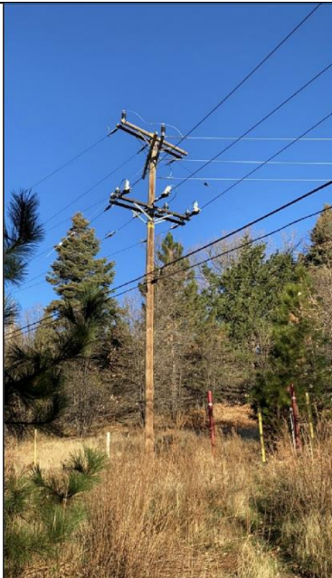
Item1CD2Img1: No wildlife covers at transition from bare to covered conductor
