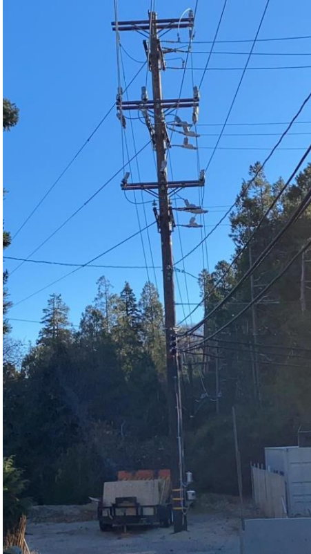
Item4Gimg1: Overall pole
