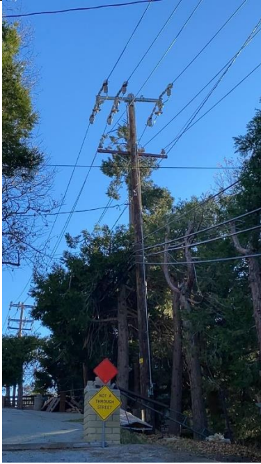
Item3GImg1: Overall pole
