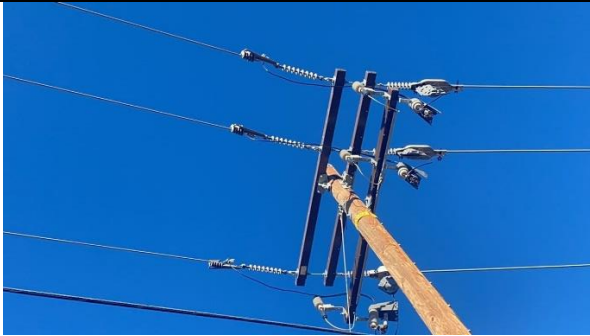
Item2IA3img1: No bolted wedge connector covers when transitioning from bare to covered conductor
