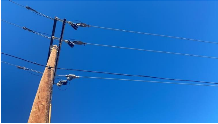
Item2IA1img1: No vibration dampers
