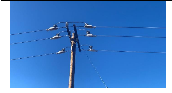
Item13IA1Img1: No vibration dampers
