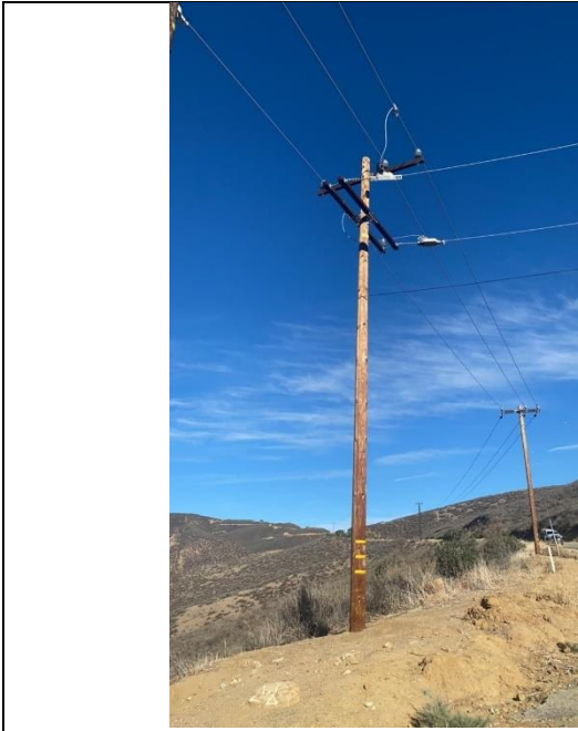
Item8GImg1: Overall pole
