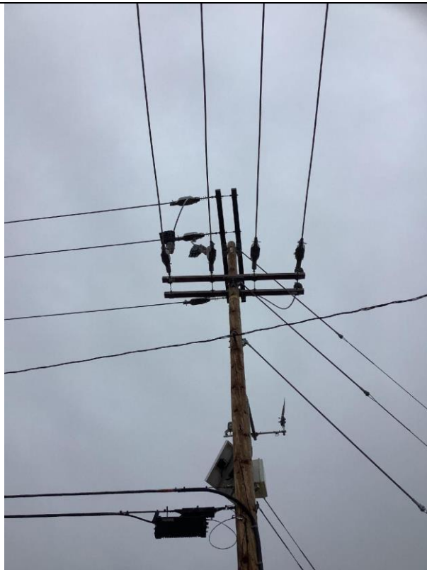
Item15IA1img1: No vibration dampers installed
