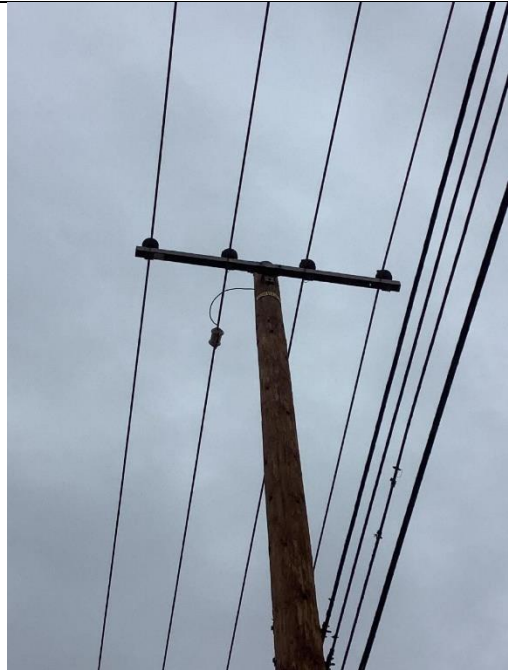
Item10Gimg2: Overall pole
