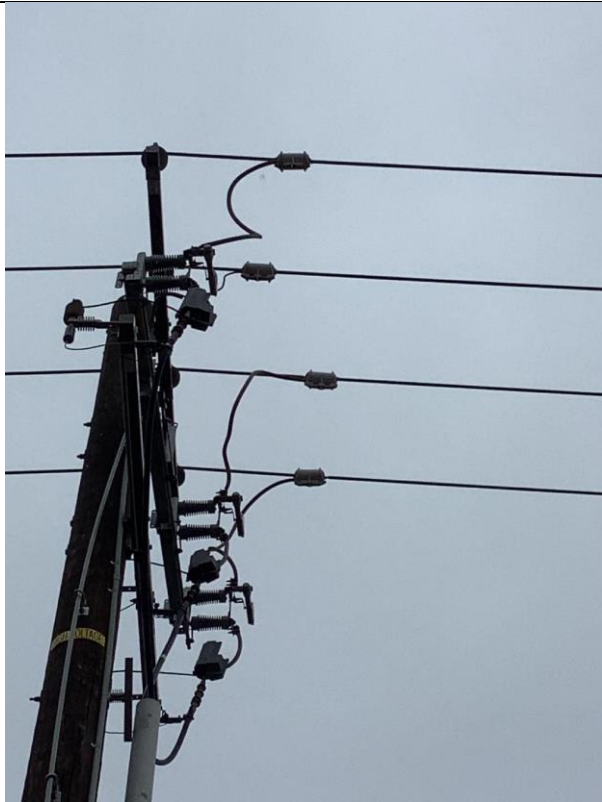
Item6IA1Img1: No vibration dampers installed
