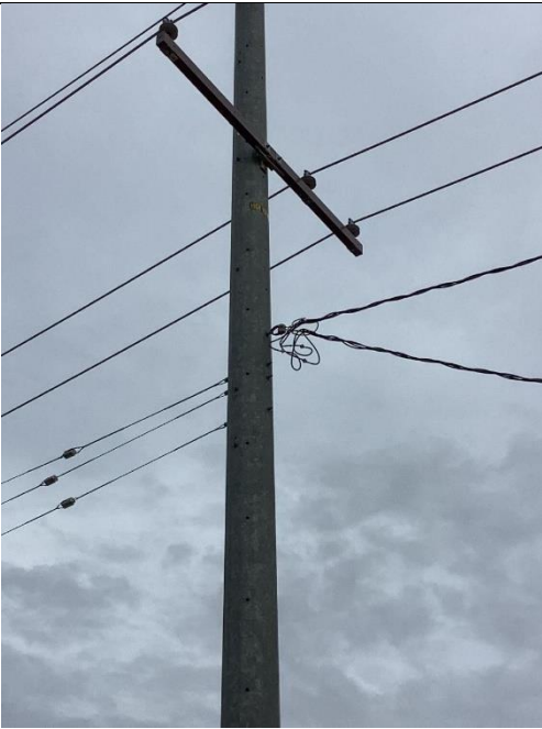
Item17IA1mg1: No vibration dampers installed
