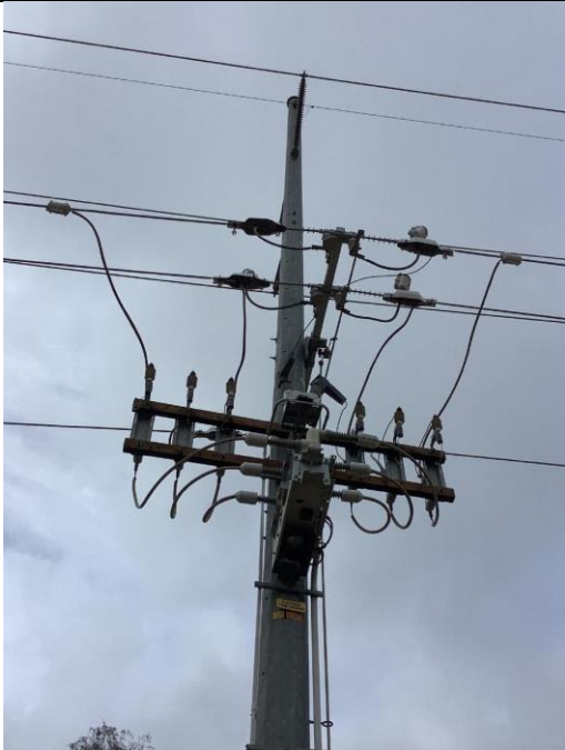
Item19IA1Img1: No vibration dampers installed
