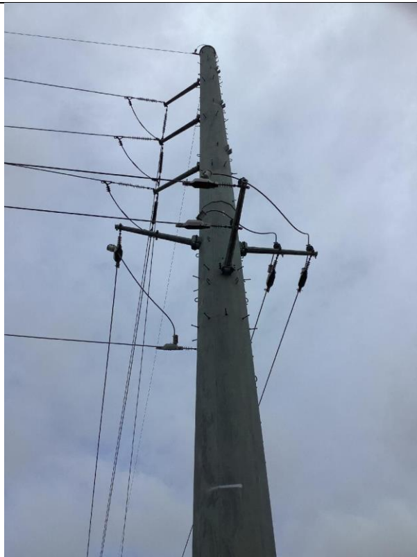
Item20Gimg2: Overall pole
