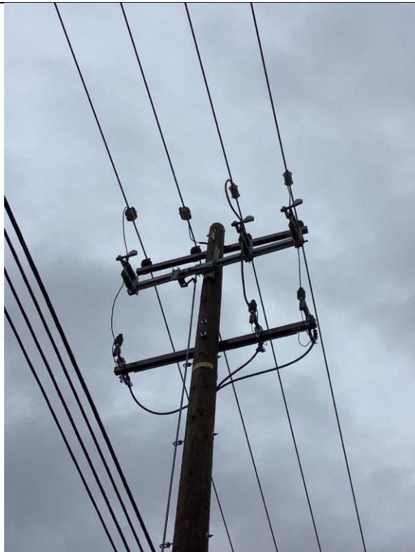
Item11IA1Img1: No vibration dampers installed
