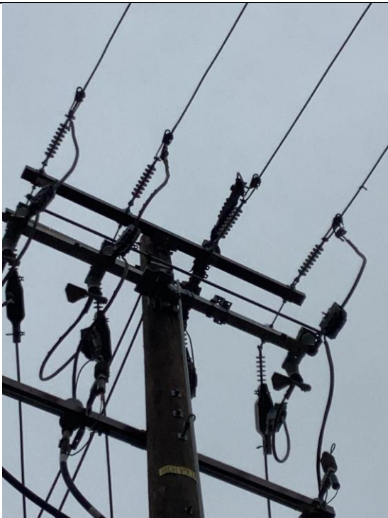
Item16IA2Img1: Bolted wedge connector cover not installed
