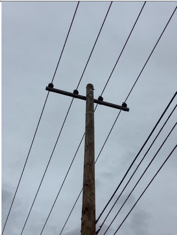
Item12IA1Img1: No vibration dampers installed
