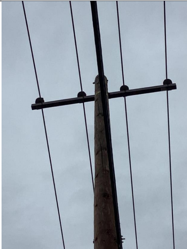
Item8IA1Img1: No vibration dampers installed
