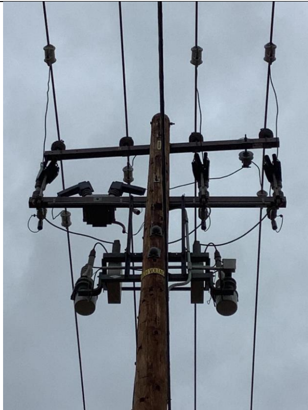
Item13IA1mg1: No vibration dampers installed
