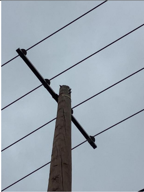
Item7IA1Img1: No vibration dampers installed
