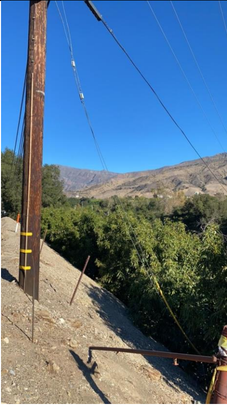
Item2GW1Img1: Overview of pole with loose down guy wire
