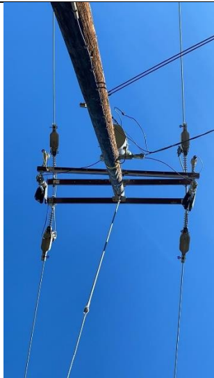
Item8IA1Img1: Vibration dampers not installed
