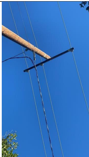
Item15IA1img1: Vibration dampers not installed
