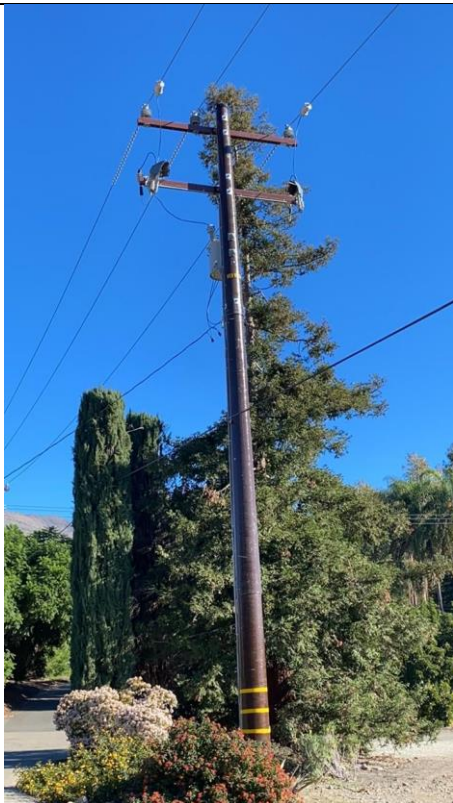
Item5Gimg1: Overall pole
