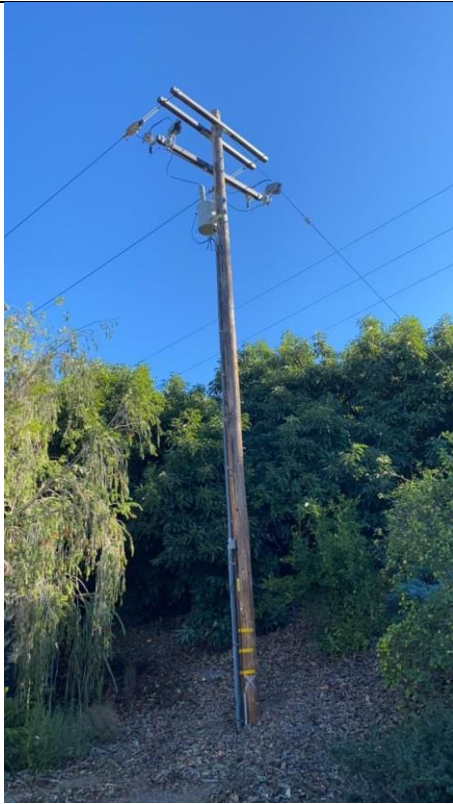
Item12GImg1: Overall pole
