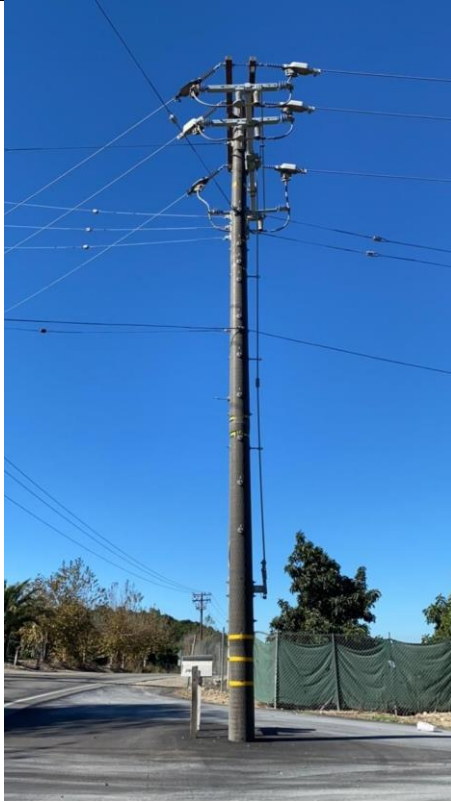
Item6GImg1: Overall pole
