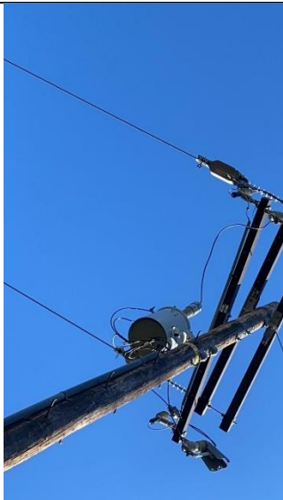
Item12IA1img1: Vibration dampers not installed
