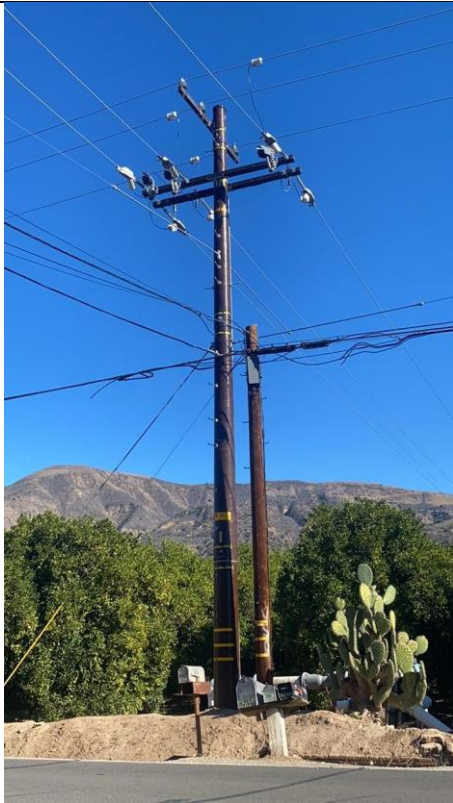
Item14GImg1: Overall pole
