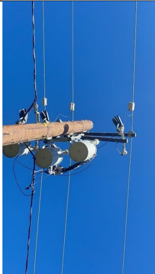
Item16IA1Img1: No vibration dampers installed
