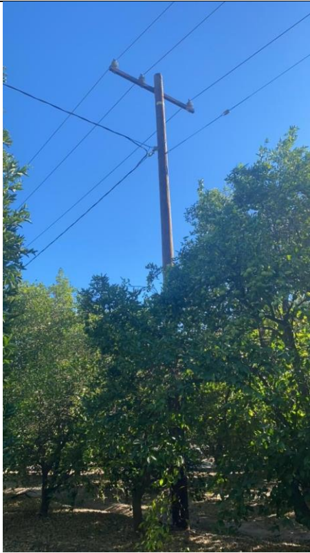
Item15GImg1: Overall pole
