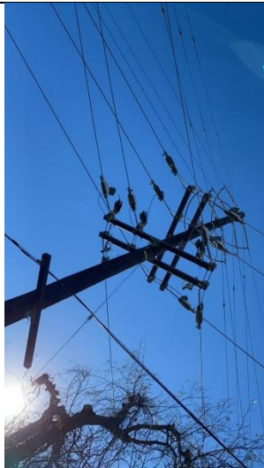
Item7IA1Img1: Vibration dampers not installed
