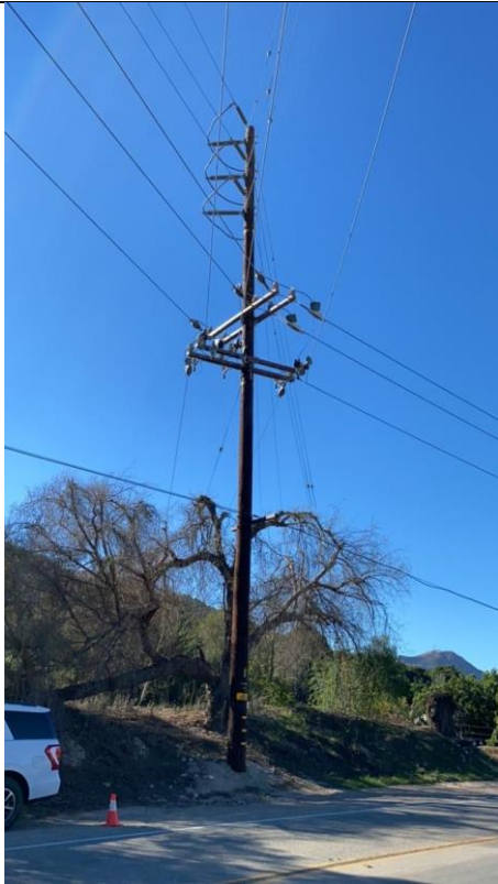
Item7GImg1: Overall pole
