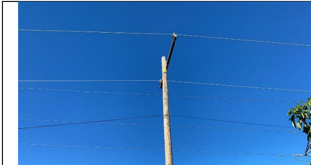
Item9IA1img1: Vibration dampers not installed
