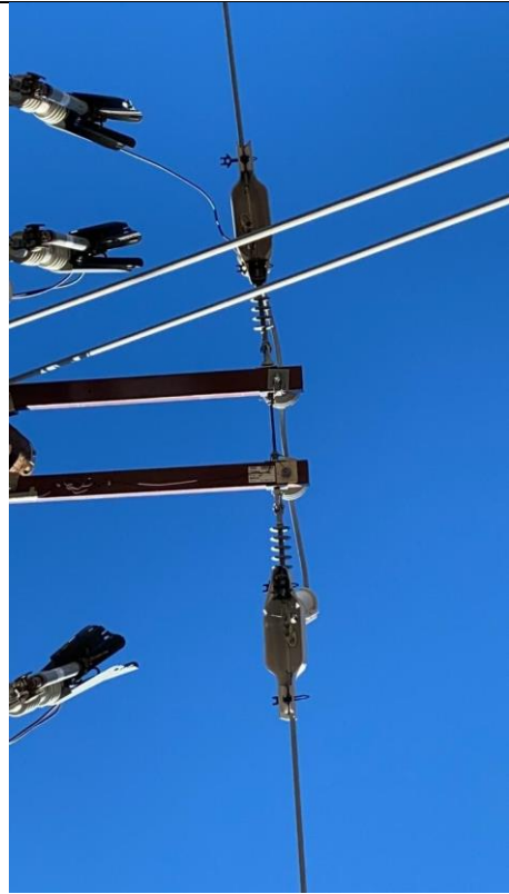
Item1IA1mg2: Close up, no vibration dampers installed
