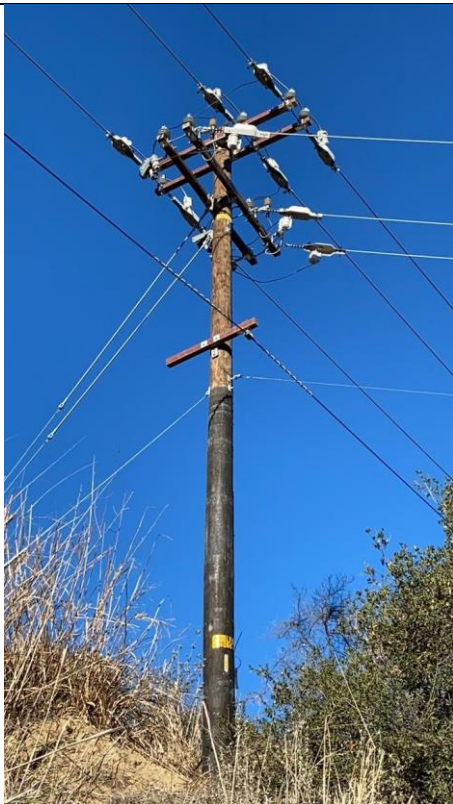
Item1Gimg1: Overall pole
