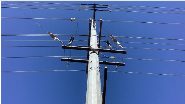
Item5IA1img1: No vibration dampers installed
