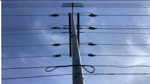
Item11IA1img1: Vibration dampers not installed
