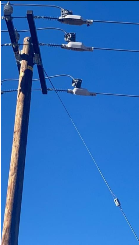
Item13IA2Img1: Porcelain guy insulator
