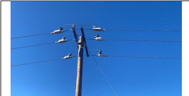
Item13IA1Img1: No vibration dampers
