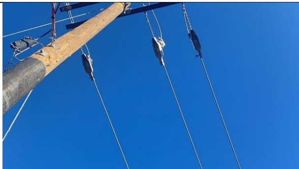
Item3IA1Img1: No vibration dampers
