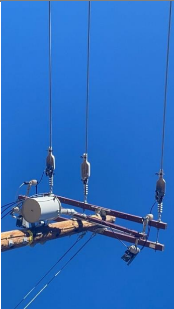
Item14IA1img1: No vibration dampers
