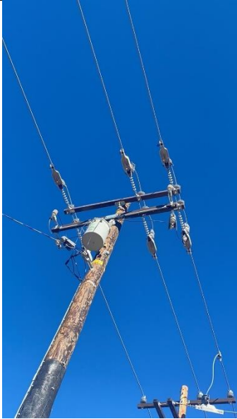
Item7IA1Img1: No vibration dampers
