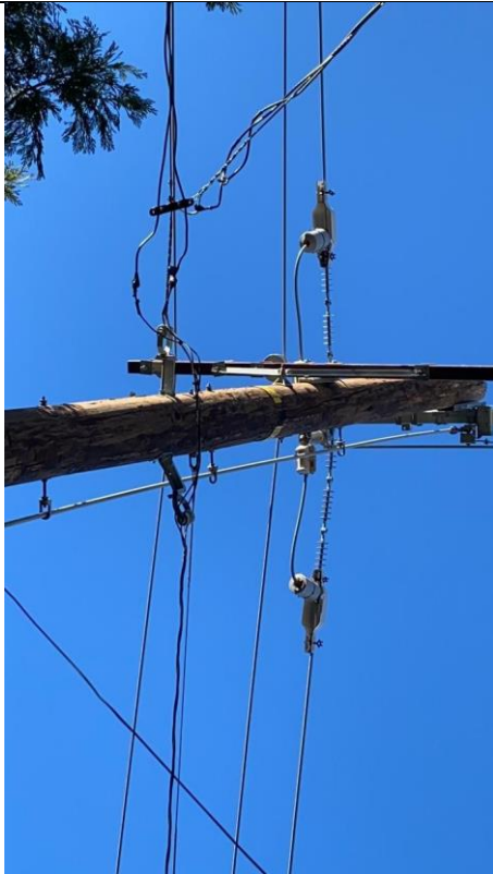
Item3IA1Img1: No vibration dampers
