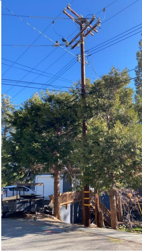
Item9GImg1: Overall pole
