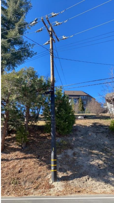
Item15GImg1: Overall Pole
