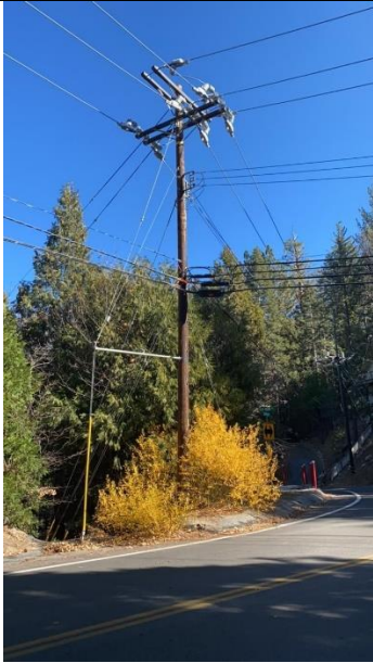
Item19GImg1: Overall pole
