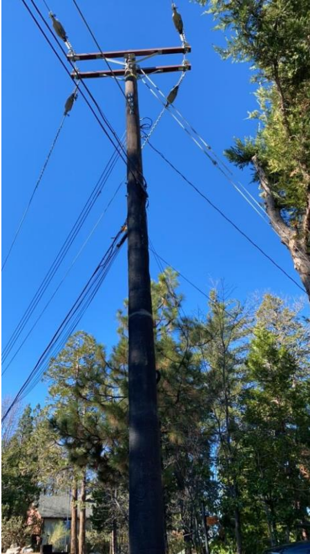
Item10Gimg1: Overall pole
