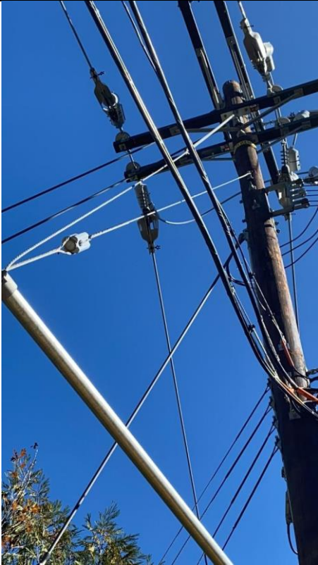
Item19IA1Img1: Missing fiberglass guy wire insulator
