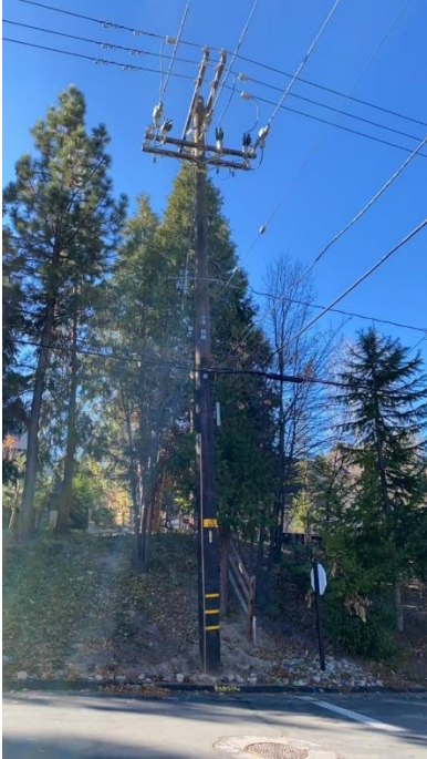
Item12Gimg1: Overall pole
