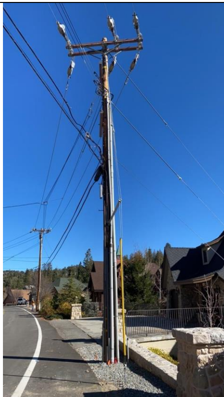
Item14Gimg1: Overall Pole
