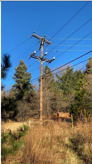
Item1Gimg1: Overall pole
