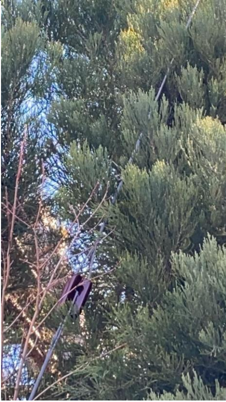
Item5GW2Img1: Vegetation touching guy wire above insulator
