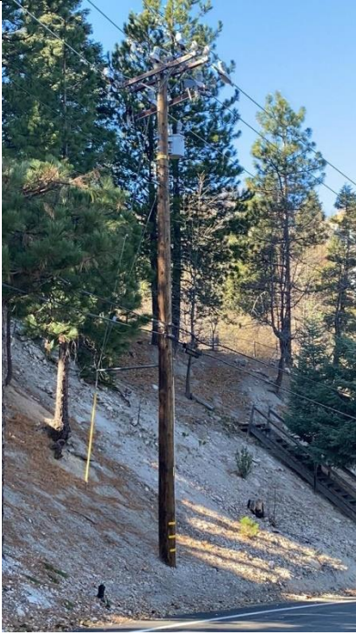
Item17Gimg1: Overall pole
