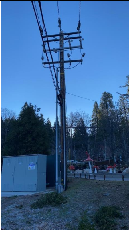
Item2GImg1: Overall pole
