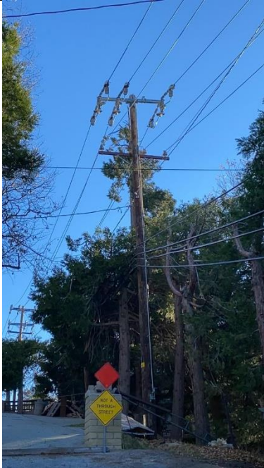
Item3GImg1: Overall pole
