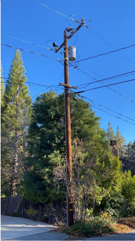
Item5GImg1: Overall pole
