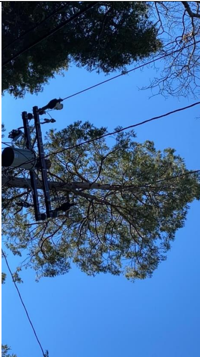
Item7IA1img1: No vibration dampers
