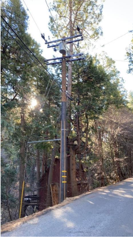
Item7GImg1: Overall pole
