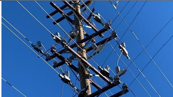
Item4IA2Img1: No vibration dampers
