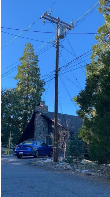
Item11Gimg1: Overall pole
