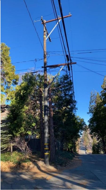
Item6GImg1: Overall pole
