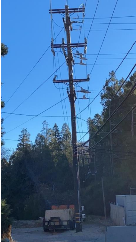
Item4GImg1: Overall pole
