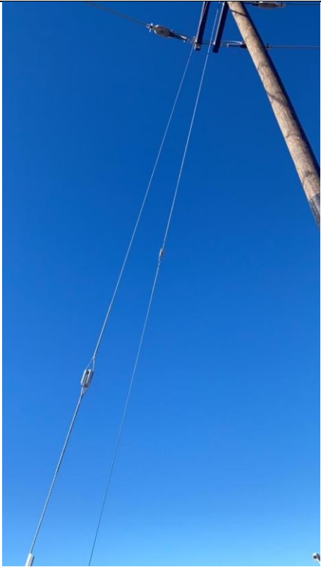
Item12IA2Img1: Porcelain guy insulators on two guy wires
