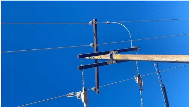
Item5IA1Img1: No vibration dampers
