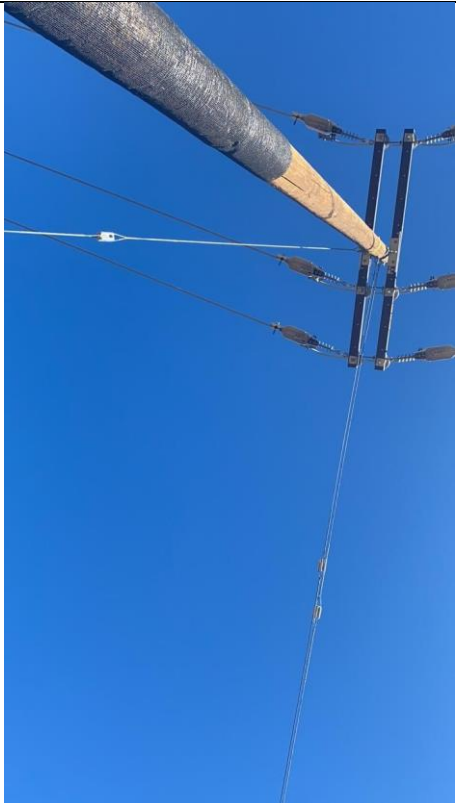
Item11IA2Img1: Porcelain guy insulators on three guys
