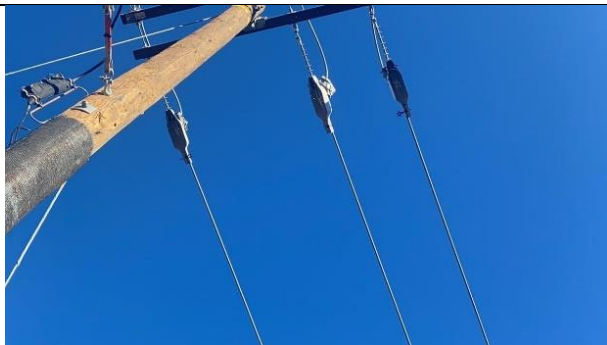
Item3IA1Img1: No vibration dampers
