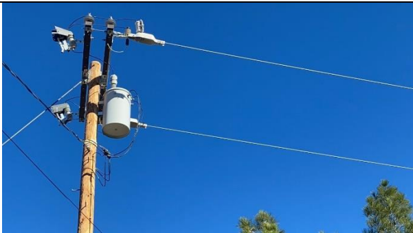
Item10IA1img1: No vibration dampers
