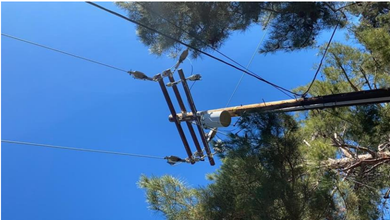
Item17IA1img1: No vibration dampers
