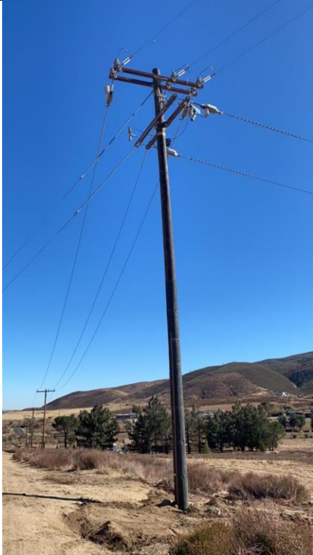
Item15GImg1: Overall pole
