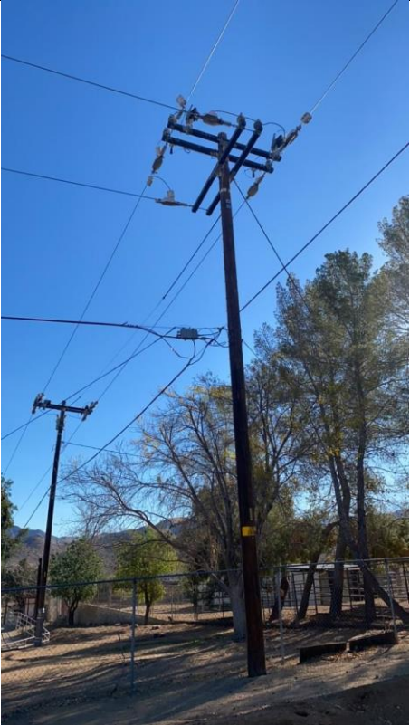
Item9GImg1: Overall pole
