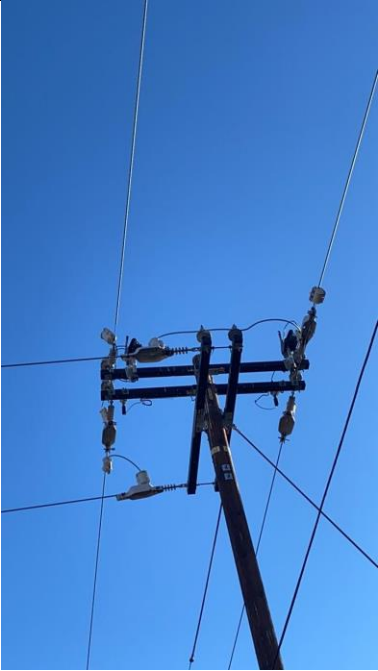
Item9IA1Img1: No vibration dampers
