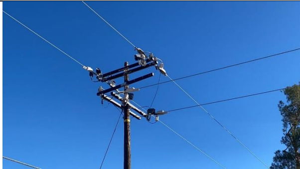
Item6IA1Img1: No vibration dampers
