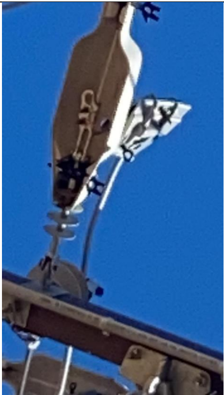
Item16IA2Img1: Loose center phase bolted wedge connector
