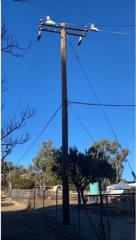
Item2GImg1: Overall pole
