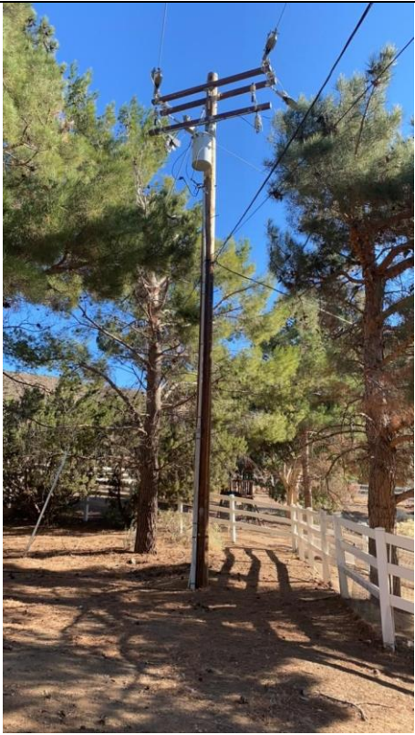
Item17GImg1: Overall pole
