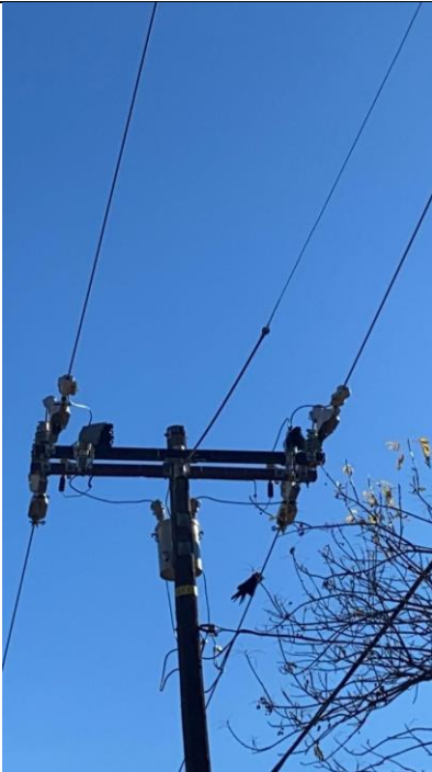
Item8IA1Img1: No vibration dampers
