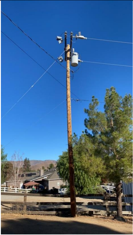
Item10GImg1: Overall pole
