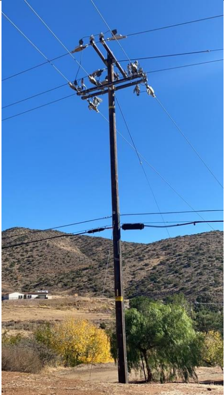
Item16GImg1: Overall pole
