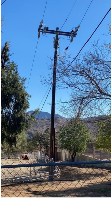
Item8GImg1: Overall pole
