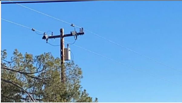
Item5IA1img1: No vibration dampers
