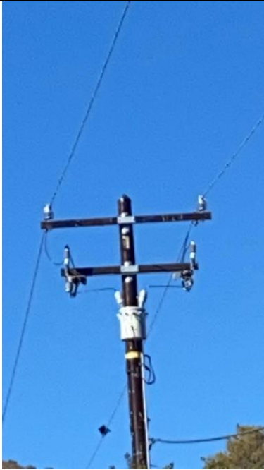
Item7IA1Img1: No vibration dampers
