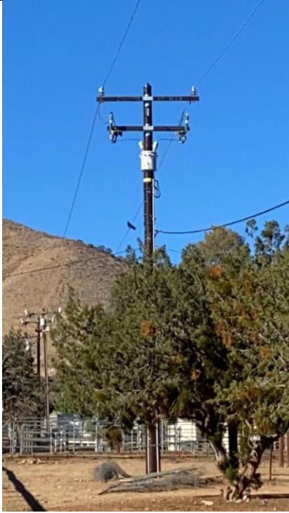
Item7GImg1: Overall pole
