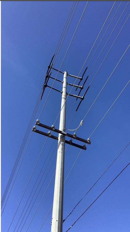
Item4IA1img1: Steel pole observed in the field and no vibration dampers installed
