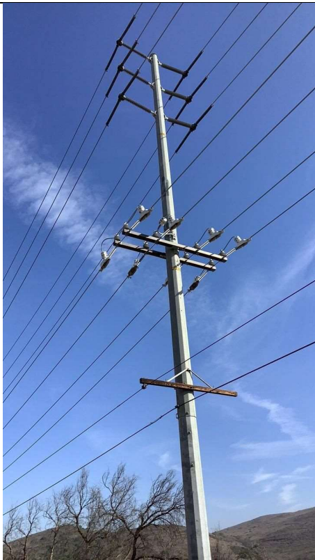
Item8IA1Img1: No vibration dampers are installed
