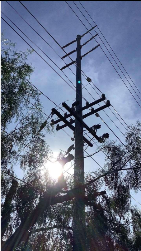
Item9IA1img1: Steel pole observed in the field and no vibration dampers are installed
