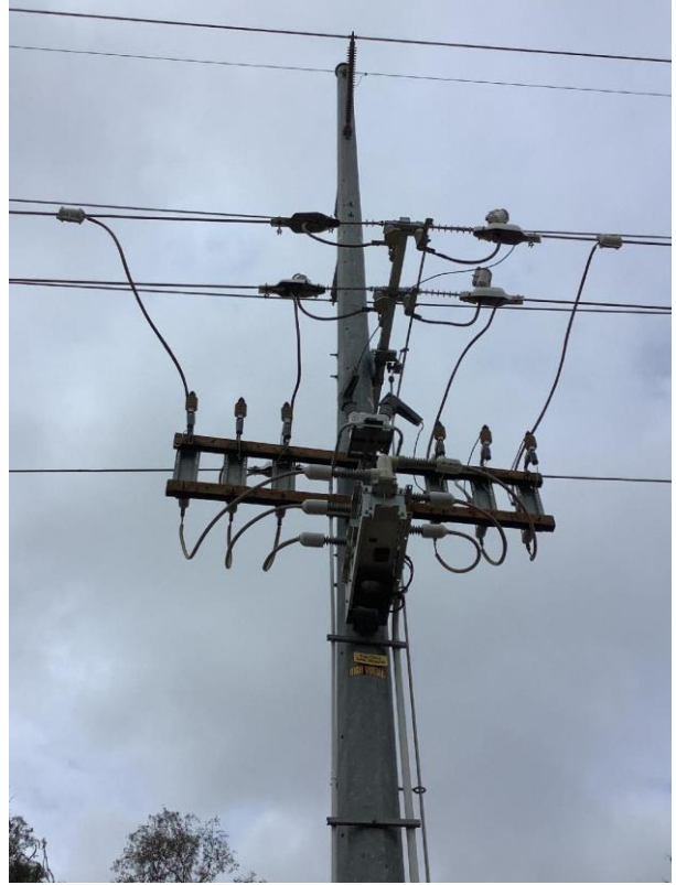
Item19GImg2: Overall pole
