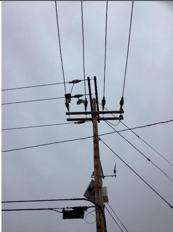
Item15IA1img1: No vibration dampers installed
