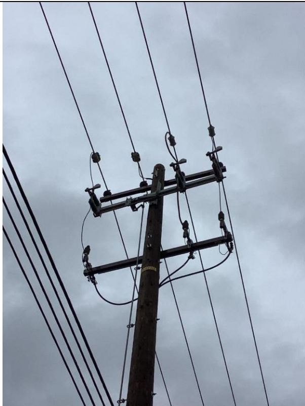
Item11IA1Img1: No vibration dampers installed
