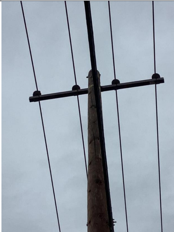
Item8IA1Img1: No vibration dampers installed
