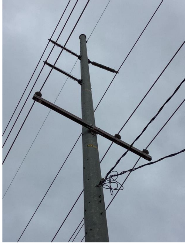
Item17G1mg2: Overall pole
