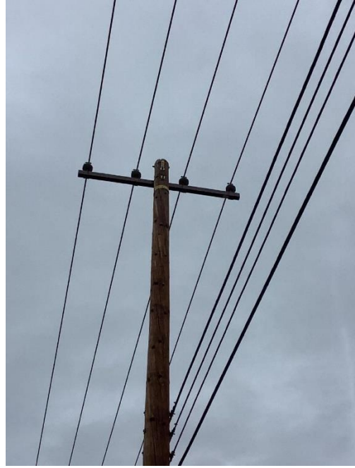
Item9GImg2: Overall pole
