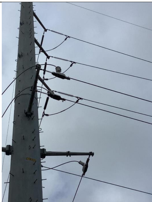
Item20IA1img1: No vibration dampers installed
