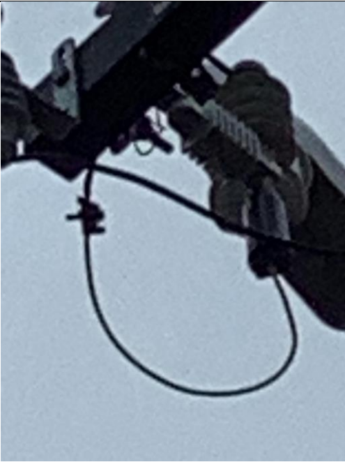
Item4IA2Img1: Close up of clamp not covered
