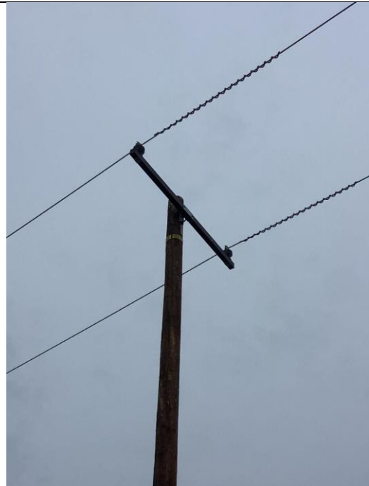
Item3GImg2: Overall pole
