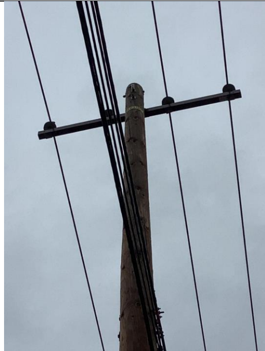
Item8GImg2: Overall pole
