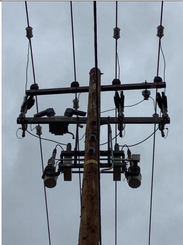
Item13IA1Img1: No vibration dampers installed
