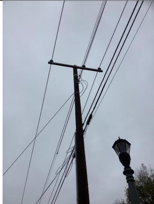
Item14GImg2: Overall pole
