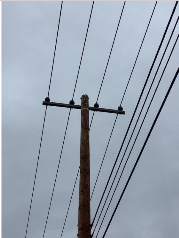
Item9IA1Img1: No vibration dampers installed
