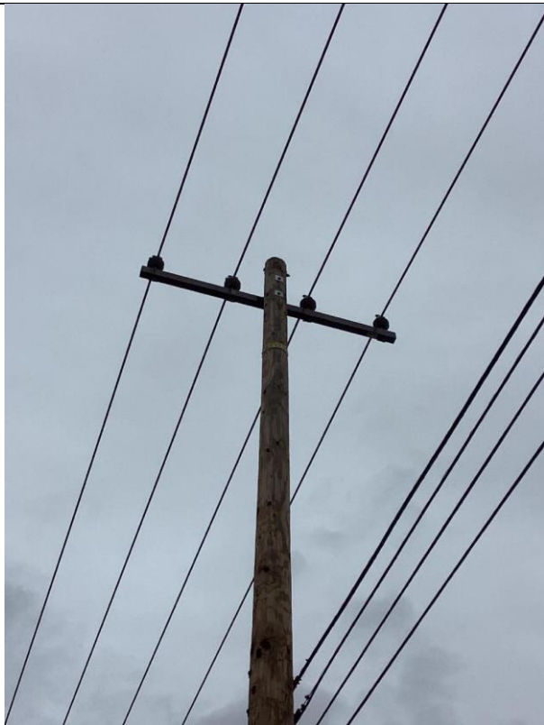
Item12IA1Img1: No vibration dampers installed
