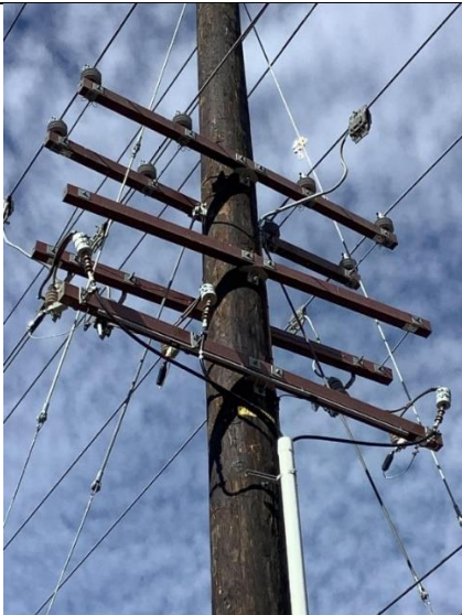
Item5IA1Img1: No vibration dampers installed
