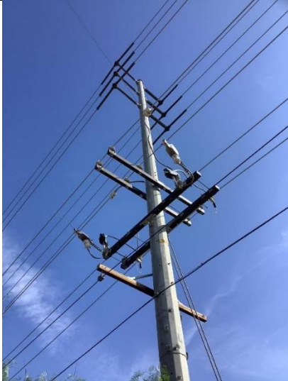
Item11IA1img1: No vibration dampers installed
