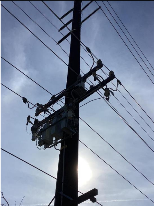
Item14IA1Img1: No vibration dampers installed
