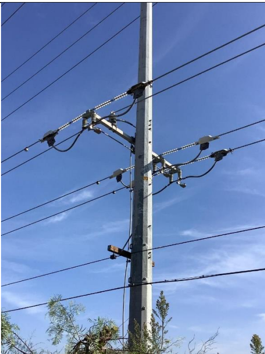
Item13IA1img1: No vibration dampers installed
