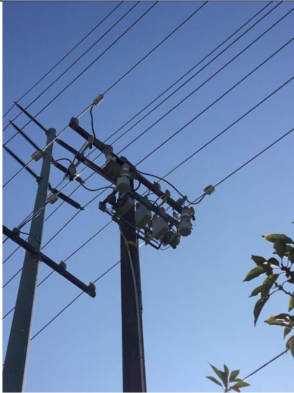
Item4GImg1: Overall pole
