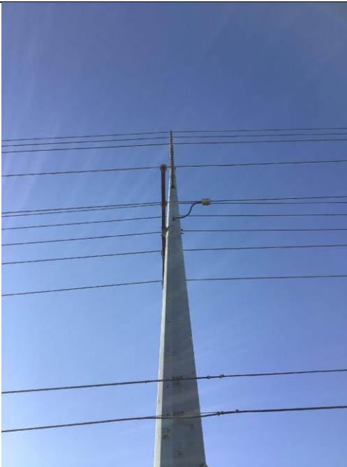
Item2IA1mg1: No vibration dampers installed
