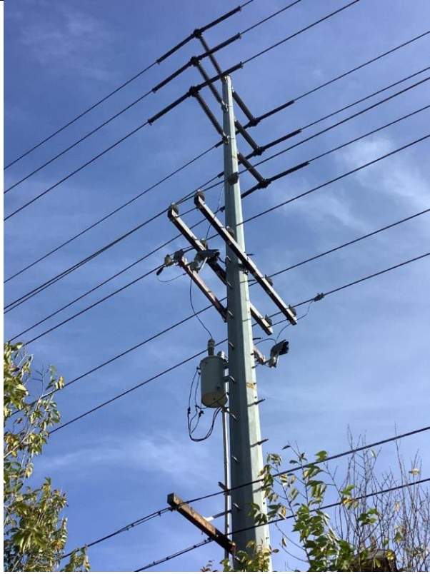
Item15GImg1: Overall pole
