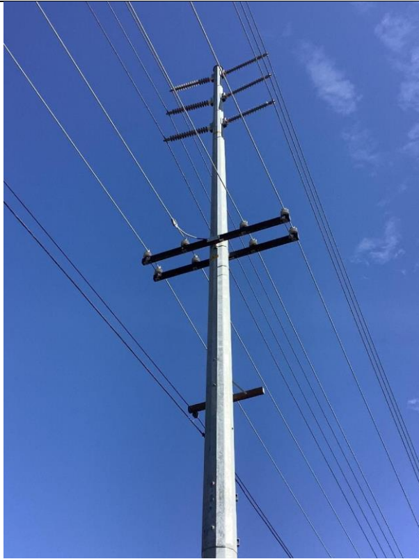
Item7GImg1: Overall pole
