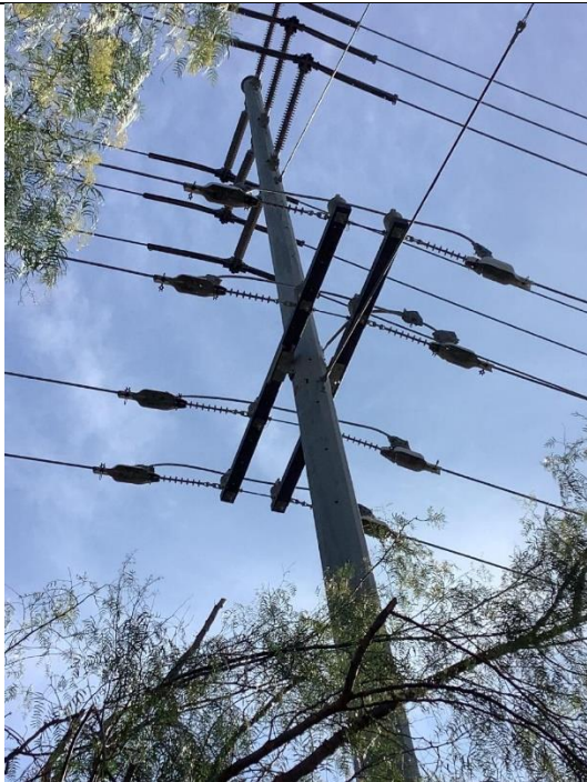
Item16IA1Img1: No vibration dampers installed
