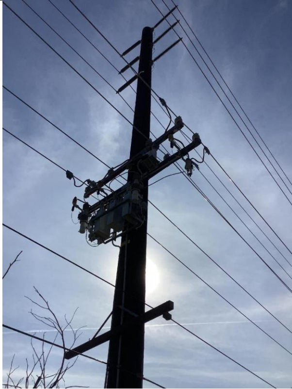
Item14GImg1: Overall pole
