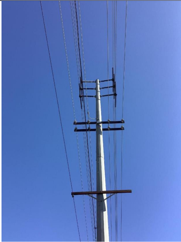
Item8GImg1: Overall pole
