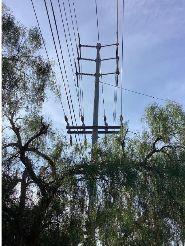
Item16GImg1: Overall pole
