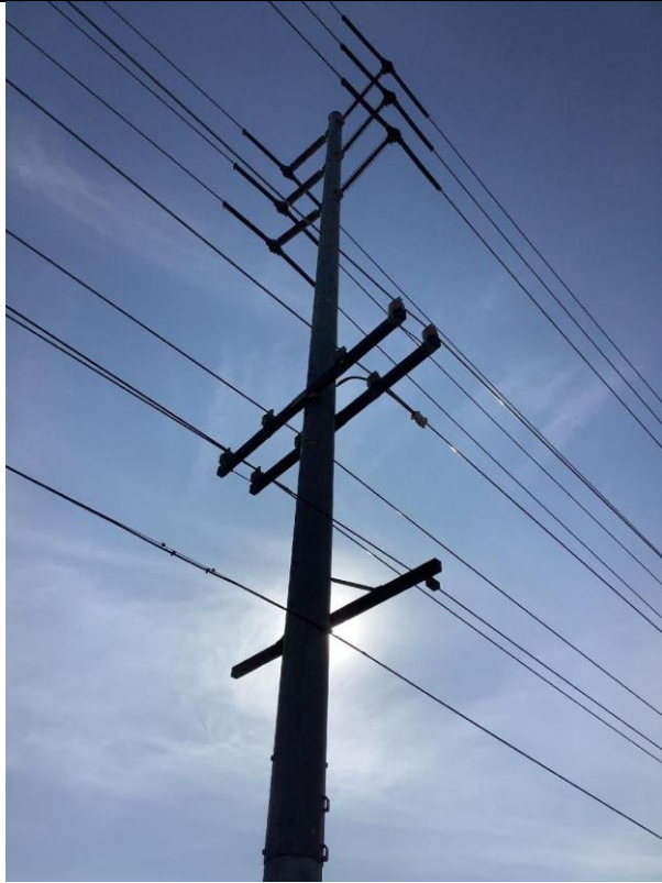
Item12GImg1: Overall pole
