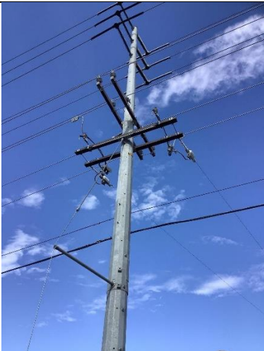
Item6IA1Img1: No vibration damper installed
