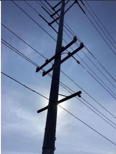
Item12IA1Img1: No vibration dampers installed
