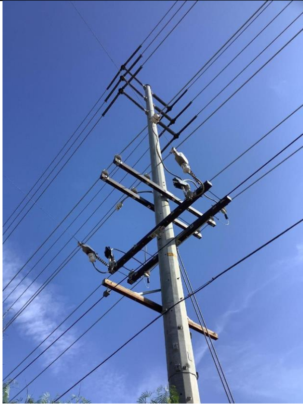
Item11GImg1: Overall pole
