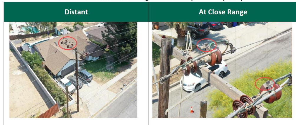
Distribution Switchblade Alignment Issue (Drone Capture)
