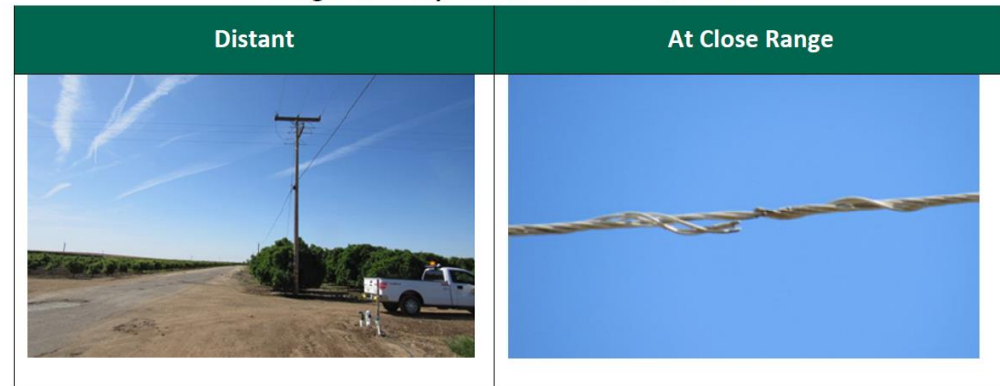
Damaged Primary Conductor on a 12kV Circuit
