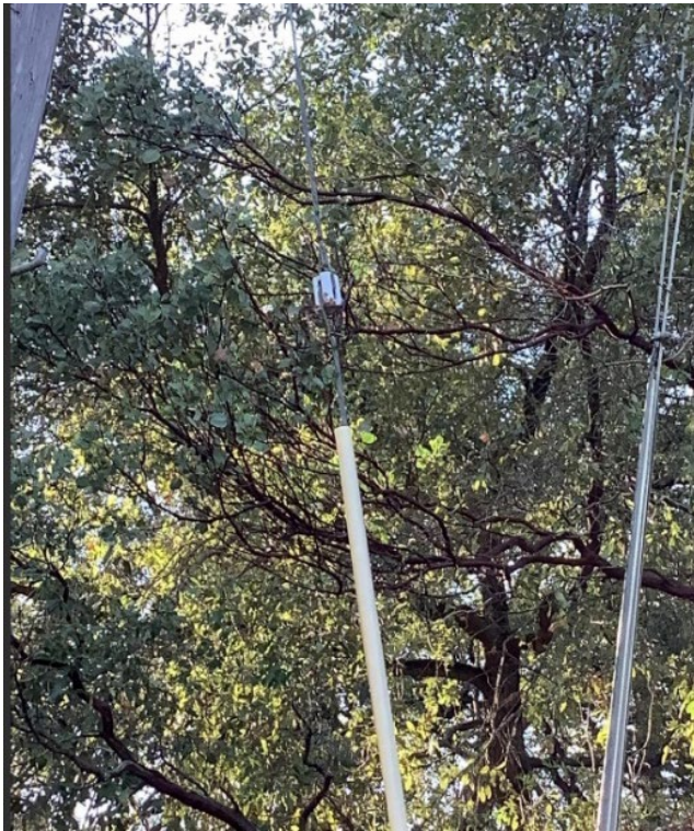
Photo 3: Picture of vegetation contacting the guy wire
