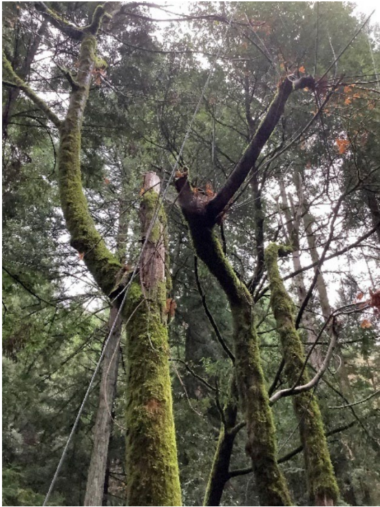
Photo 3: Picture of vegetation contacting the guy wire
