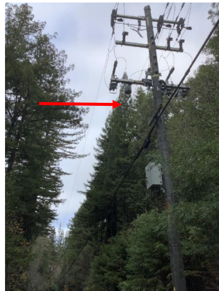
Photo 4: Picture of the primary conductors showing the middle phase conductor with four splices.
