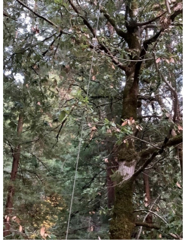
Photo 3: Picture of vegetation contacting the guy wire
