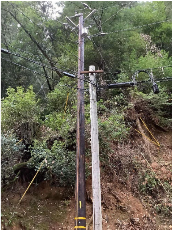
Photo 2: Picture of the entire Pole
