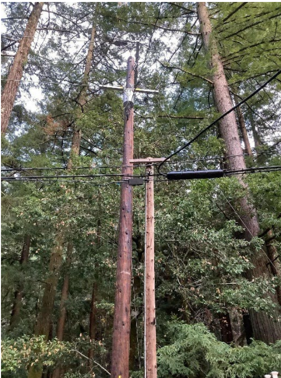
Photo 2: Picture of the entire Pole
