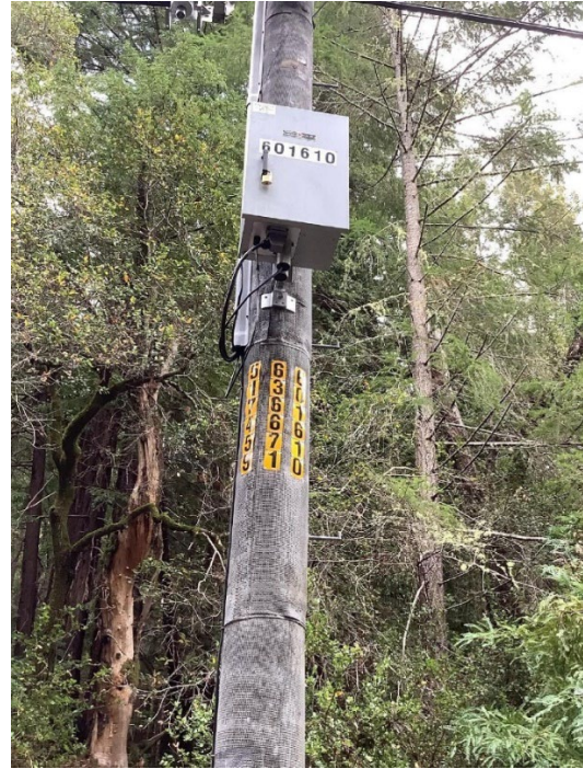
Photo 3: Line Recloser viper #601610
