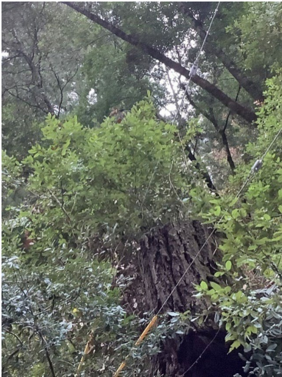
Photo 3: Picture of vegetation contacting the guy wire
