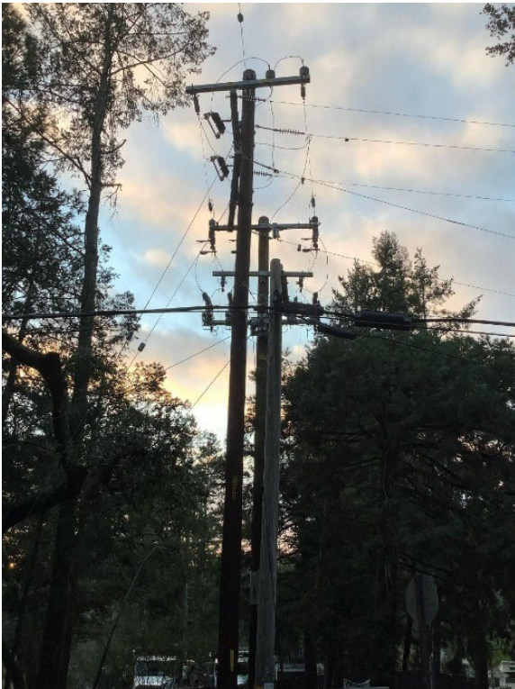
Photo 2: Picture of the entire Pole
