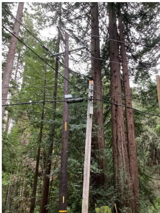
Photo 2: Picture of the entire Pole
