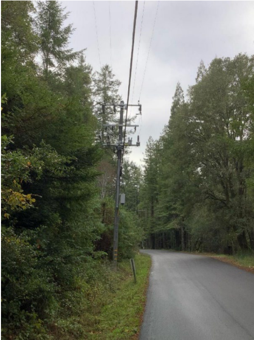
Photo 1: Picture of the entire pole
