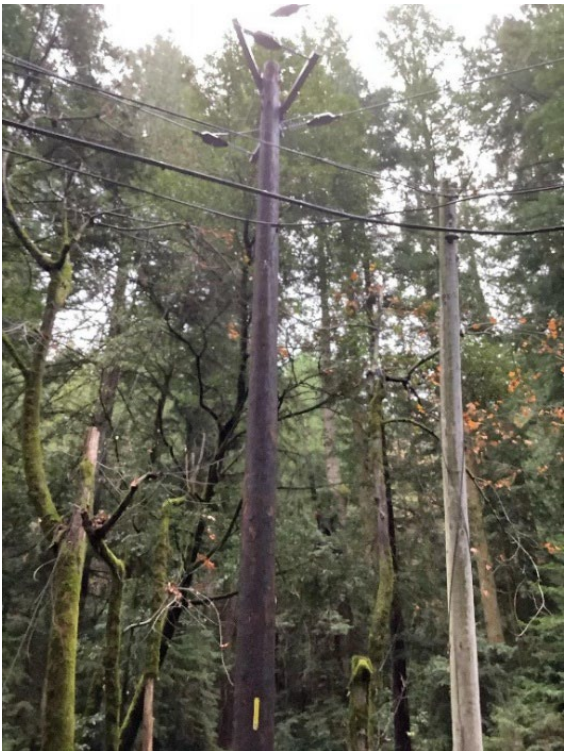
Photo 2: Picture of the entire Pole
