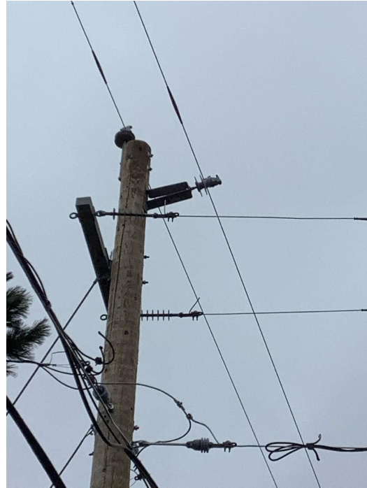
Item5CD6Img2: Conductor not secured
