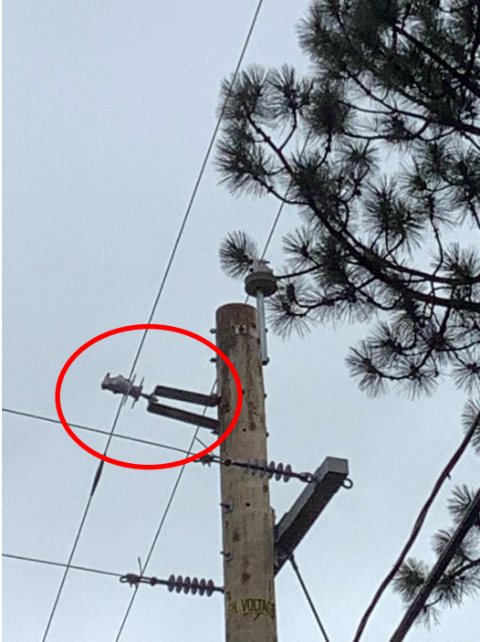
Item5CD6Img1: Conductor not secured
