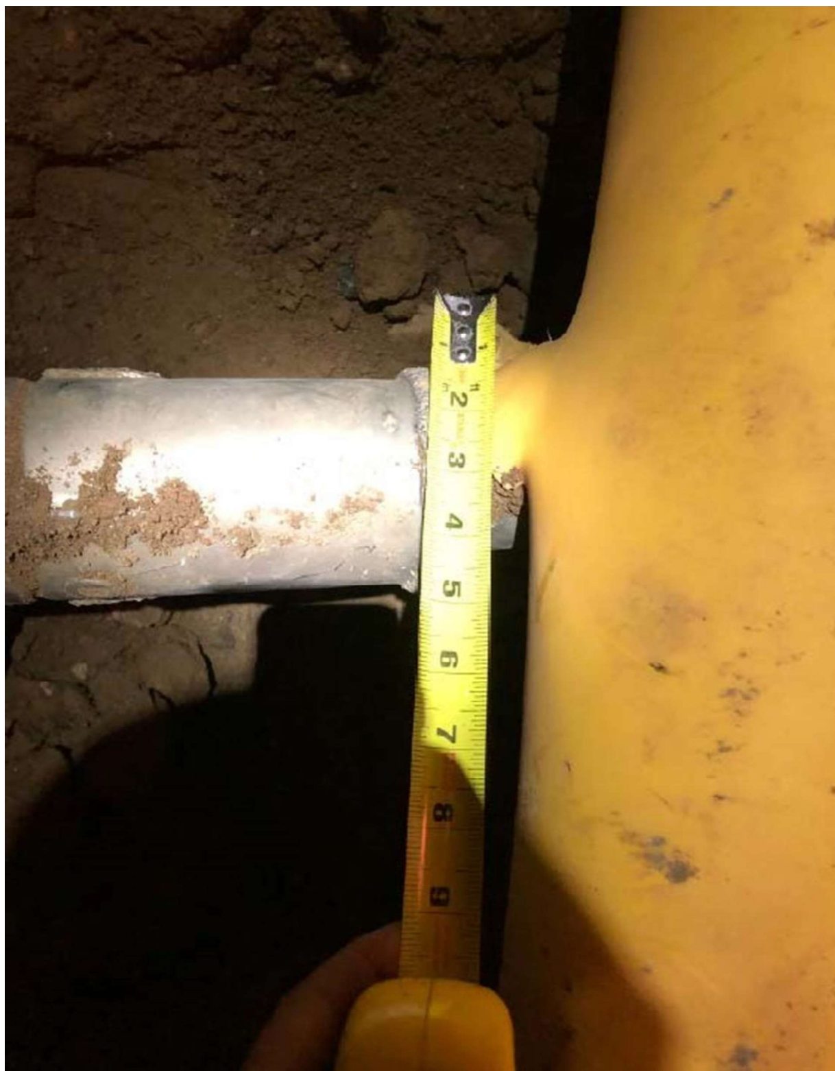
Photo 8: Drill penetrated the pipe
