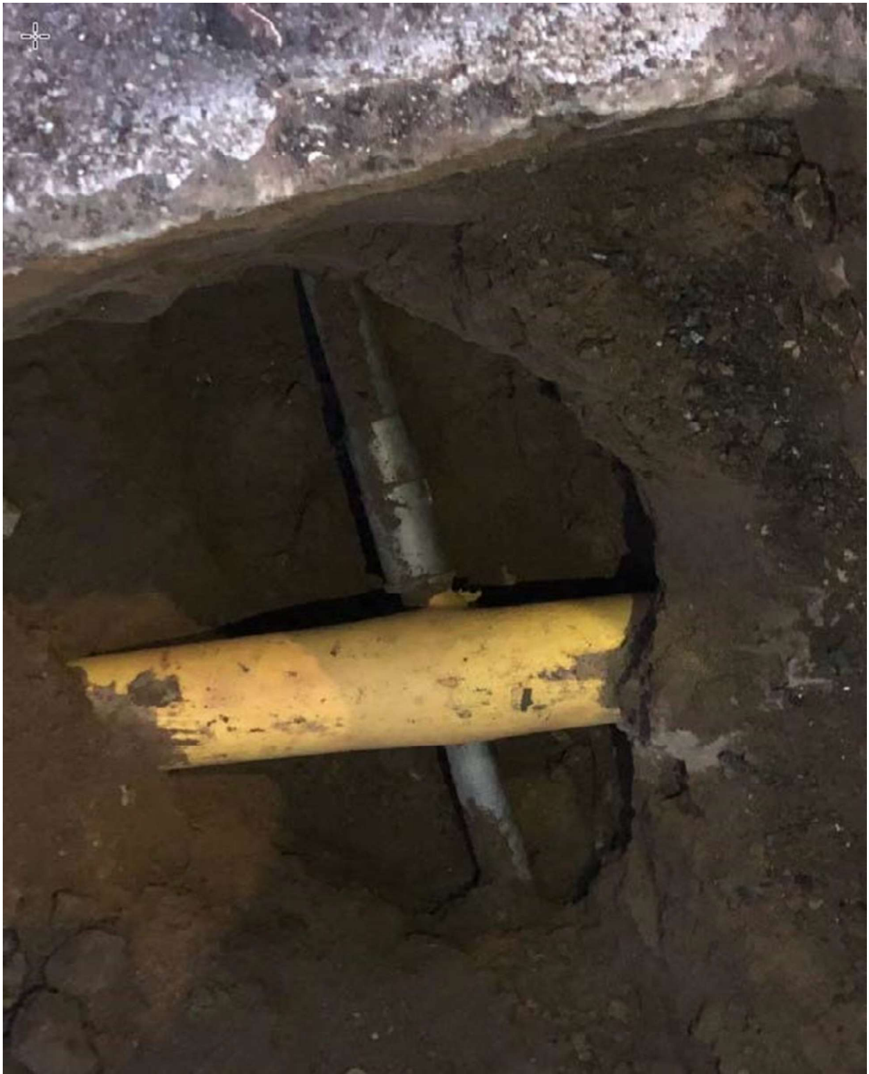
Photo 6: Directional Drill bored through the six-inch gas main
