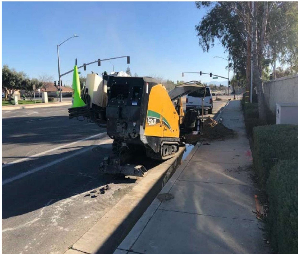
Photo 5: Directional Drill made contact with six-inch gas main
