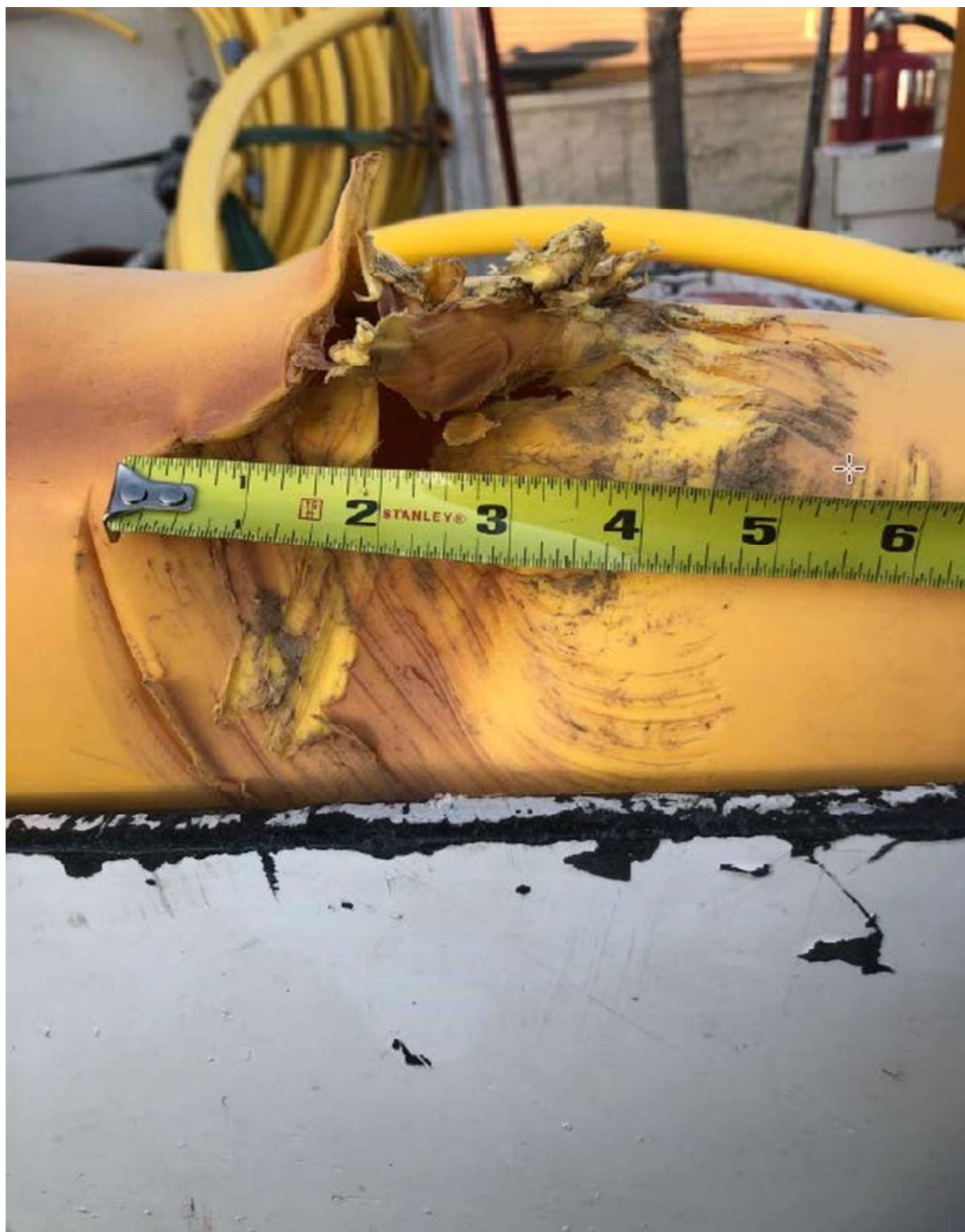
Photo 9: Damaged six-inch plastic gas main
