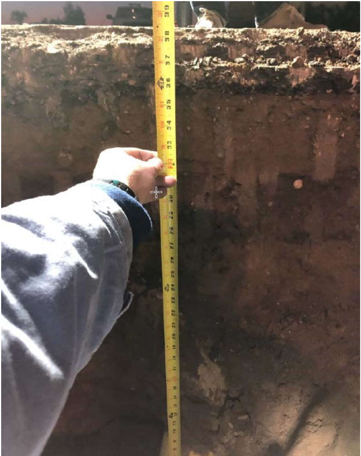
Photo 7: Damaged gas main located approximately 38.5 inches below ground surface
