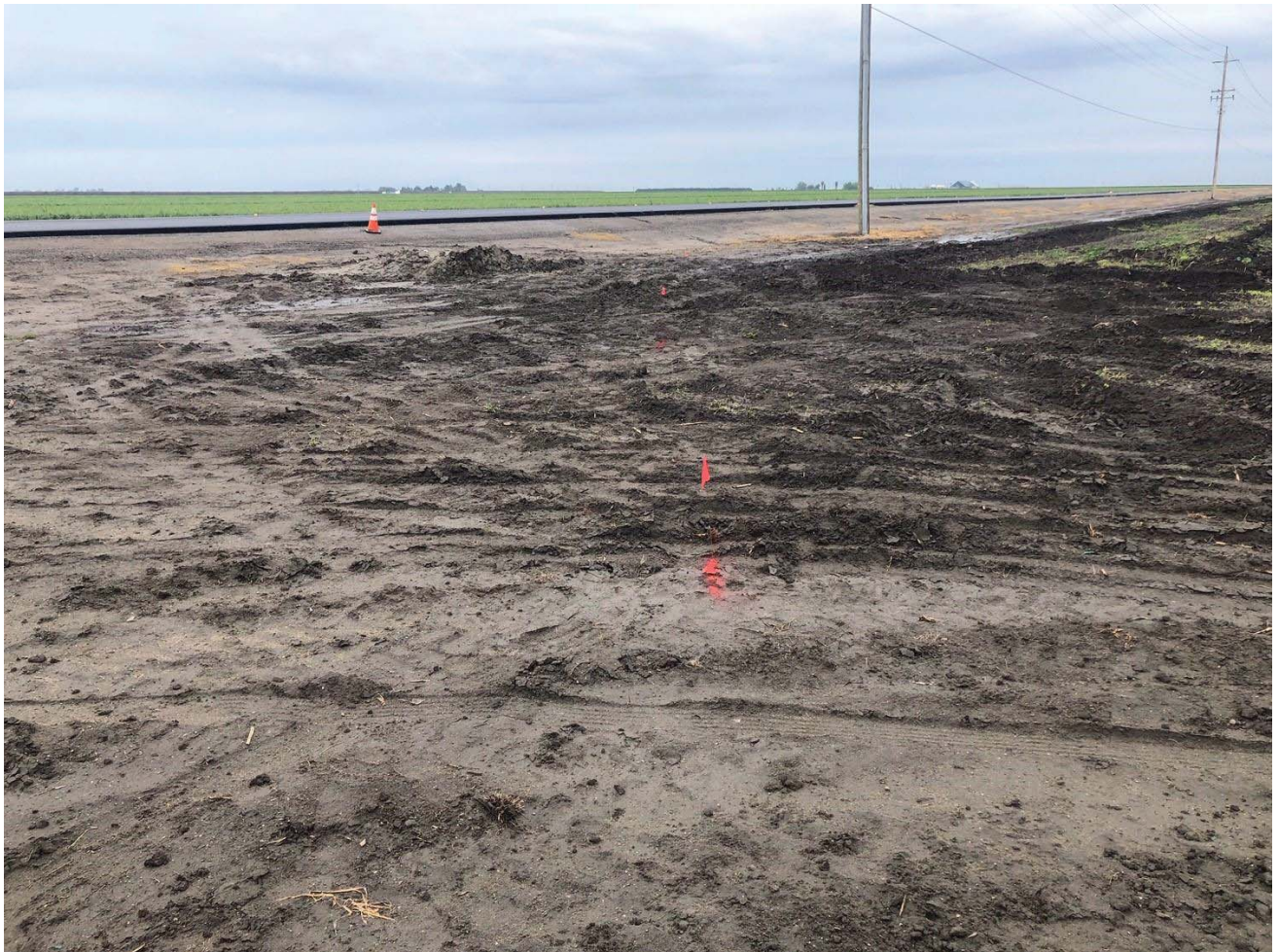
Photo: site of repaired line and new markings. Provided by Mr. Kincaid.
