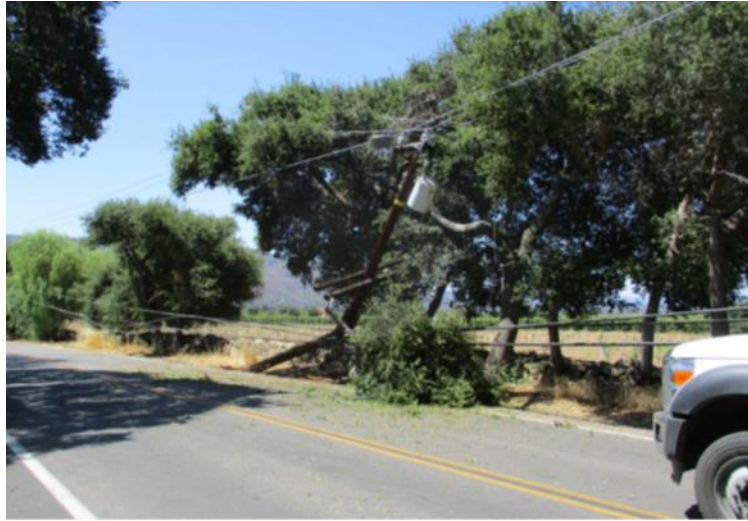
FIGURE PG&E-REMEDY-21-09-10: COVERED CONDUCTOR CONTACT WITH VEGETATION AFTER CAR HIT POLE OJAI, CALIFORNIA – JULY 24, 2020
