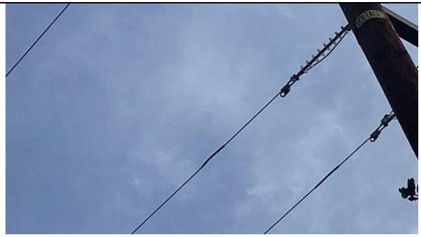
Item1IA1Img2: Close up of bare wire
