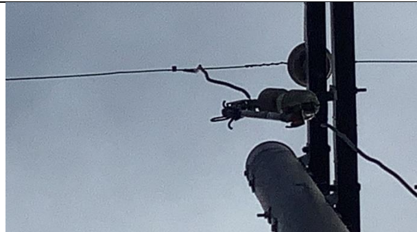
Item3IA1Img2: Close up of bare wire
