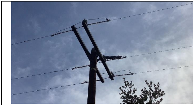
Item1IA1Img1: No covered conductor
