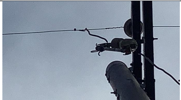
Item3IA1Img2: Close up of bare wire
