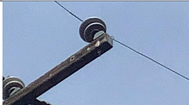
Item2IA1Img2: Bare wire closeup
