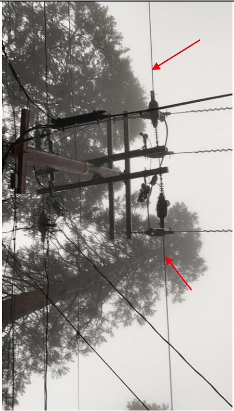
Item3IA1mg1: No vibration dampers on span (see red arrow)
