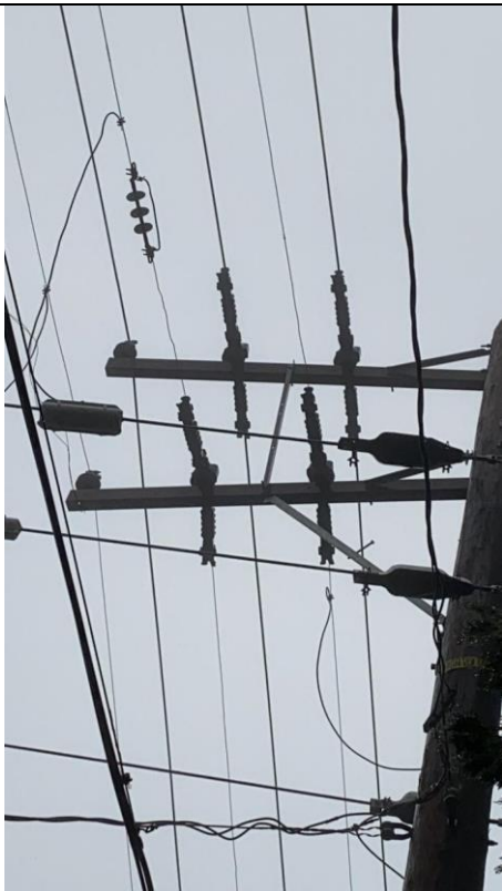
Item1IA1Img1: Top level crossing phase showing bare wire and no covered conductor installed
