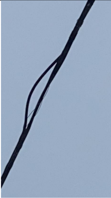
Item9CD4Img1: Broken support strand
