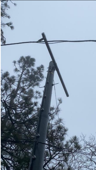
Item10IA1Img1: No covered conductor installed
