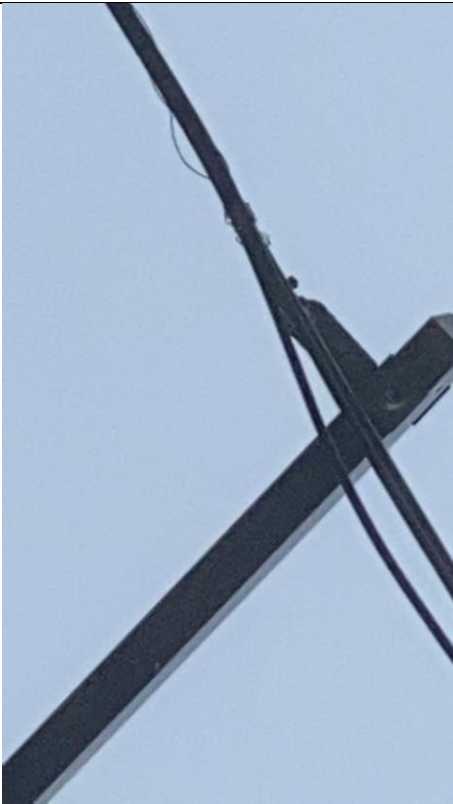
Item10CD4Img1: Fraying conductor
