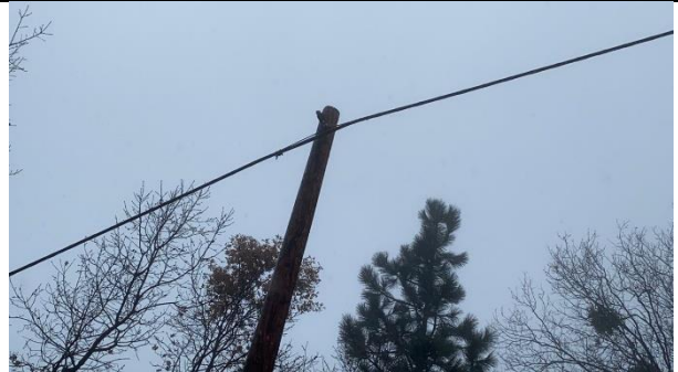
Item9IA1mg2: Zoomed out view of top of pole with no covered conductor
