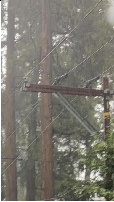
Item5IA1Img1: No vibration dampers
