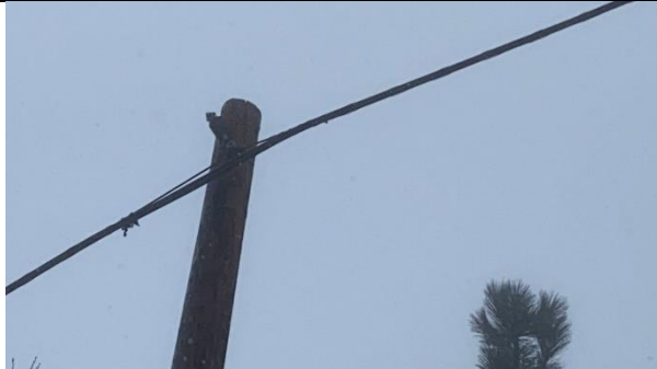
Item9IA1mg1: Close up no covered conductor
