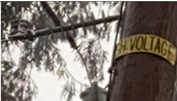
Item3IA5Img1: Bare jumper going into bolted wedge connector cover
