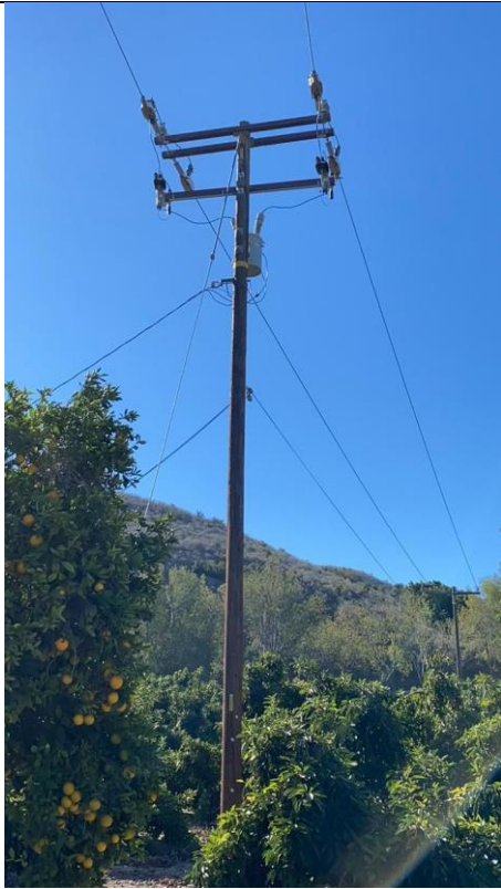
Item8GImg1: Overall pole
