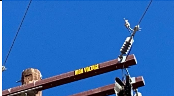
Item13IA1mg2: Bare wire to covered conductor close up
