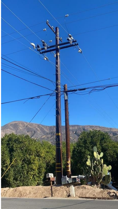
Item14GImg1: Overall pole
