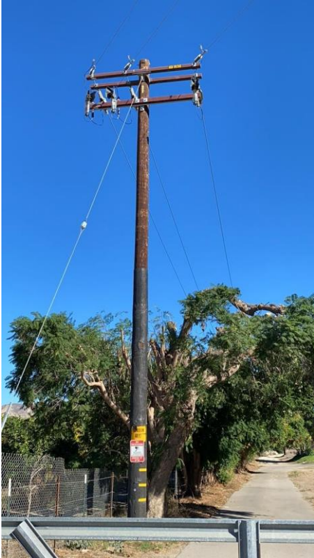
Item13G1mg1: Overall pole
