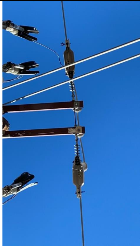
Item1IA1img2: Close up, no vibration dampers installed
