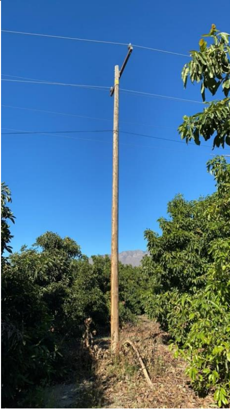
Item9GImg1: Overall pole
