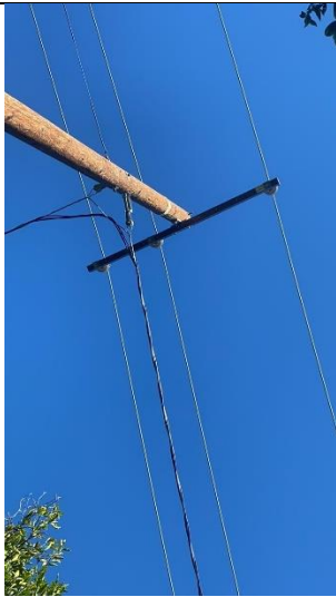
Item15IA1img1: Vibration dampers not installed
