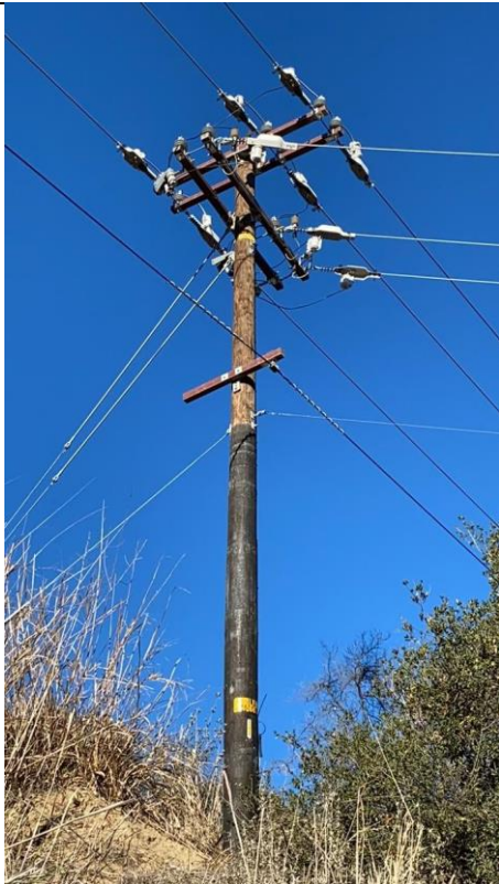
Item1GImg1: Overall pole
