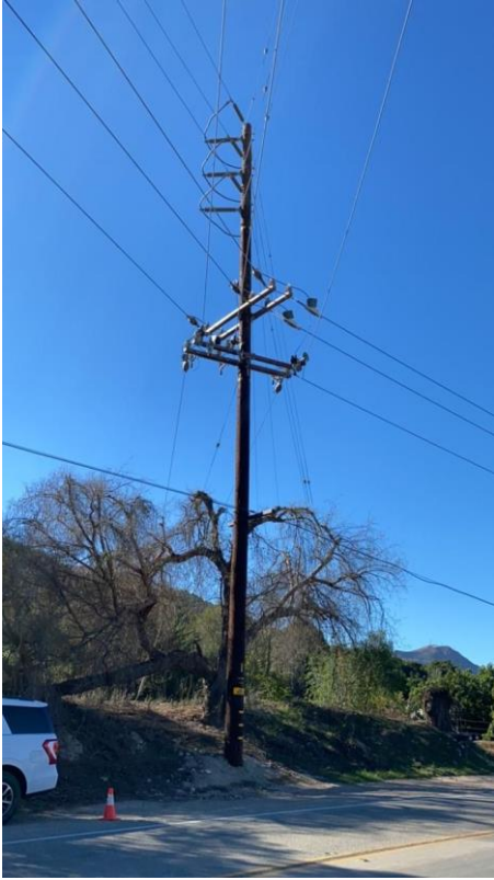
Item7GImg1: Overall pole
