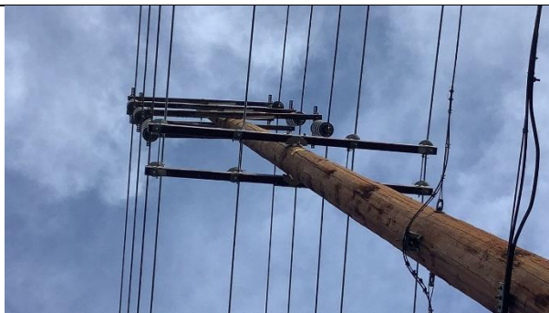
Item4IA1img1: Vibration dampers not installed
