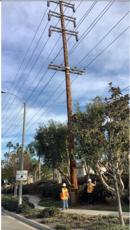
Item9GImg1: Overall pole
