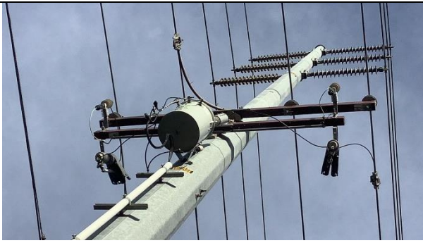
Item8IA1Img1: No vibration dampers installed
