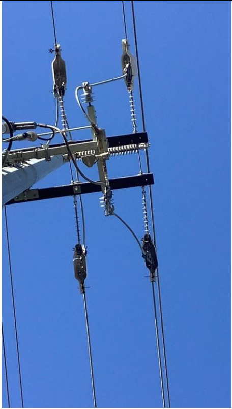
Item1IA1mg3: Close up of one phase showing no vibration dampers
