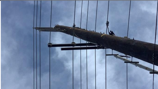
Item5IA1Img1: Vibration dampers not installed
