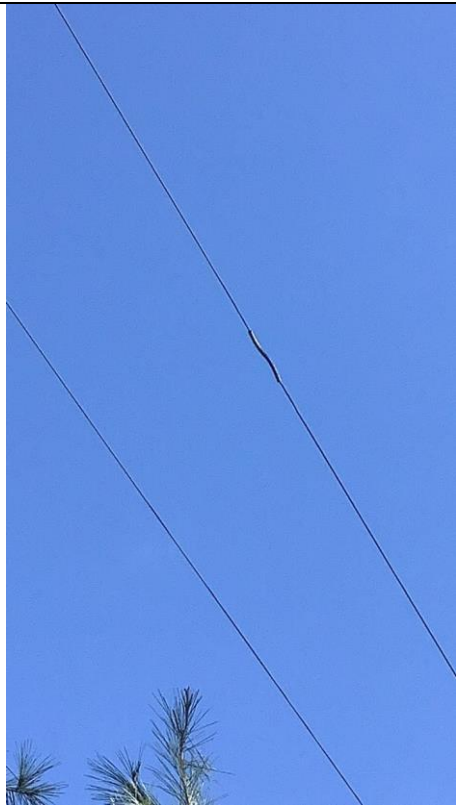
Item7CD9Img2: Third splice on same phase
