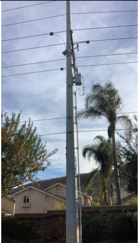
Item8GImg1: Overall pole
