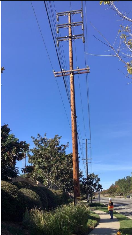
Item4GImg1: Overall Pole
