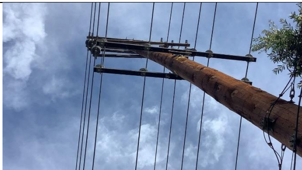
Item9IA1Img1: Vibration dampers not installed
