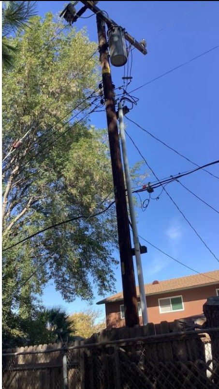
Item7GImg1: Overall pole
